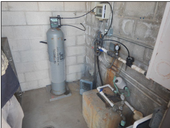
Photograph #11 (DSCN9141) Description: View of the chlorine feed system inside the Facility's out-building.
