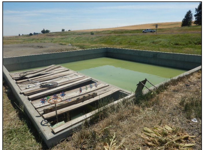
Photograph #12 (DSCN9151) Description: View of the Facility's disinfection unit.
