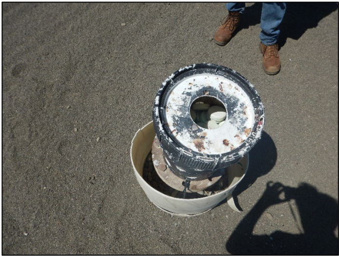
Photograph #17 (DSCN9156) Description: View of an improvised dechlorination unit at one of the Facility's sand filters.
