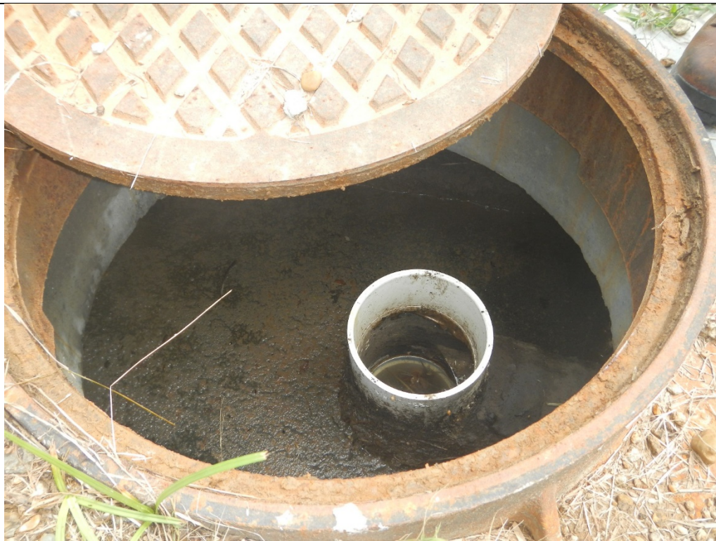
Photo 5 Oil and grease separator 2
