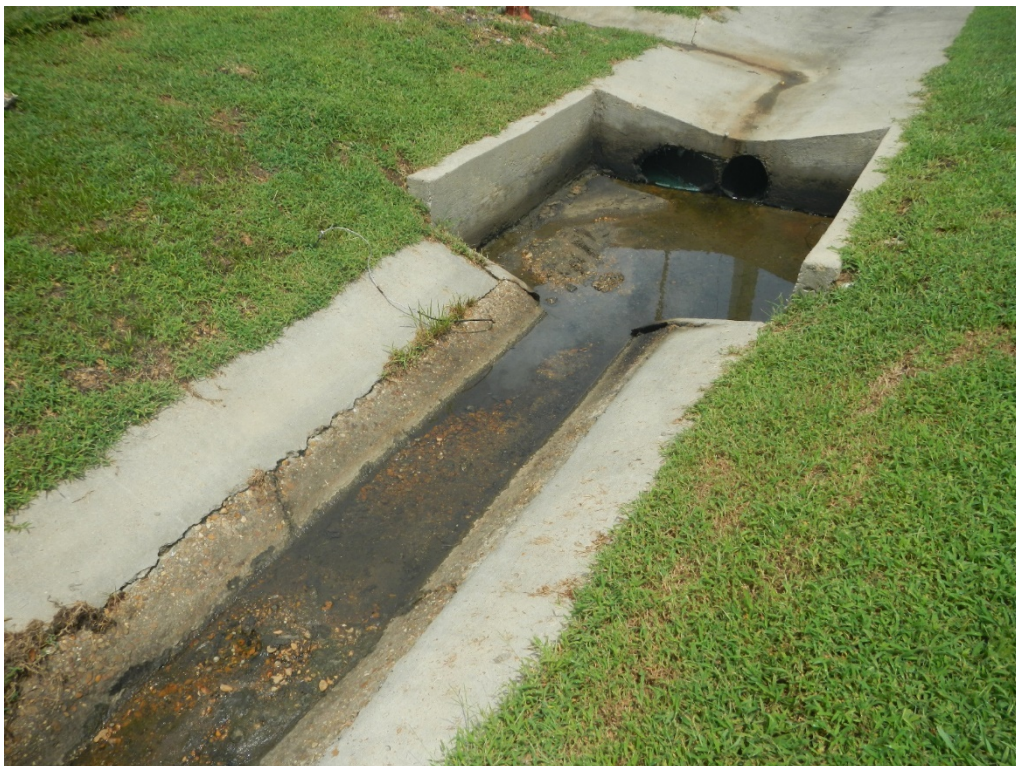
Photo 4 Actual location of discharge for outfall 001
