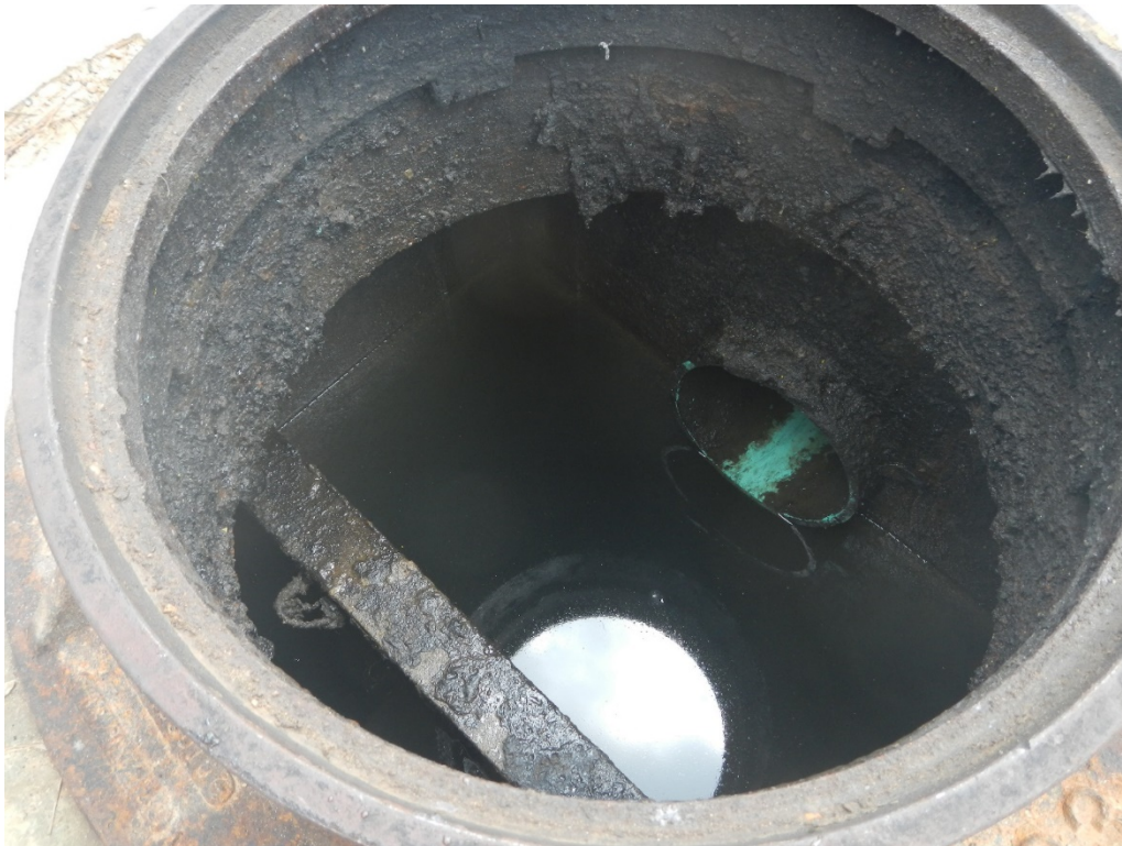
Photo 2 Influent pipe for oil and grease separator 1
