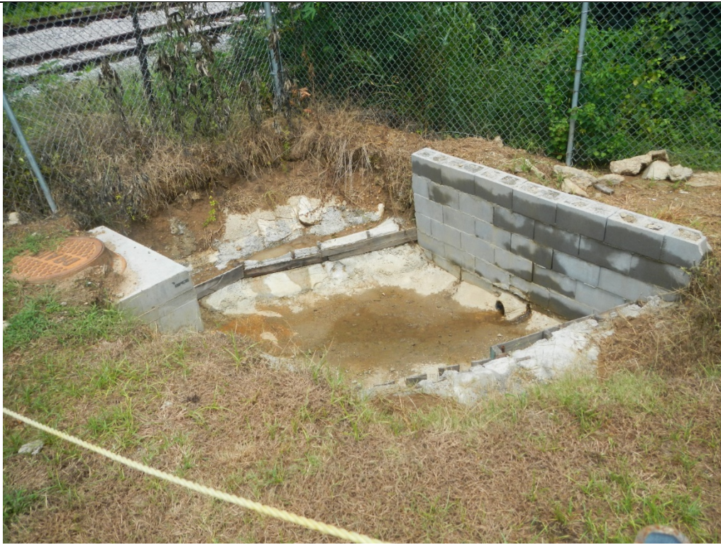
Photo 7 Water storage after oil and grease separator and before outfall.
