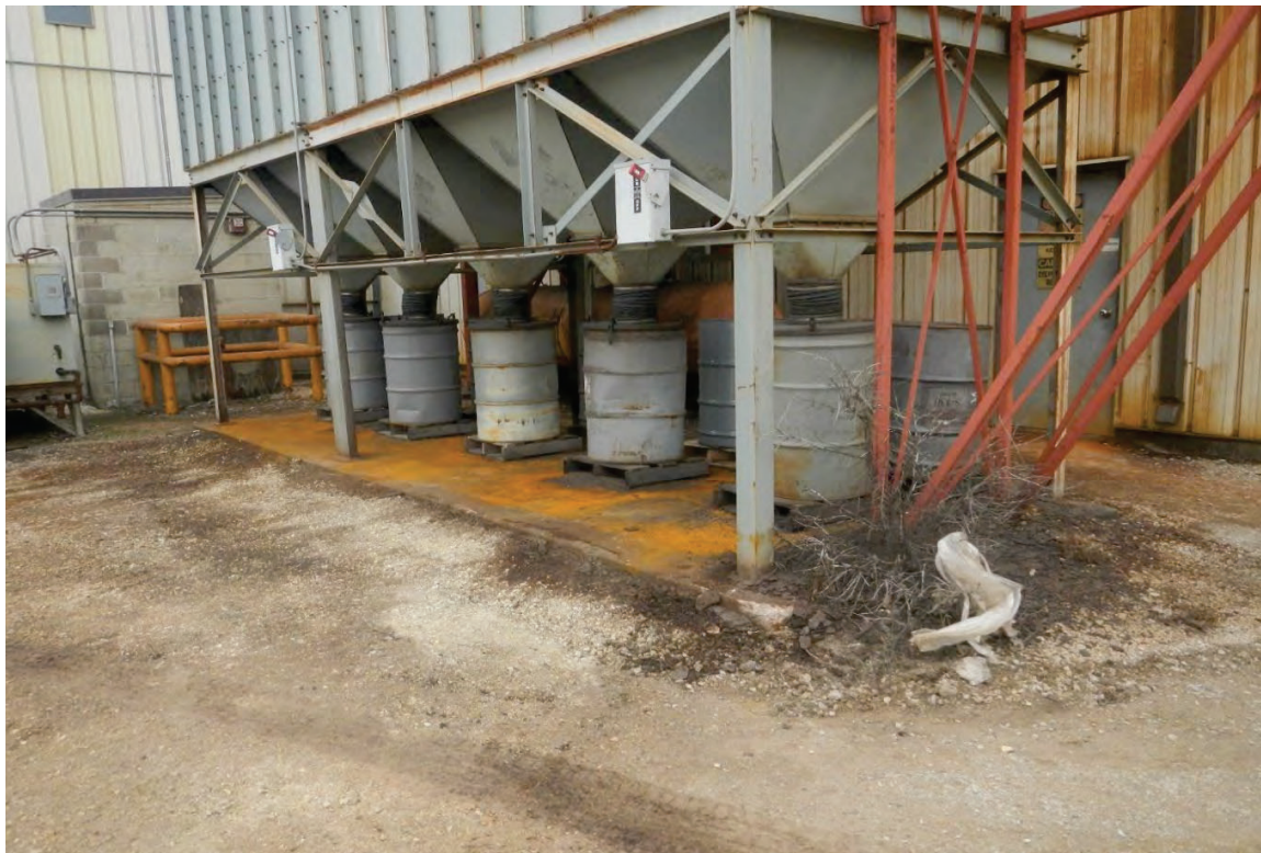
Photo 15, Ground discoloration from the collection system
