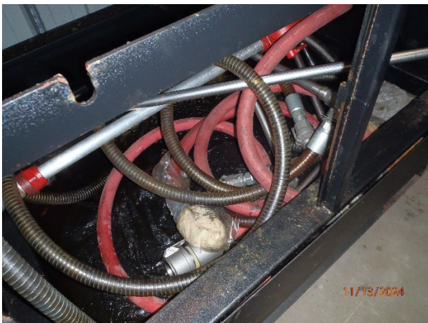
Picture 21 – Spinning Maintenance lube oil station drain pan full of used oil
