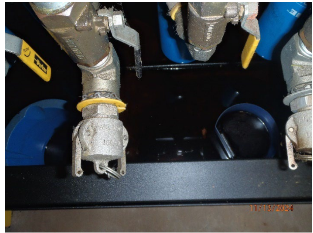
Picture 22 – Spinning Maintenance lube oil station drain pan full of used oil
