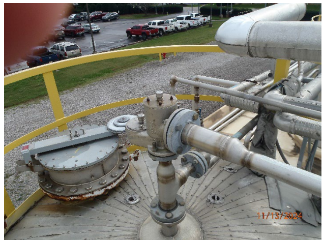
Picture 49 – AN Waste Tanks top of the tank piping
