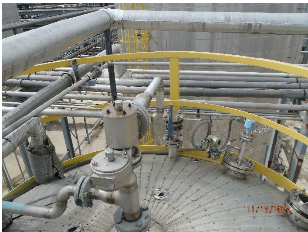
Picture 48 – AN Waste Tanks top of the tank piping
