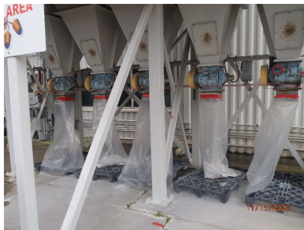
Picture 43 – Thermal Oxidizer Baghouse dust
