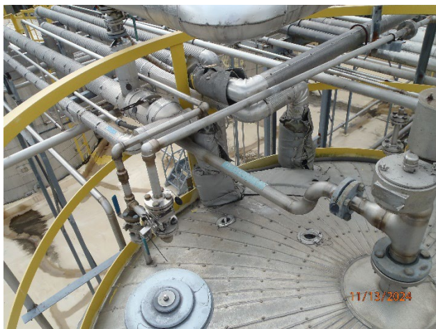
Picture 47 – AN Waste Tanks top of the tank piping
