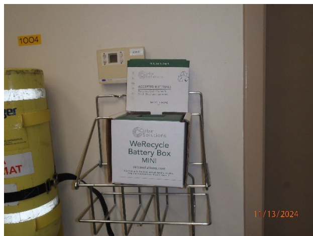
Picture 6 – Carbonization Line 1 UW Battery box need label
