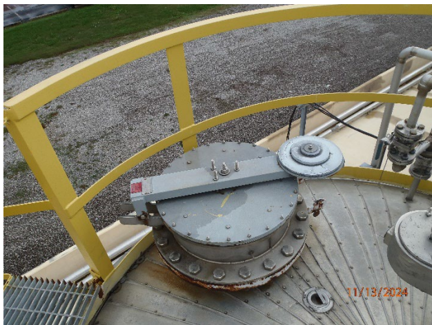
Picture 46 – AN Waste Tank conservation vent
