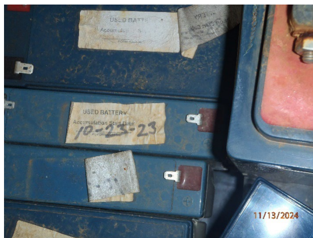
Picture 30 – UWSA spent lead acid battery labels – exceeded the storage date
