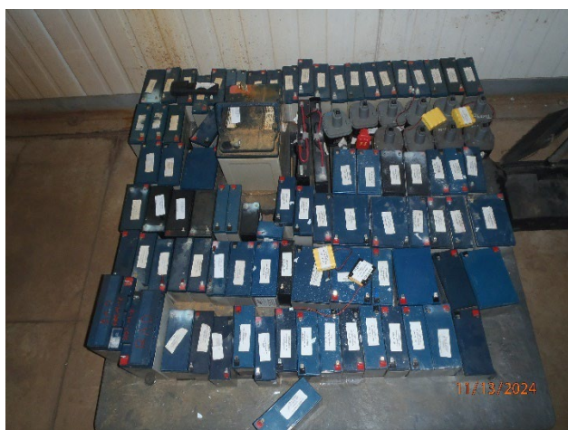
Picture 27 – UWSA spent lead acid batteries
