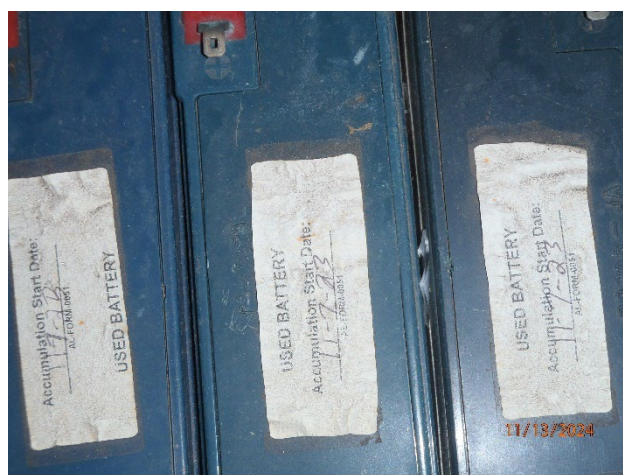
Picture 29 – UWSA spent lead acid battery labels – exceeded the storage date
