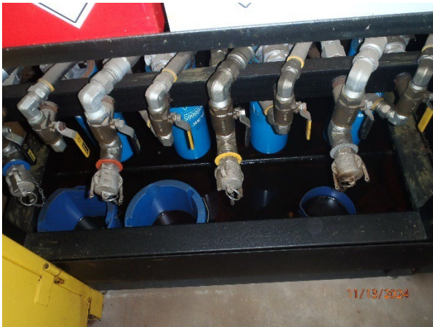
Picture 20 – Spinning Maintenance lube oil station drain pan full of used oil
