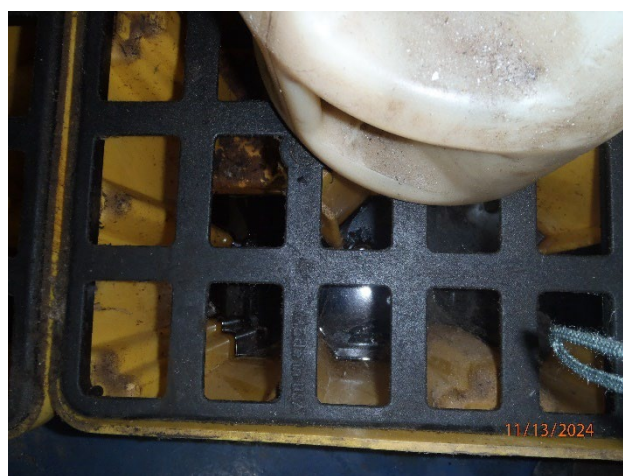
Picture 5 – CARB Used Oil secondary containment need clean out
