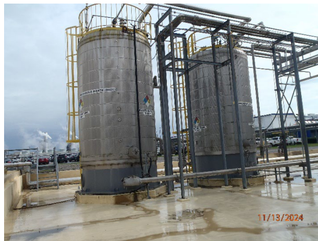
Picture 45 – AN Waste Tanks
