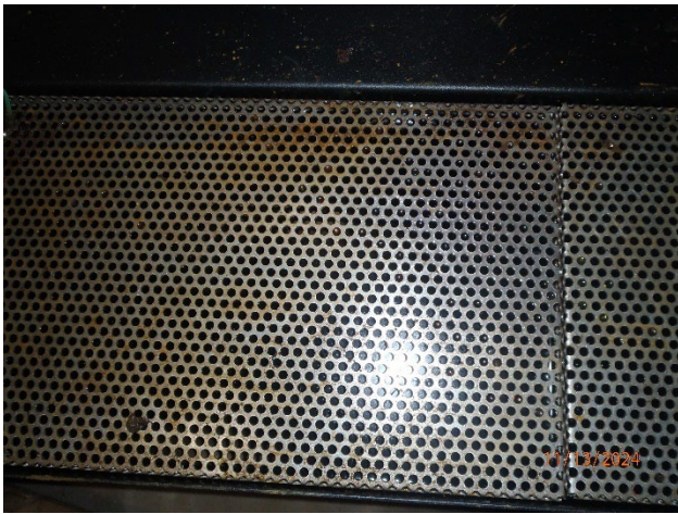
Picture 19 – Spinning Maintenance lube oil station drain pan full of used oil
