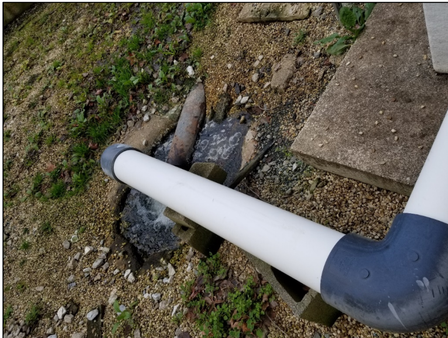
Photograph 10. View of the effluent discharge location, upstream of Outfall 001. Note the pipe in the ground is below grade and the surrounding area is mostly dirt and gravel.
