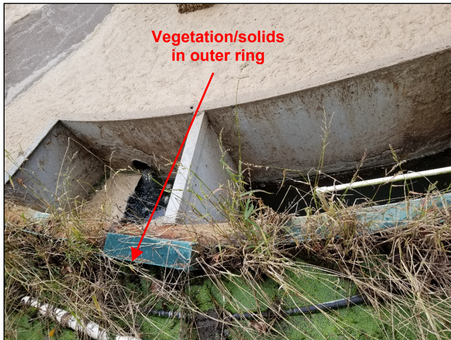
Photograph 6. View of vegetation/solids in the outer ring of the Plant. Note that this area could be used for additional capacity or emergency storage.
