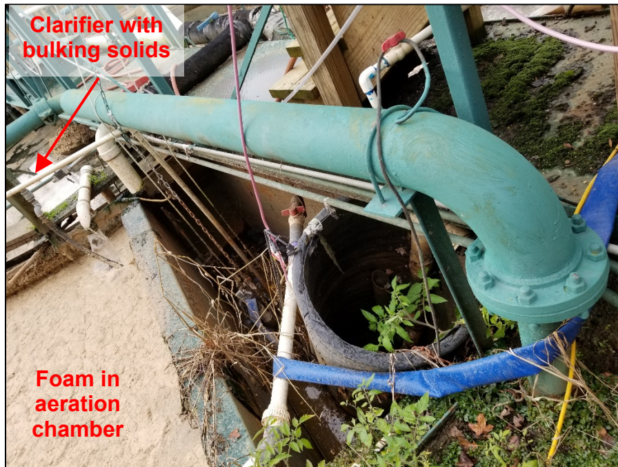
Photograph 4. Additional view of the aeration chamber. Note the presence of foam. Also note the presence of bulking solids in the clarifier.
