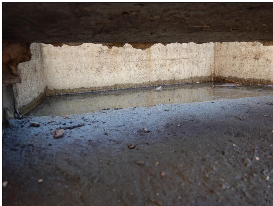
Photograph 12. View inside the inlet to the Meridian MS4 shown in Photograph 11 . Note the lack of inlet protection.
