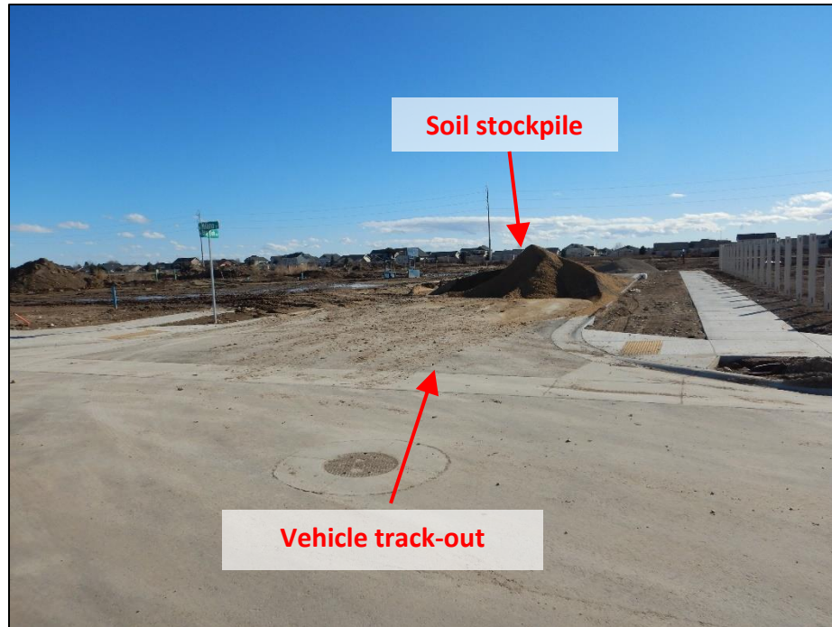
Photograph 1. View, facing south, of an unprotected stockpile on North Sunfield Road. Note the vehicle track-out in the foreground.
