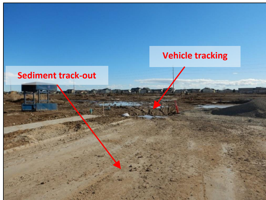
Photograph 6. Additional view, facing south, of unrestricted vehicle access and construction vehicle track-out on North Sunfield Road in Phase 4 as shown in Photograph 5 . Note no stabilization techniques had been implemented to prevent sediment track-out.
