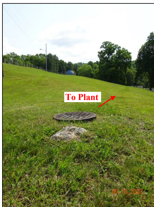
Photograph 4. View, facing east, of confluence manhole where wastewater from the boat pump-out and comfort station meet.
