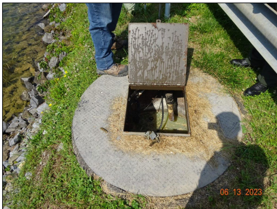
Photograph 2. View, facing west, of the lift station which pumps wastewater from the boat pump-out to the manhole behind the comfort station.
