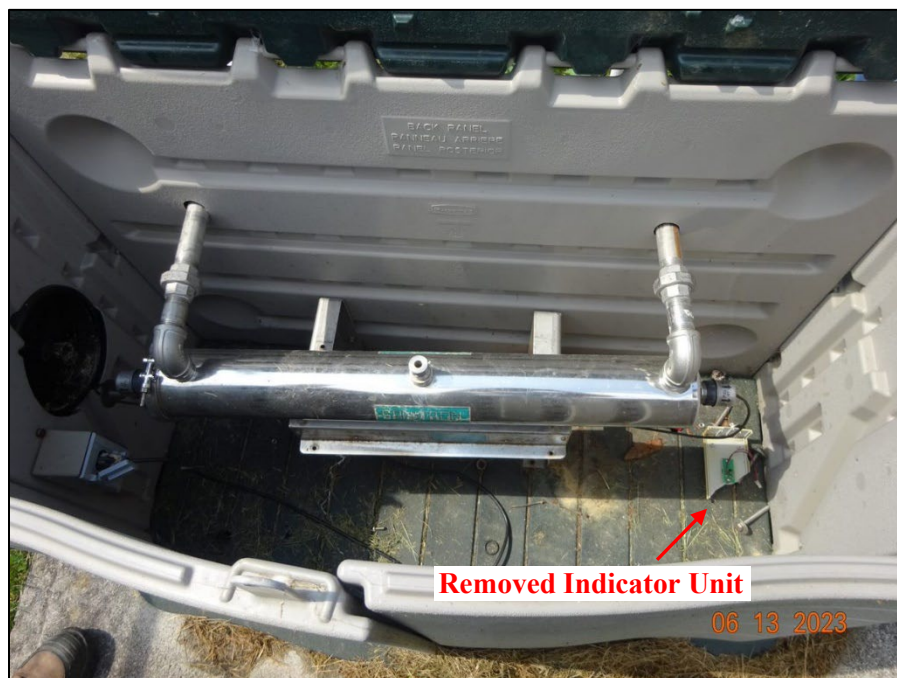
Photograph 11. View of the UV contact chamber inside its housing. Note debris and removed indicator unit on the floor of the housing.
