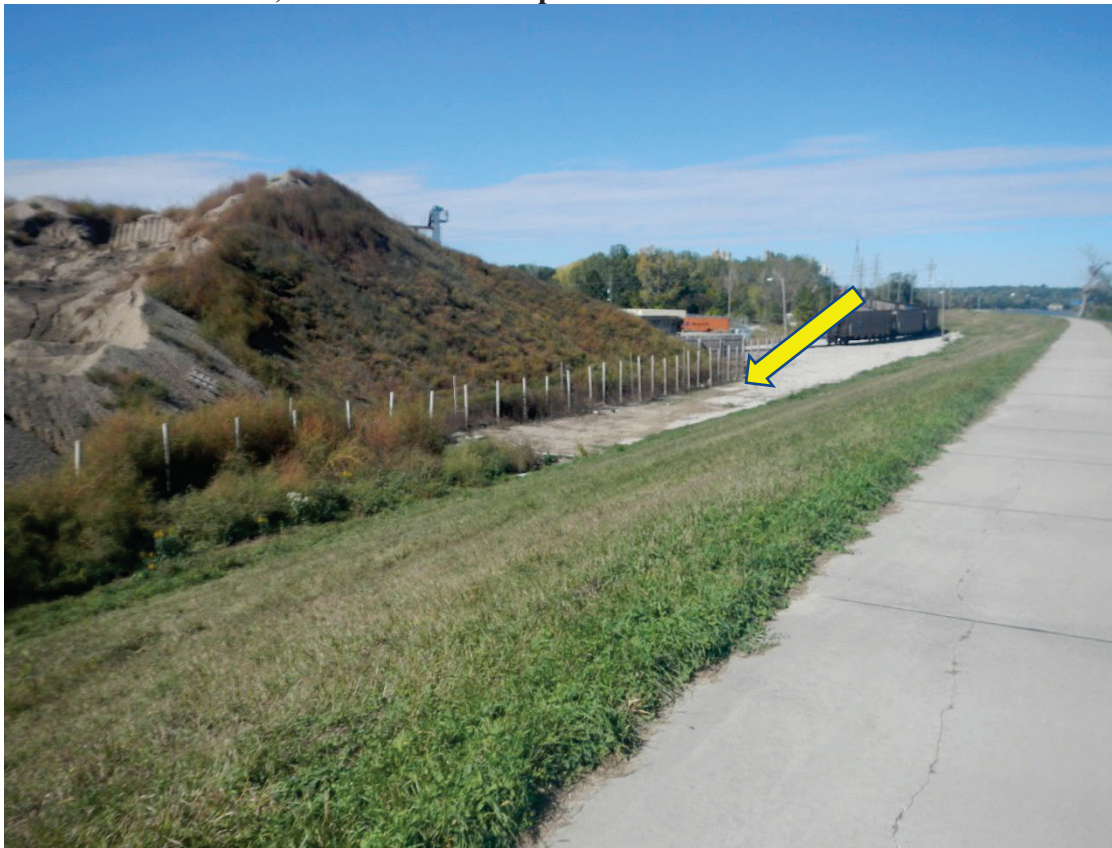
Photo 8, Process material spilled outside the north fence line.
