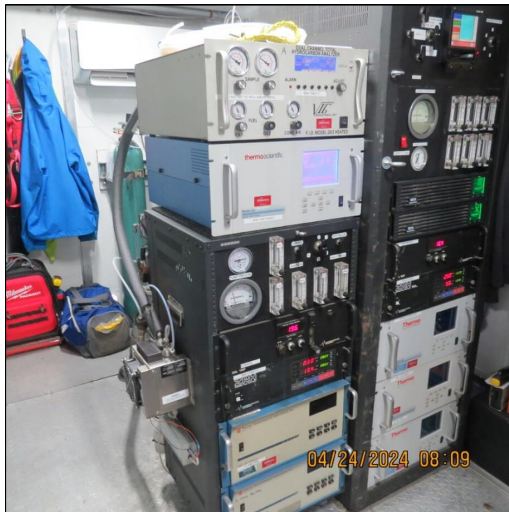
Photograph 3: Testing Trailer Analyzer Setup
