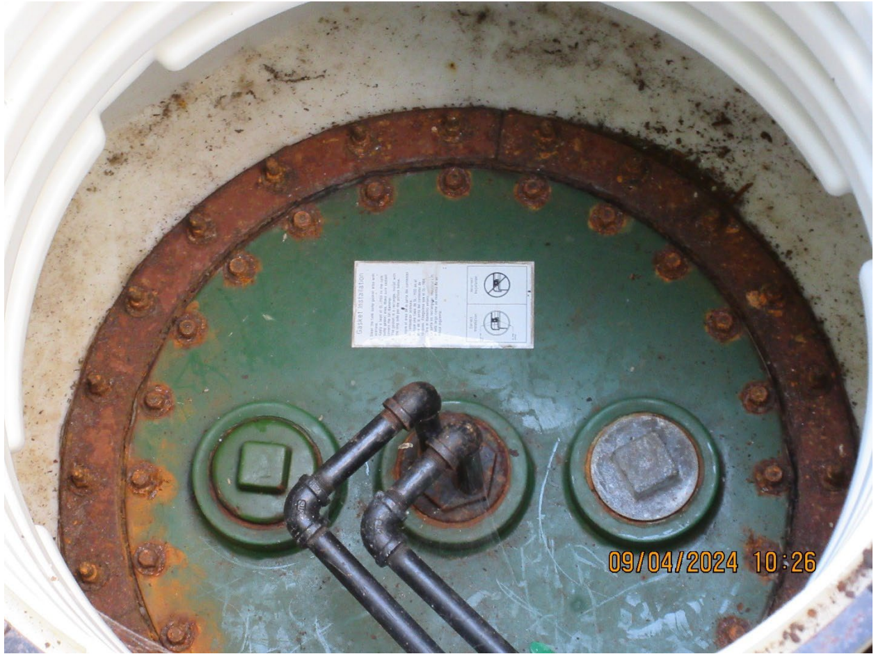
Photo 2 – Opened containment sump
