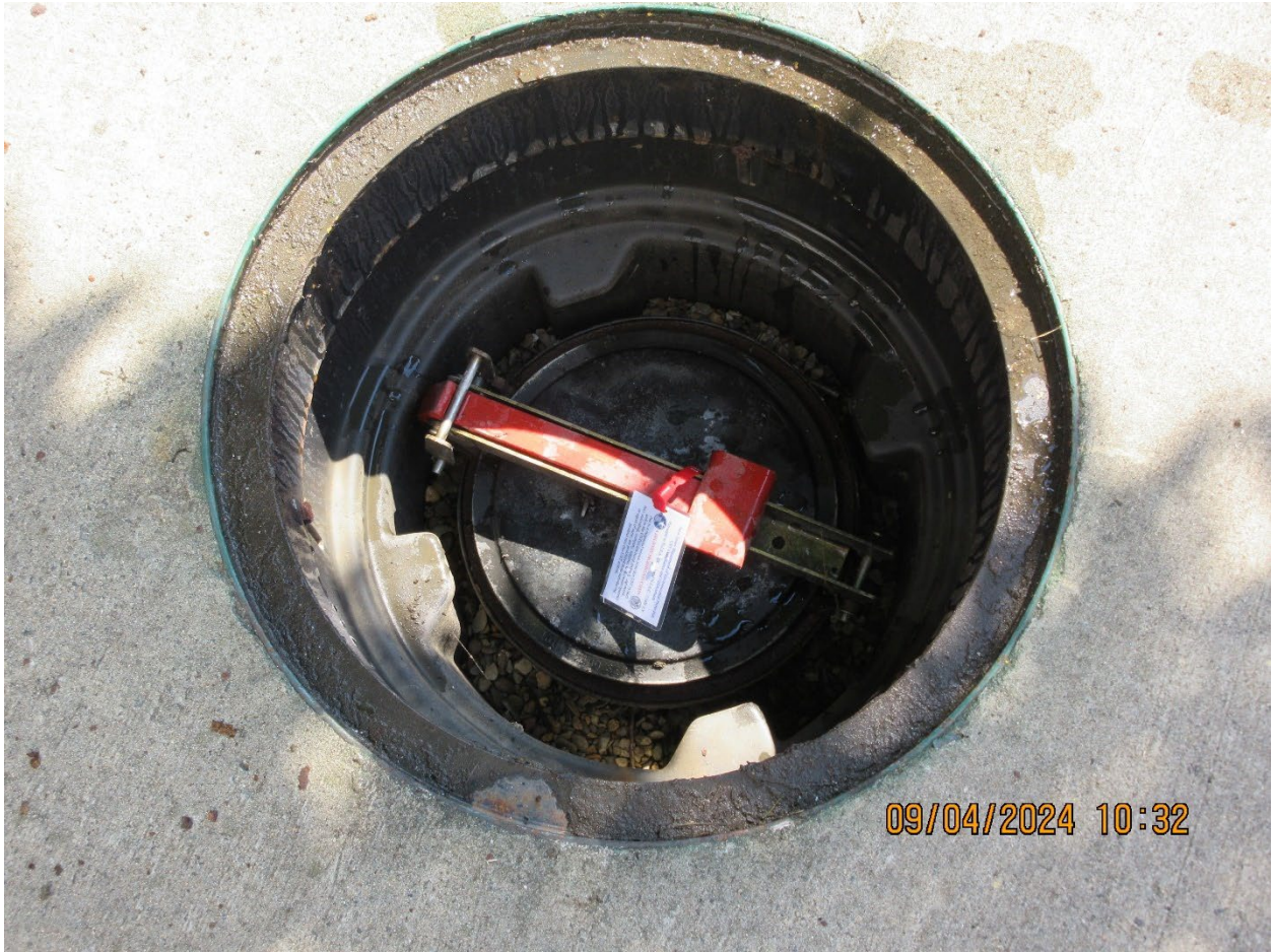
Photo 5 – Fill port and spill bucket
