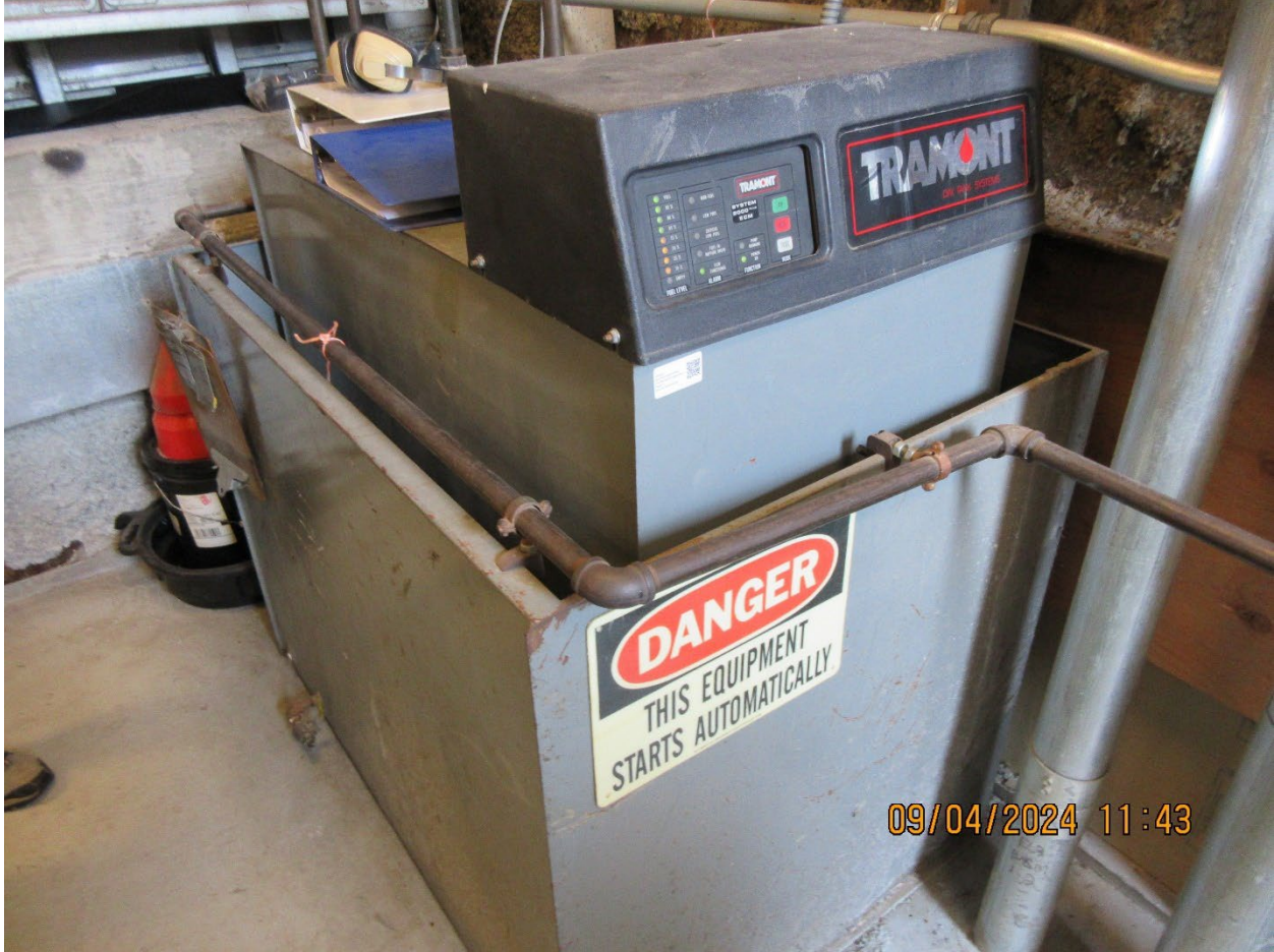
Photo 18 – Day tank with secondary containment
