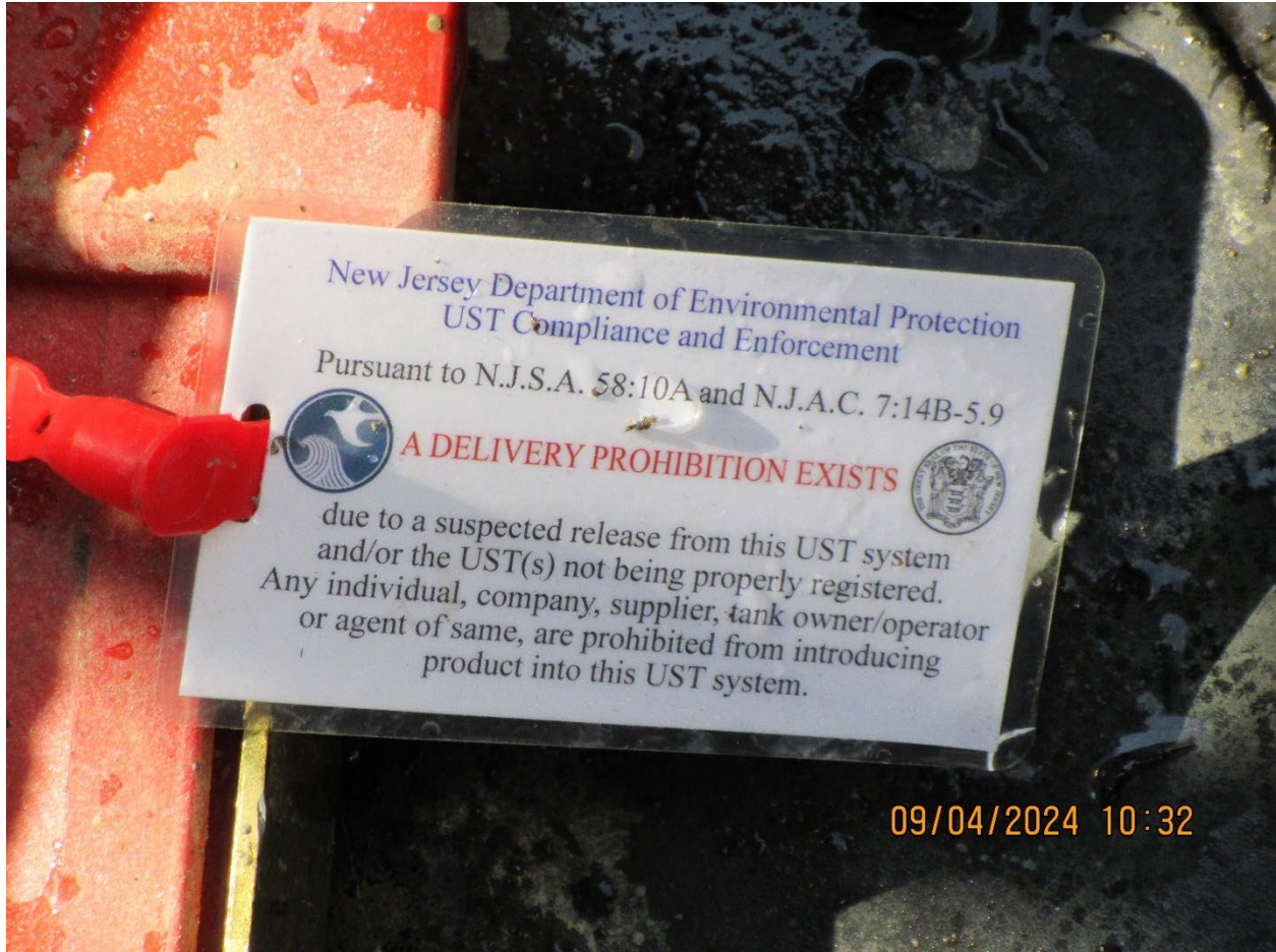
Photo 6 – NJDEP fuel delivery prohibition tag
