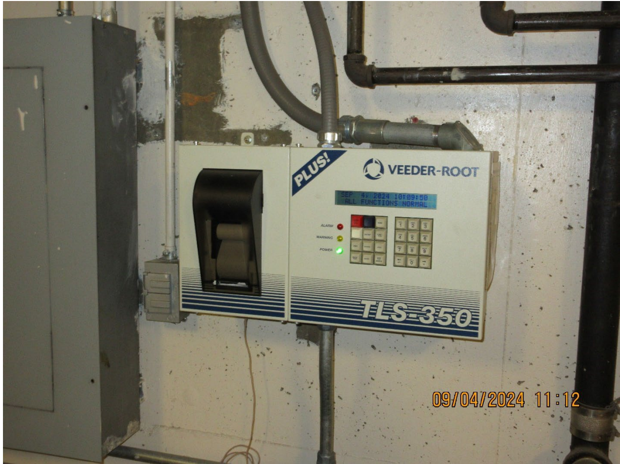
Photo 12 – Automatic tank gauge
