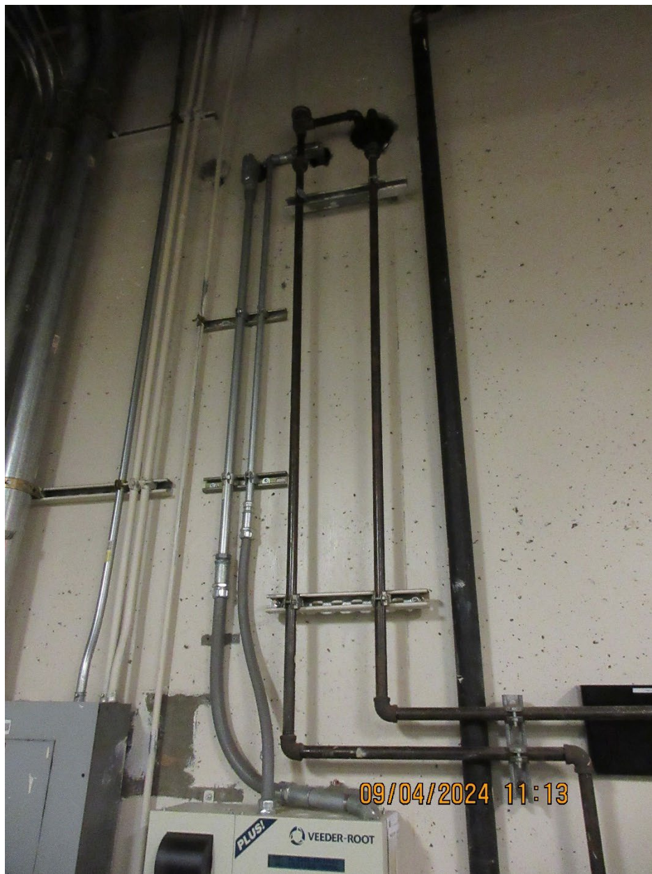
Photo 14 – Interior product pipes to pump
