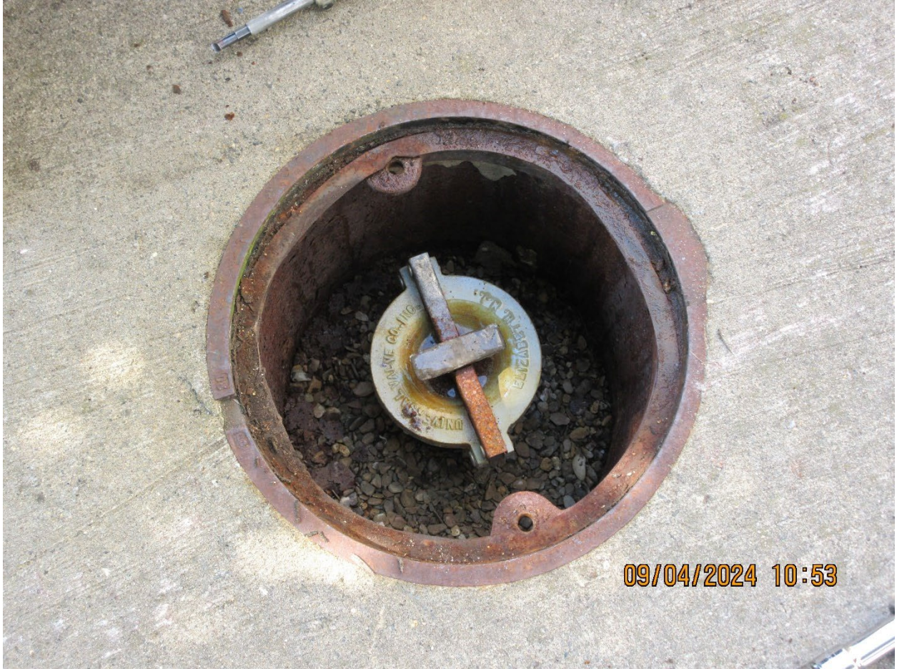
Photo 9 – Access port for pipe
