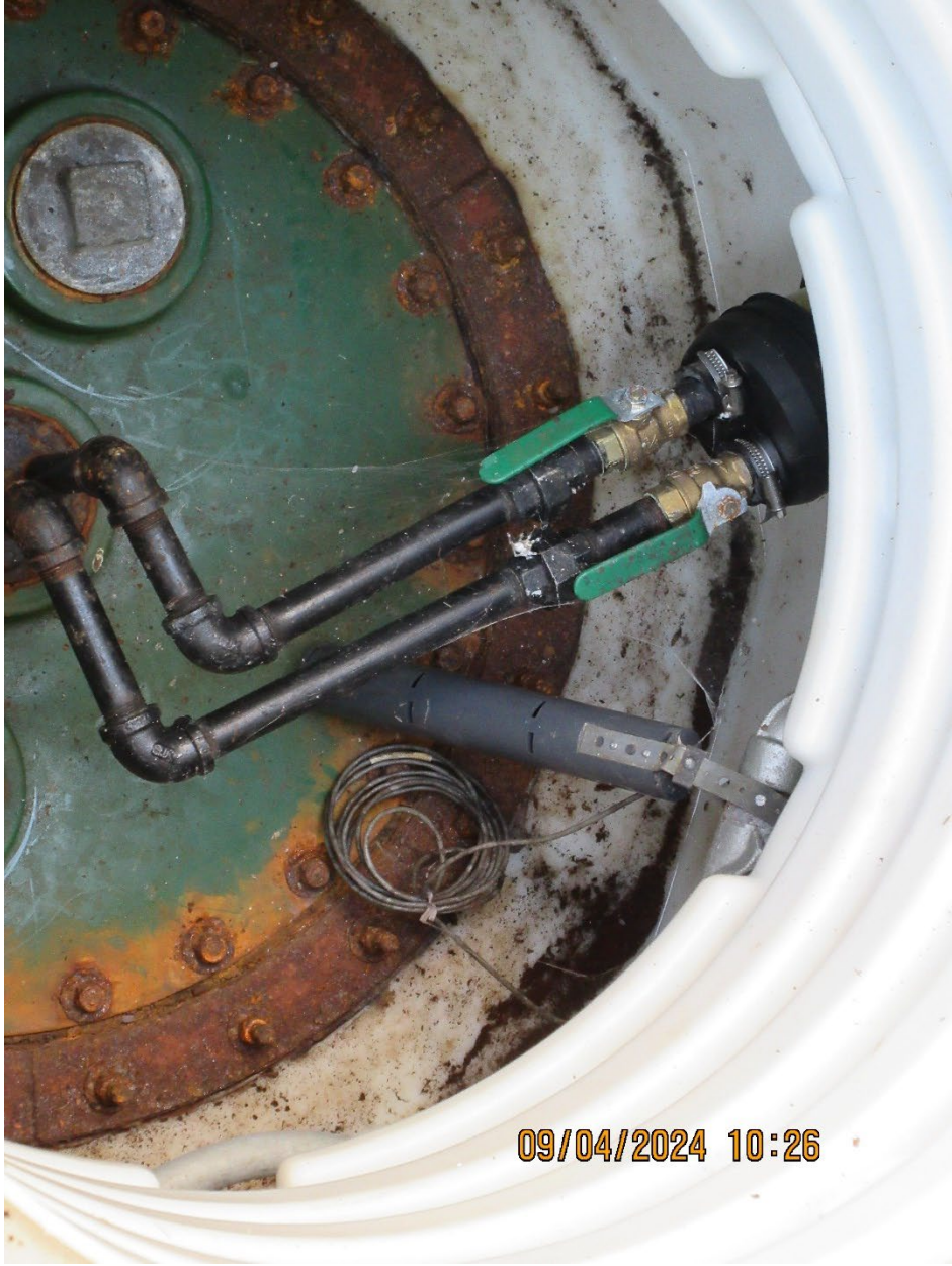
Photo 3 – Containment sump liquid sensor
