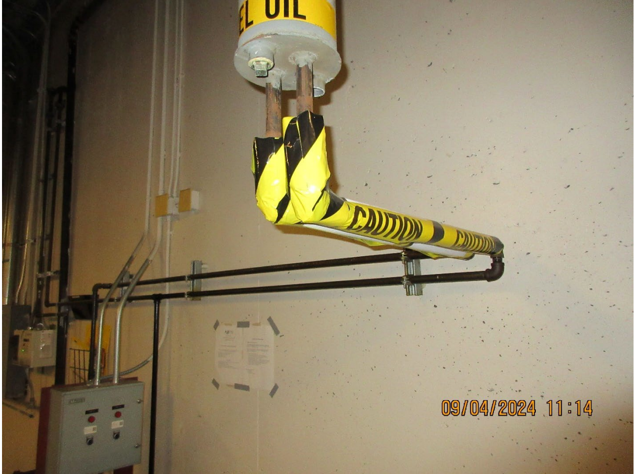
Photo 15 – Interior product pipes from the pump to the emergency generator on roof
