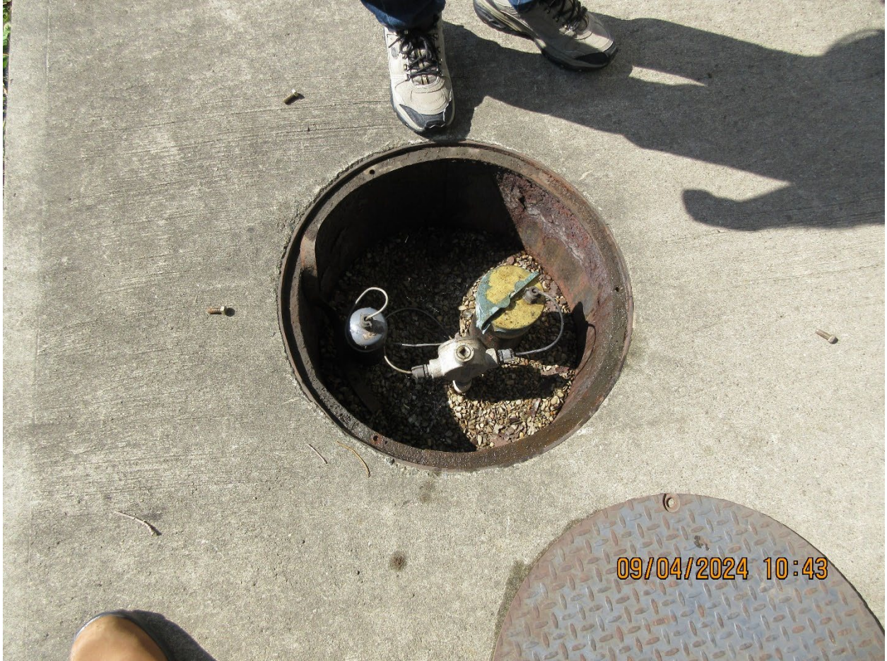
Photo 8 – Access port for ATG and HLA sensors
