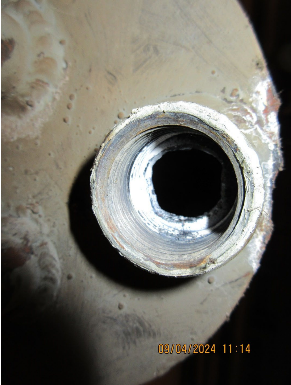
Photo 16 – Interior pipes to roof open double wall valve
