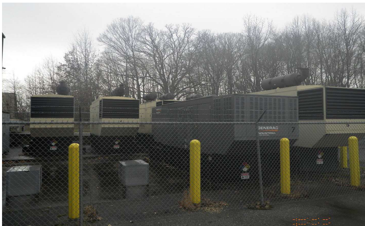
13. Overview of Generators 4, 5, 6, and 7 – Intelishift – 02/28/24
