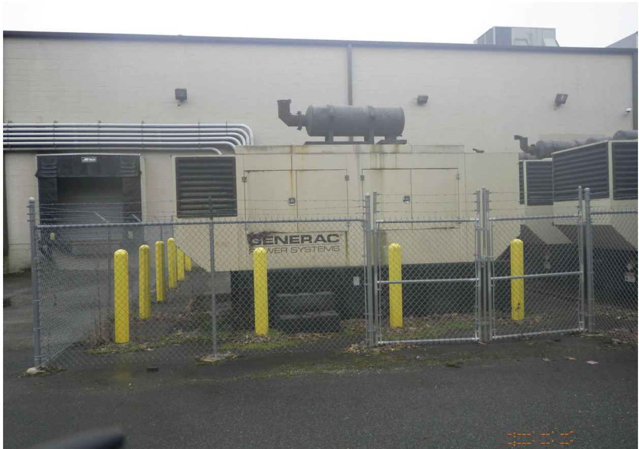
15. Overview of Generator 7 – Intelishift – 02/28/24
