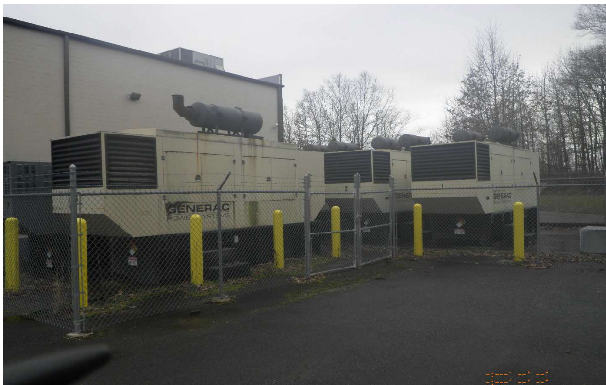
14. Overview of Generators 1, 2, and 7 – Intelishift – 02/28/24
