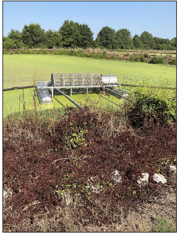
Photo 6: Lagoon- Cell 3 (non-functional rotating contactor and woody vegetation in berm).
