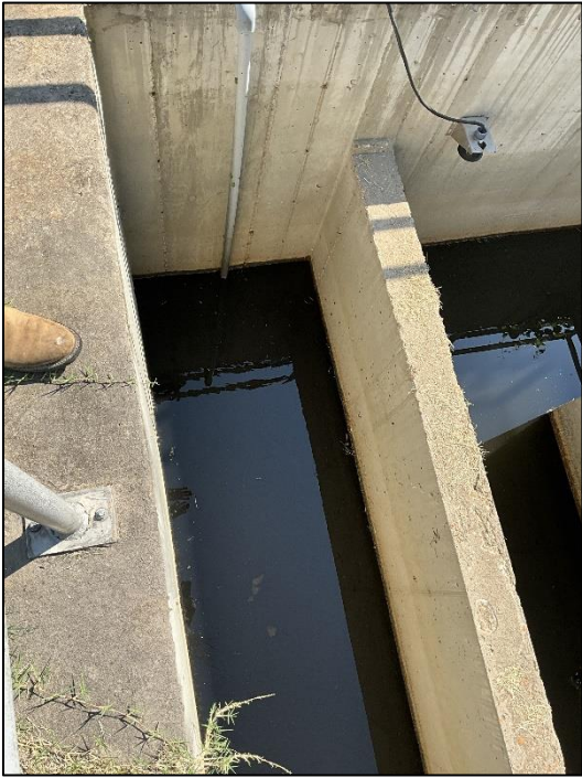
Photo 1: Chlorine injection point.
