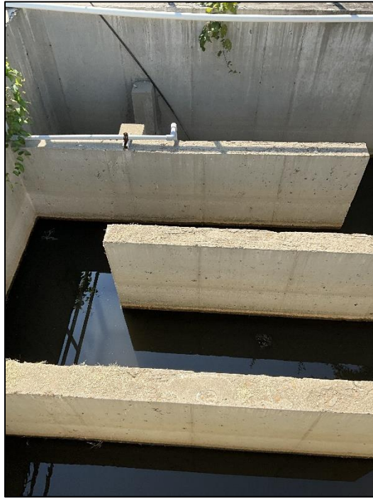
Photo 2: Sulfur Dioxide injection point.
