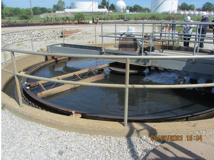
14: IMG_0334 Description: DAF unit Location: West of EQ basin Camera Direction: East Date/Time: 8/29/23, 3:04 p.m.
