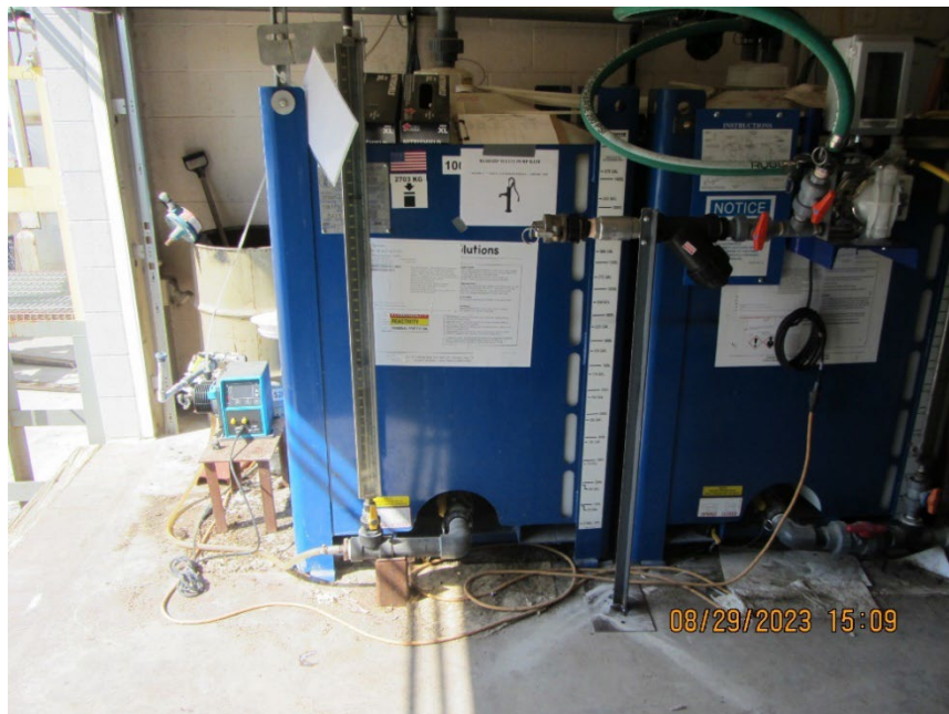
15: IMG_0335 Description: Totes of coagulant (left) and polymer (right) Location: South of DAF unit Camera Direction: North Date/Time: 8/29/23, 3:09 p.m.
