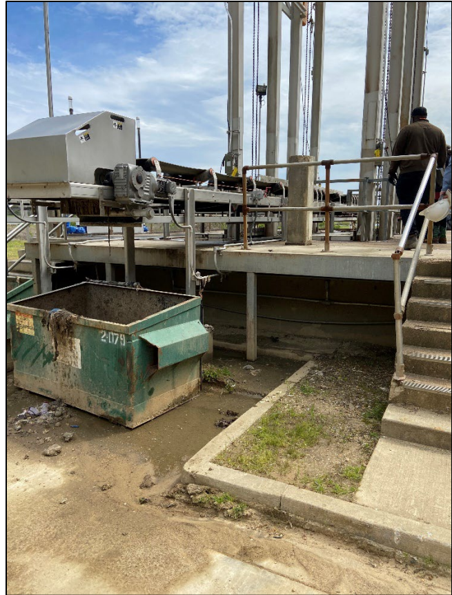
Photo 6: Bar screen dumpster and bar screens.
