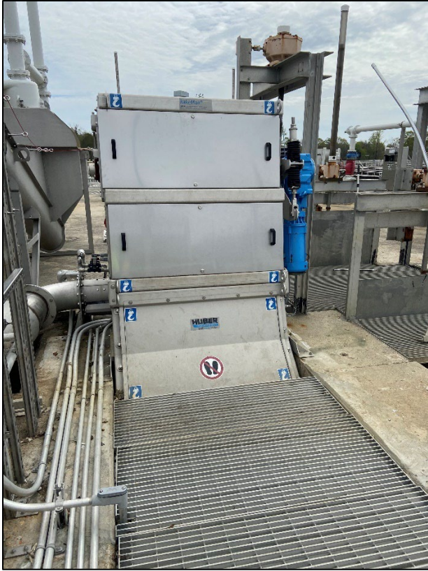
Photo 9: New fine screens.
