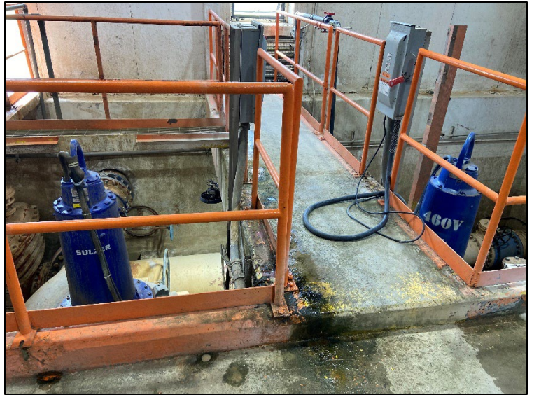
Photo 22: New RAS pump motors (three pumps in service).
