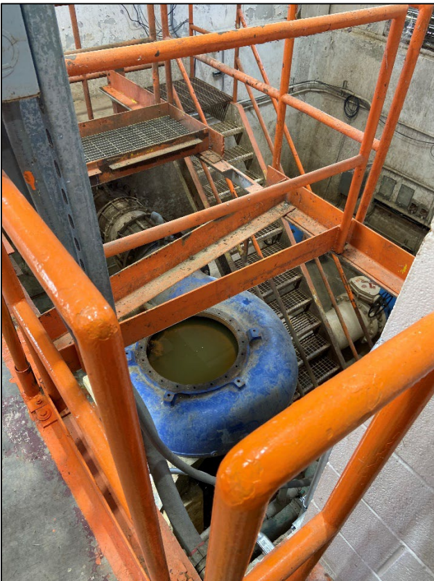
Photo 23: RAS pump out of service.
