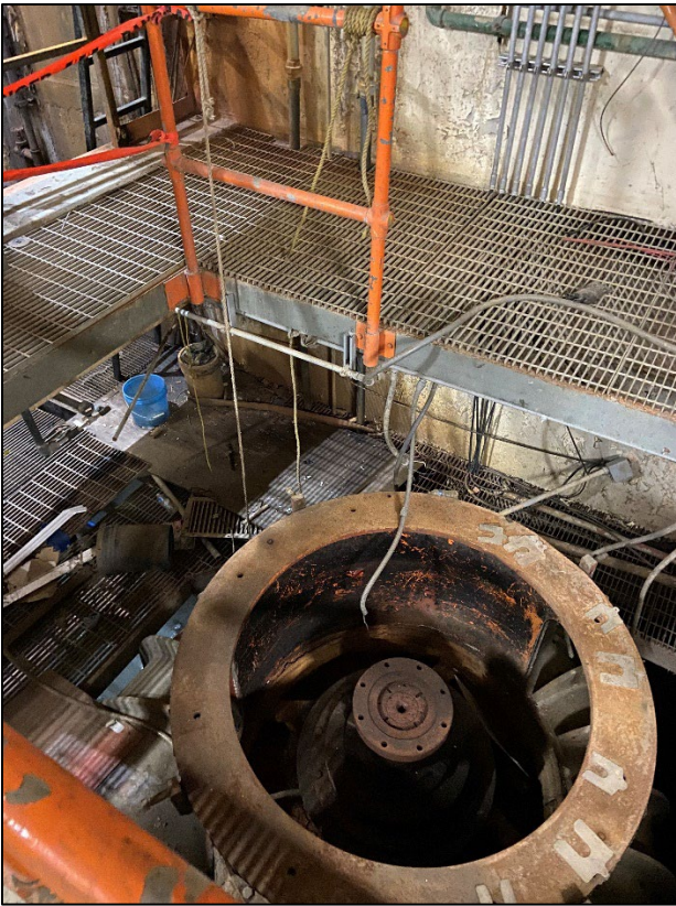
Photo 5: 100 MGD pump (out of service).
