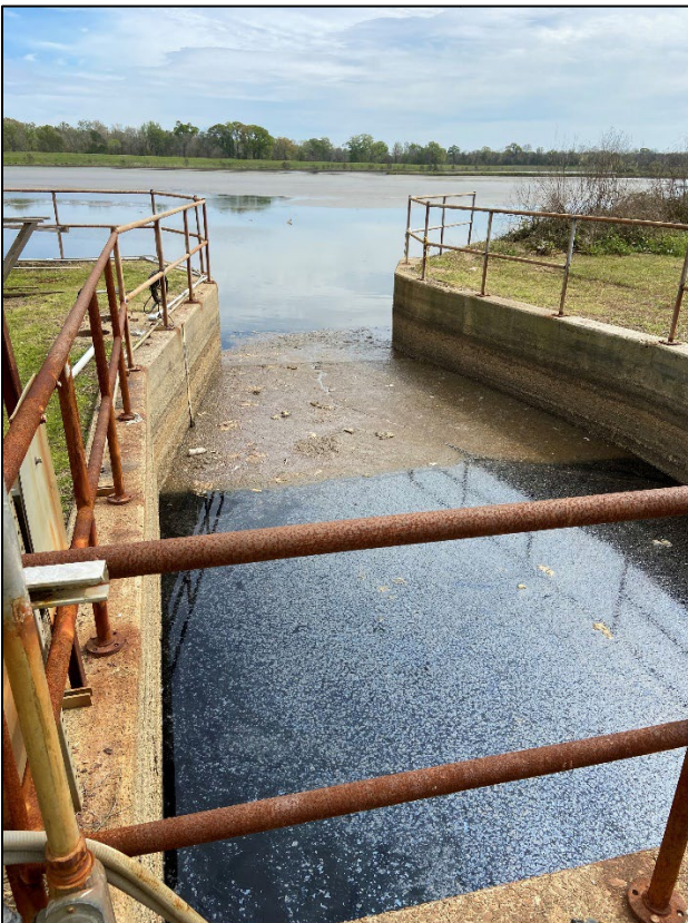
Photo 7: Influent channel to storm cells.
