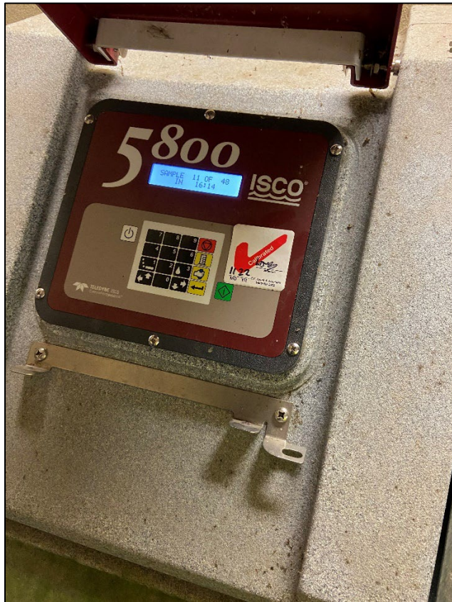
Photo 28: Effluent sampler calibration sticker.
