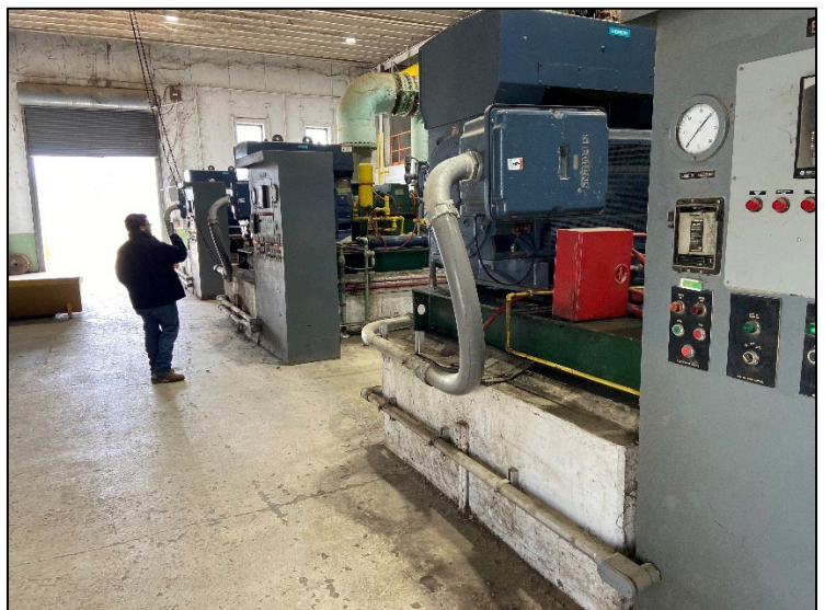
Photo 16: New blower controls.
