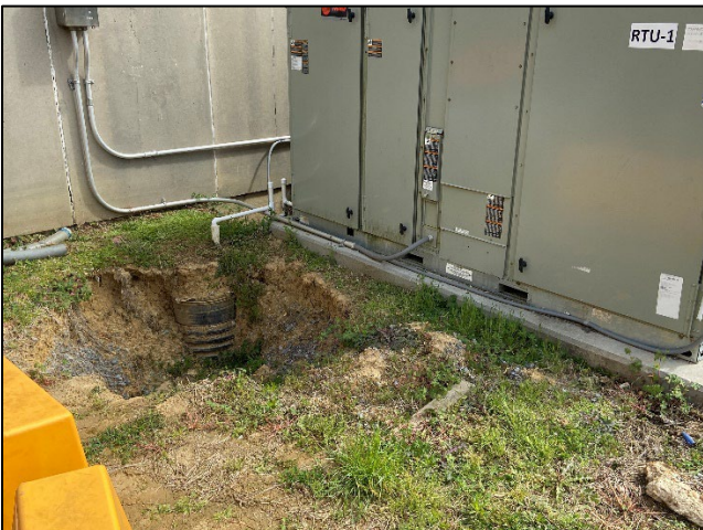
Photo 3: Sinkhole at influent pump station.
