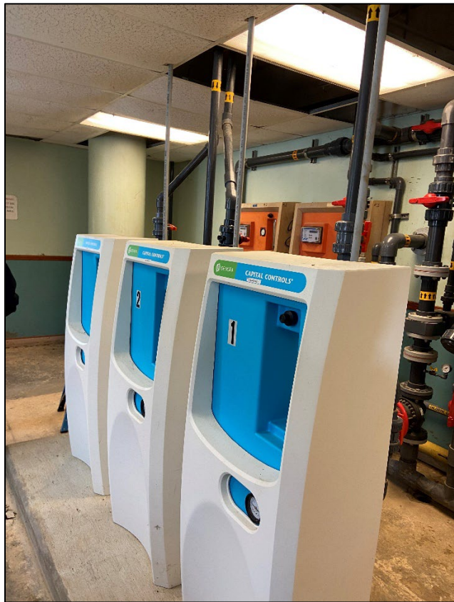
Photo 24: New electrical controls.
