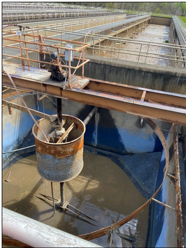
Photo 14: Sludge thickener (out of service).
