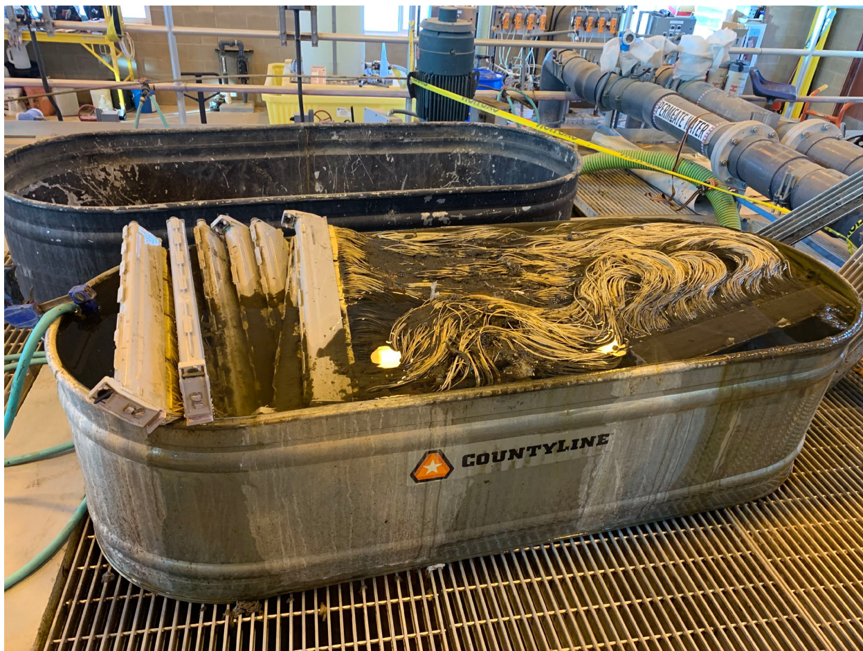
View of "spaghetti" type membranes awaiting cleaning. These membranes physically separate water from the microorganisms and suspended solids. (IMG_0223). Photographed by D. Esparza
