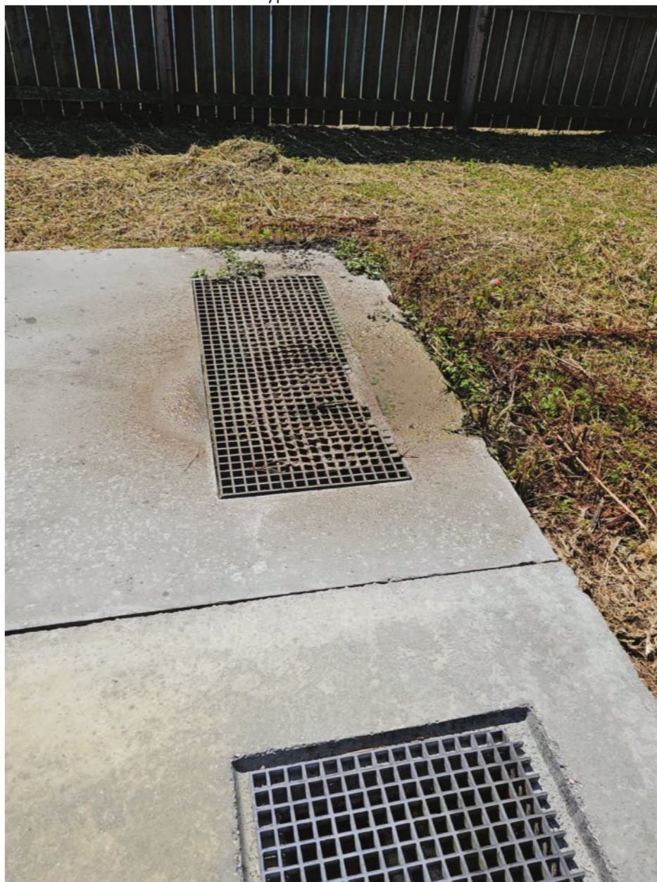
Bypass of Chamber
