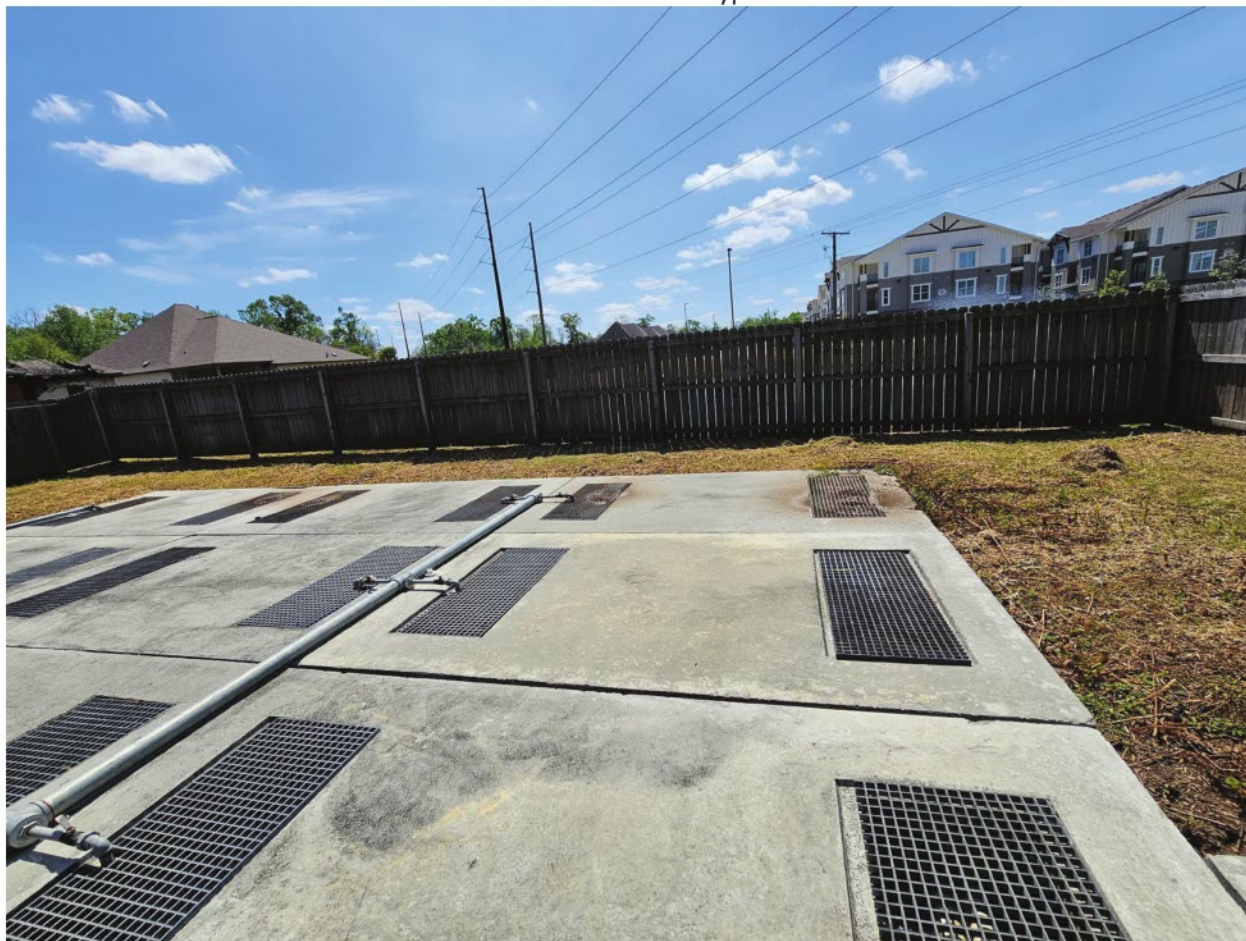
Aeration Chamber Bypass
