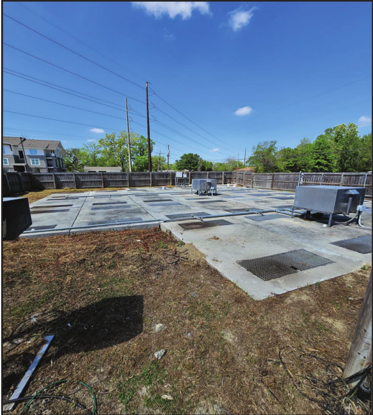
Extended Aeration In-ground Plant
