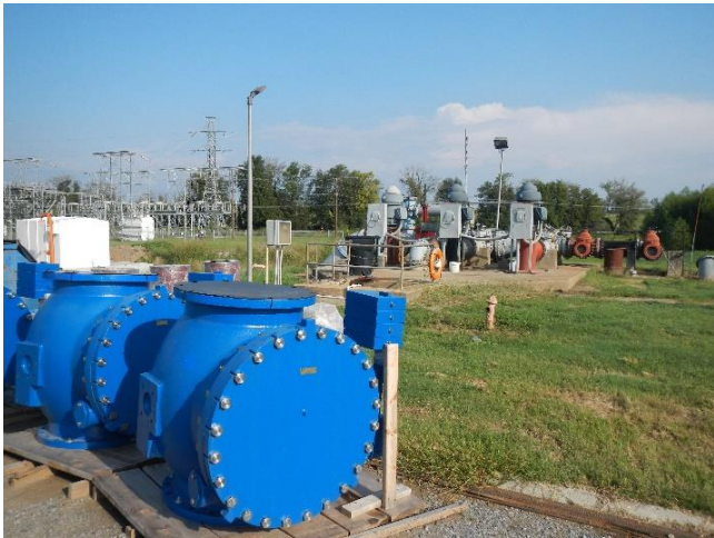
Photo 15: Effluent pump (gray pipes in background) and new check valves (blue).
