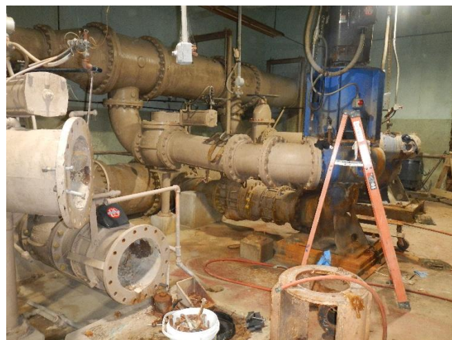
Photo 12: RAS pipes and pumps.
