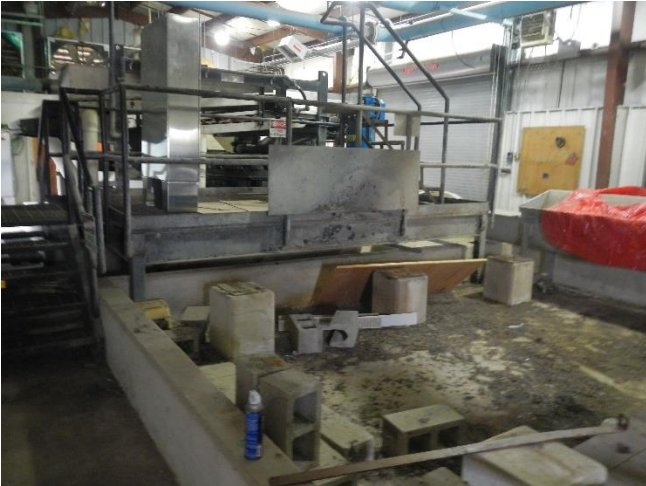
Photo 18: Sludge processing building. 2-meter belt press (aft) and slab for second belt press.
