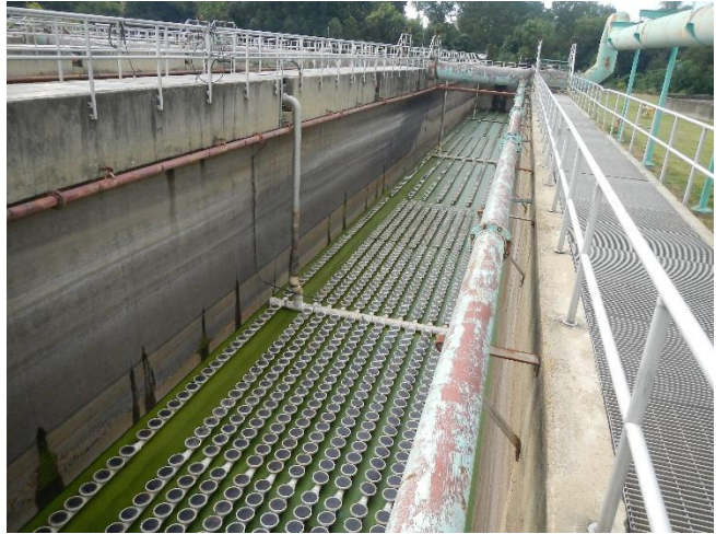
Photo 8: Aeration Basin 1. New air diffusers installed. Bypass channel is located under grates between the handrails.
