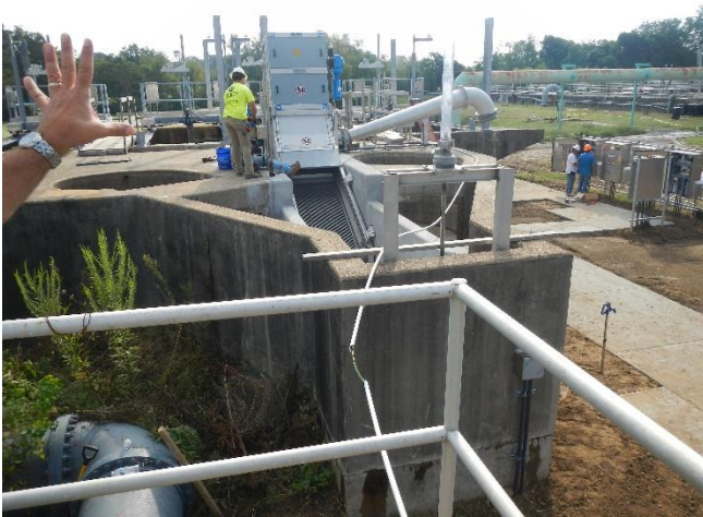
Photo 3: Headworks, bar screen and grit removal System.
