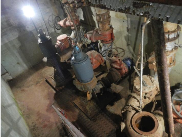
Photo 1. Influent pump station.
