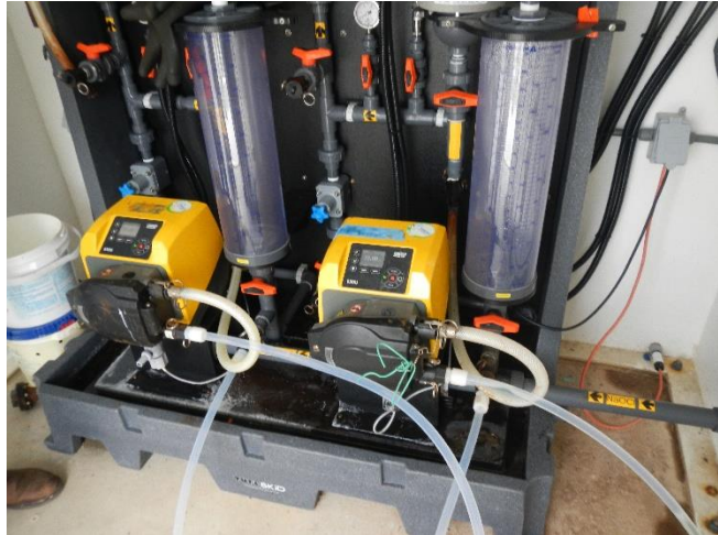
Photo 19: New polymer pumps for sludge processing.
