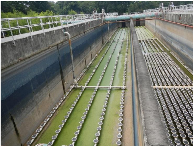
Photo 9: Aeration Basin 6 and Digester Basin 7 (left).
