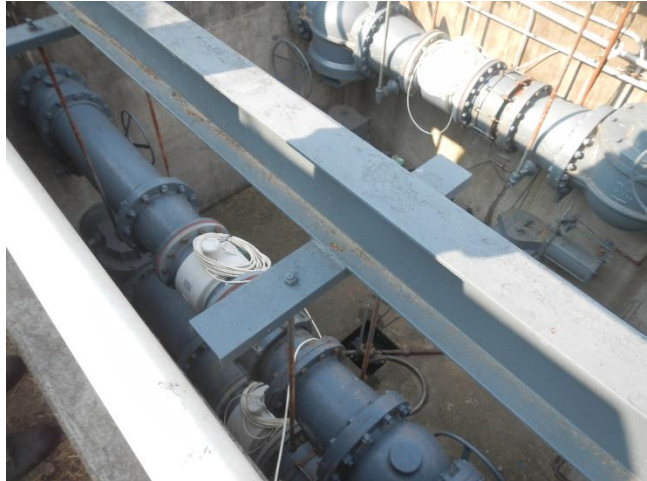
Photo 2: Influent Metering Vault.
