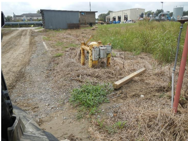
Photo 27: Ground water drawdown well on access road to Sludge Lagoons.
