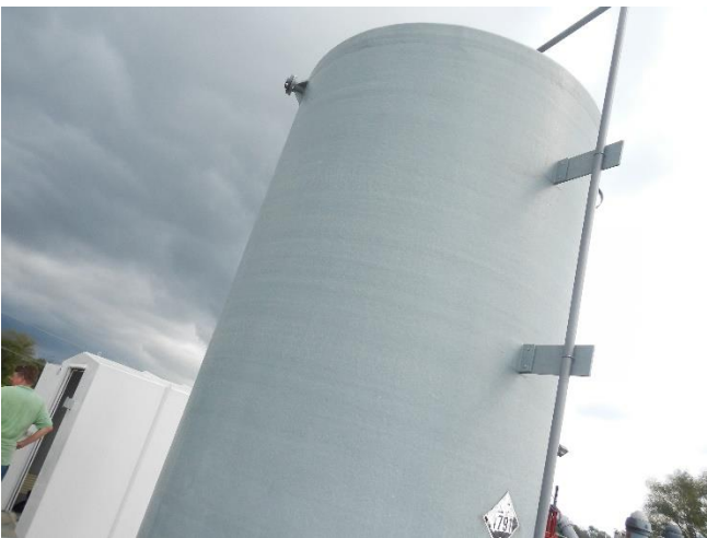
Photo 20: Interim NaClO disinfection tank.
