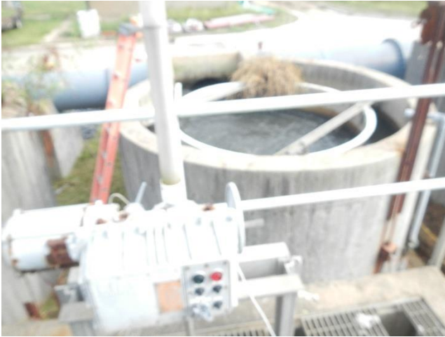
Photo 7: Original cyclone-type grit removal system.
