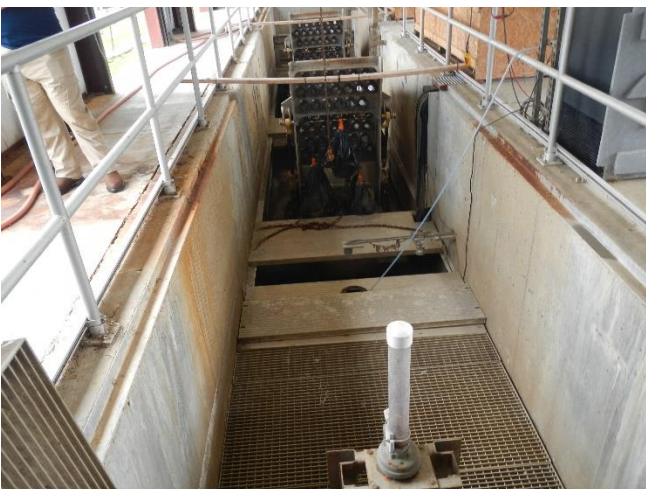
Photo 22: Ultra-violet light bulb fixtures and contact Chamber.
