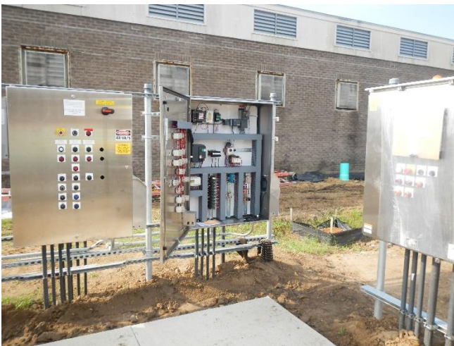
Photo 5: New headworks and grit removal control panels.
