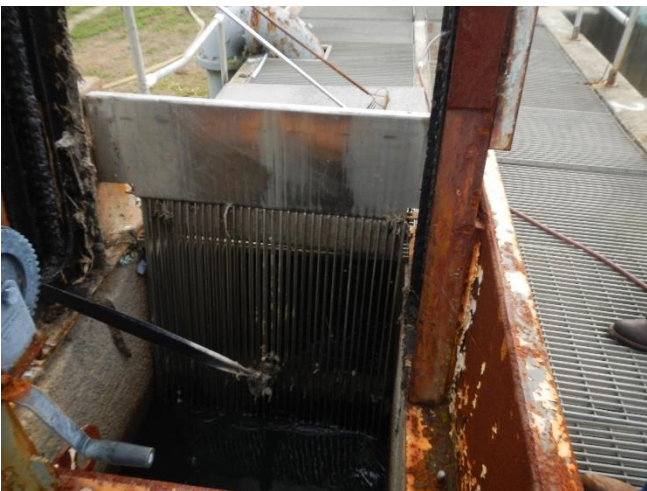
Photo 6: Bar screen for inflow to Digester Basin 8.
