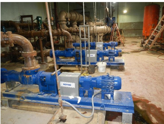
Photo 11: Return Activated Sludge (RAS) (brown pipes) and sludge pumps (blue piping)
