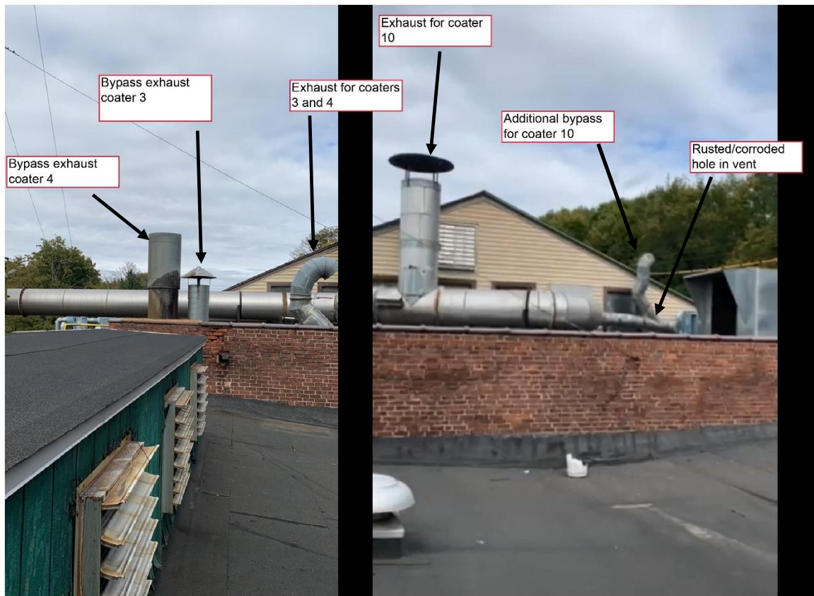
Photo 1. Trelleborg bypass ducts up on flat roof.
