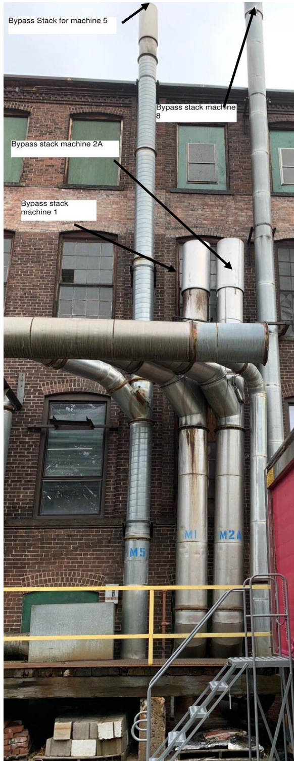
Photo 2. Trelleborg back wall bypass ducts.
