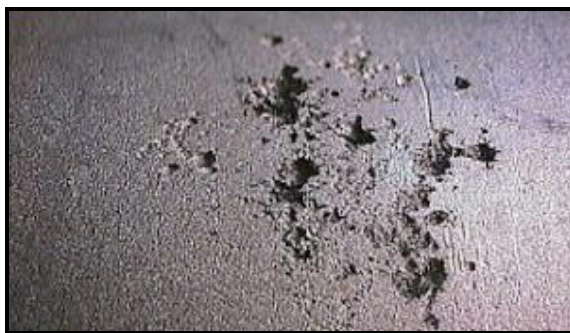
Figure 4.1: Pitting corrosion of stainless steel
