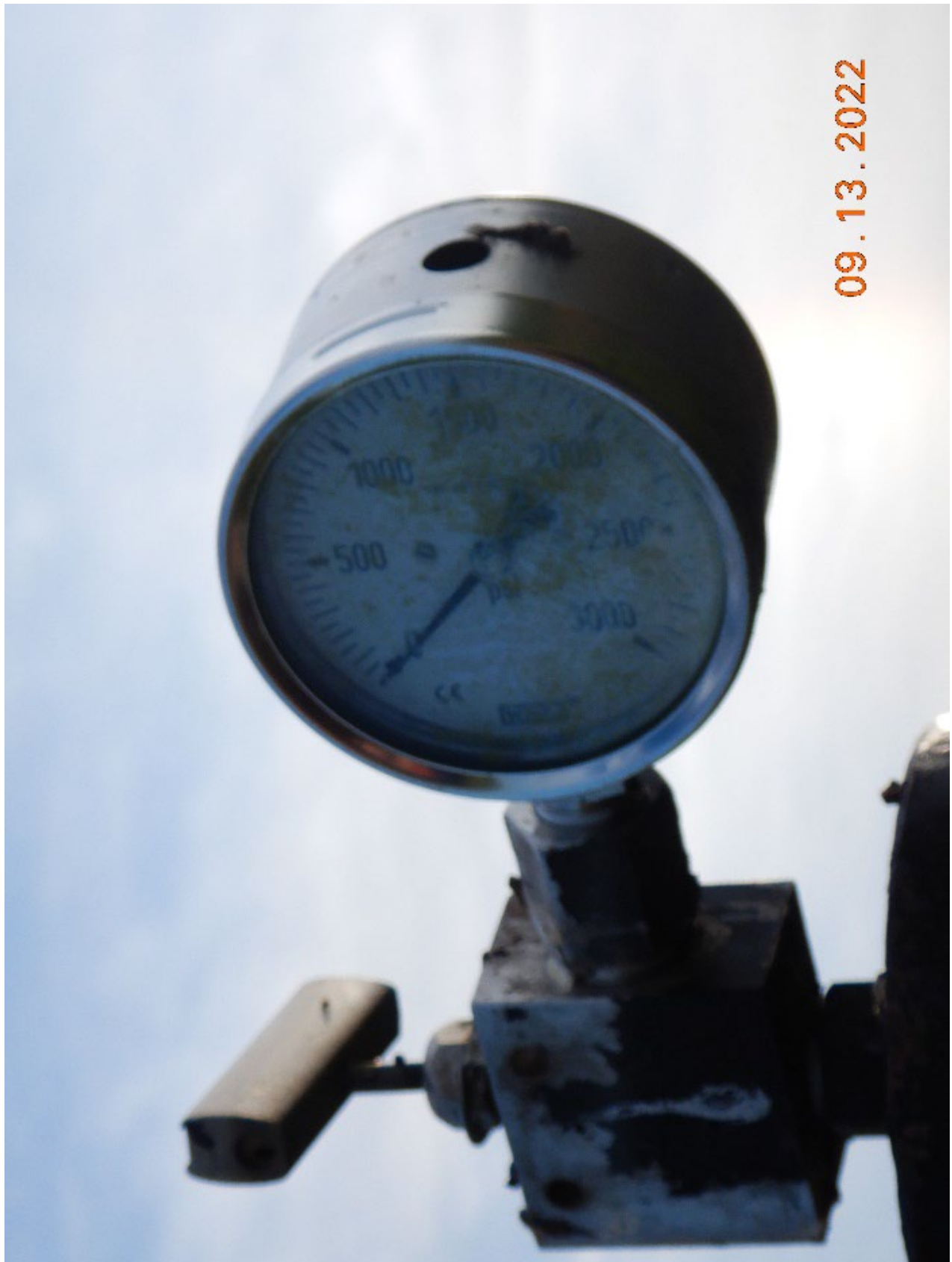
Photograph 3: Looking northeast, closeup view of internal pressure gauge reading 0 psi.
