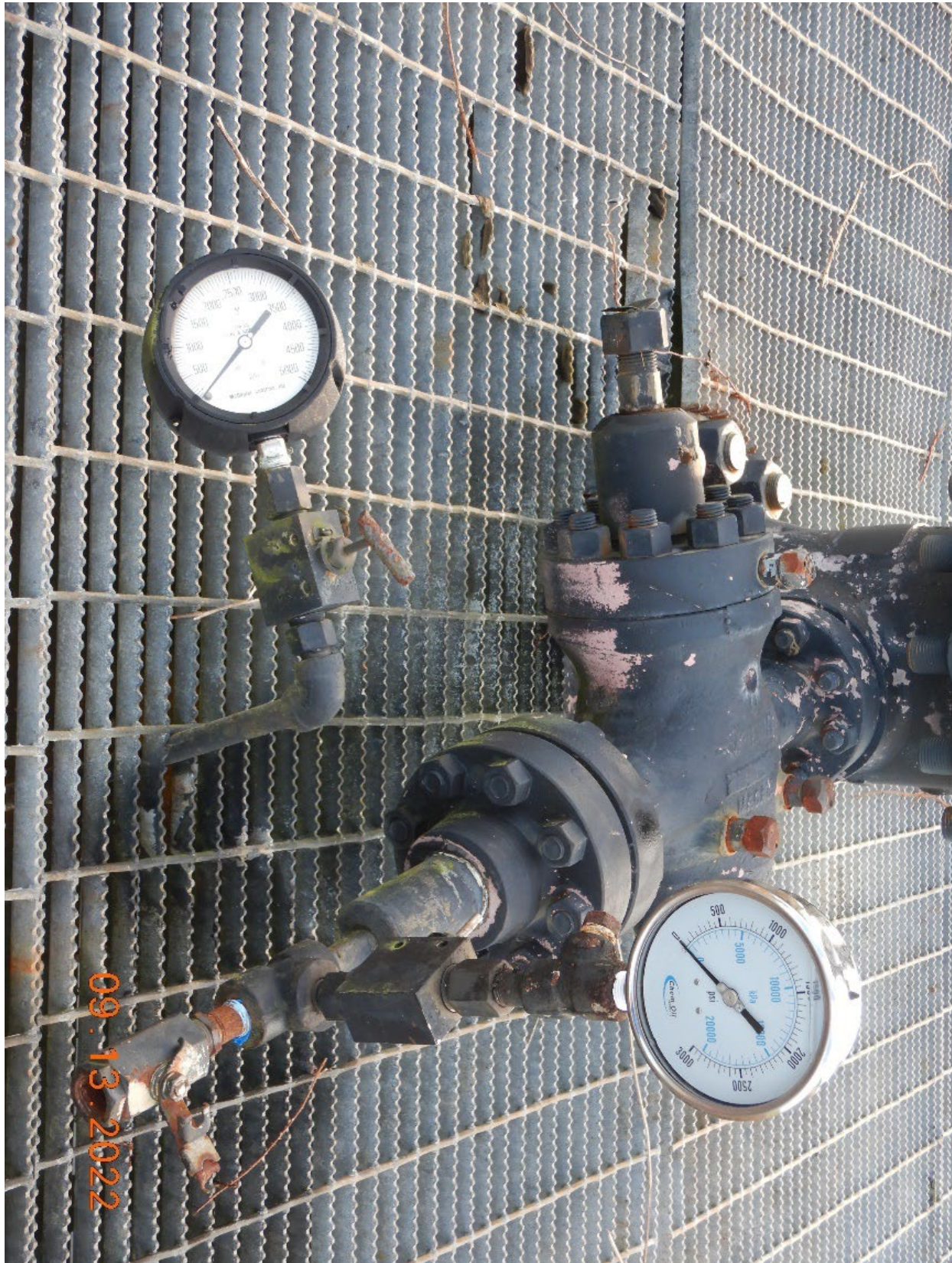
Photograph 2: Looking east, closeup view of surface casing pressure gauge (left, reading 0 psi) and production casing pressure gauge (right, reading 0 psi).
