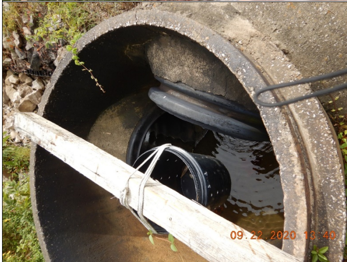
21: DSCN0057.JPG Location: Crane Naval Surface Warfare Center Photographer: Jonathan Moody Date/Time: 9/22/2020 1:40 PM Camera Direction: Down, South Description: At Outfall 012 from Pond 4. At the time of the inspection, this outfall was not discharging.
