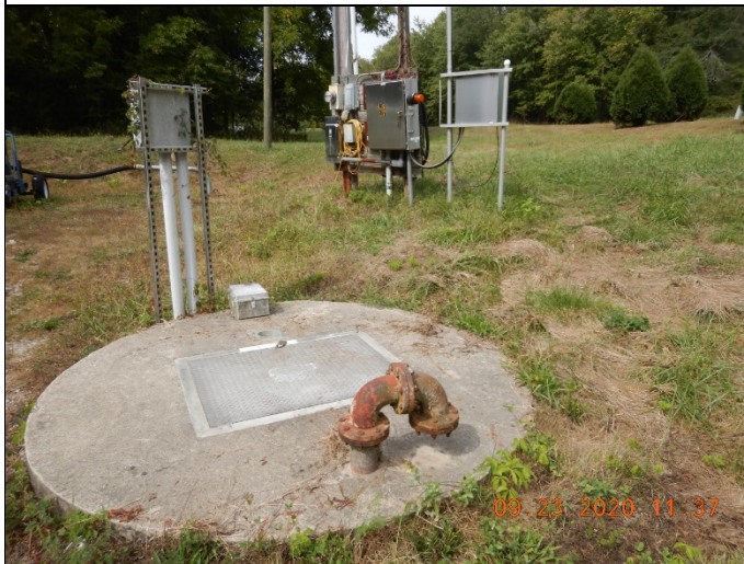
25: DSCN0061.JPG Location: Crane Naval Surface Warfare Center Photographer: Jonathan Moody Date/Time: 9/23/2020 11:37 AM Camera Direction: West Description: Lift Station 17, located on the southside of Highway 5 and ½ mile west of the Crane Naval Surface Warfare gate.
