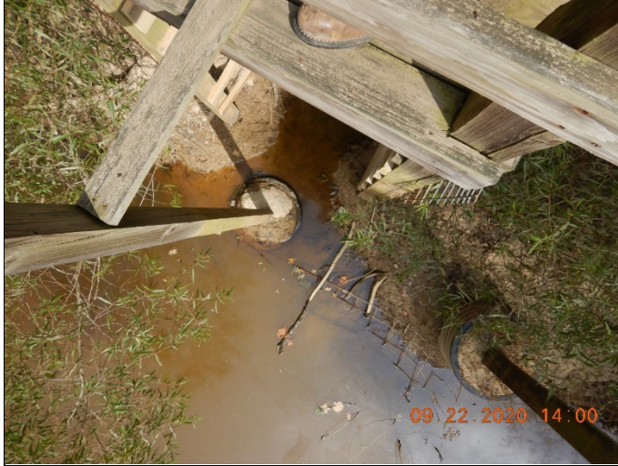
23: DSCN0059.JPG Location: Crane Naval Surface Warfare Center Photographer: Jonathan Moody Date/Time: 9/22/2020 2:00 PM Camera Direction: Down Description: The control structure at Pond 3 which drains to Pond 3A. At the time of the inspection, the trash rack was off the control structure.
