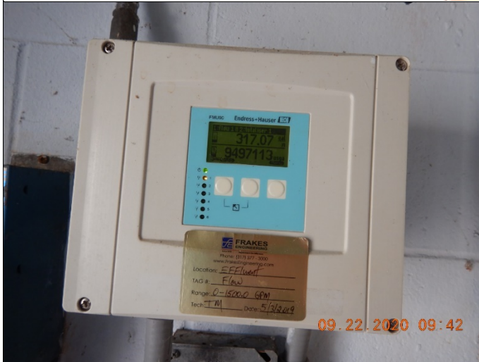
6: DSCN0042.JPG Location: Crane Naval Surface Warfare Center Photographer: Jonathan Moody Date/Time: 9/22/2020 9:42 AM Camera Direction: Inside, South Description: Inside the building with the filters with the readout from the flow measurement flume shown in DSCN0039.JPG and DSCN0040.JPG. At the time of the inspection, the reading was fluctuating around 317 GPM, or 456,000 Gallons/day.
