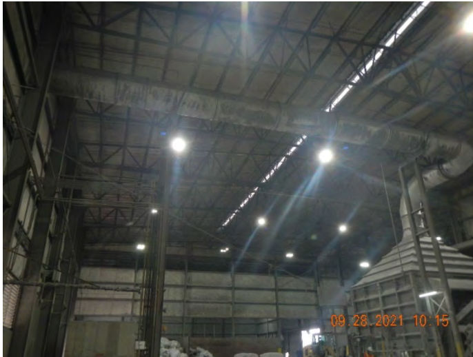
Photo #:05 (DSCN2490) Description: Facing north, photo of Rotary Furnace #3 capture hood and ducting.
