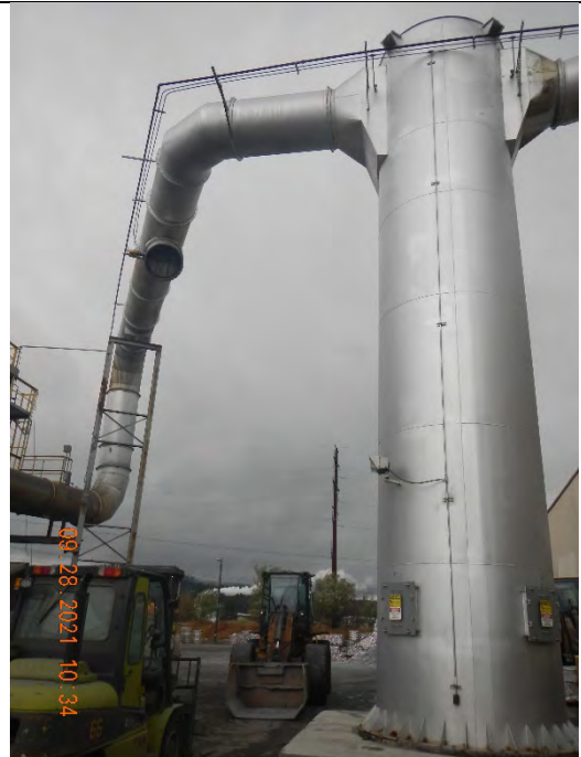
Photo #:08 (DSCN2498) Description: Facing northwest, photo of Baghouse #3 cooling tower.
