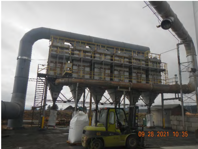
Photo #:07 (DSCN2499) Description: Facing west, photo of Baghouse #3.
