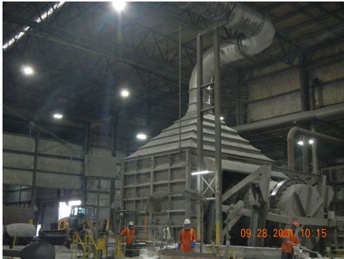
Photo #:03 (DSCN2489) Description: Facing north, photo of Rotary Furnace #3 enclosure and capture hood.
