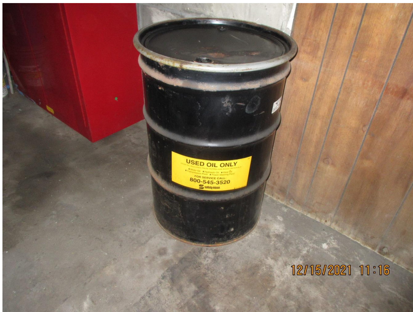
Photo 13 – Used oil from condenser blowdown
