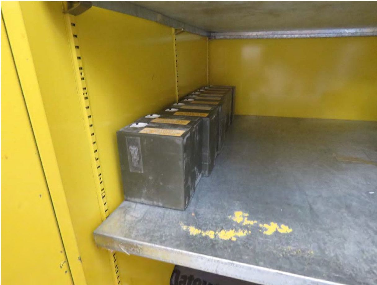
In-use lithium manganese dioxide batteries at building 1678.
