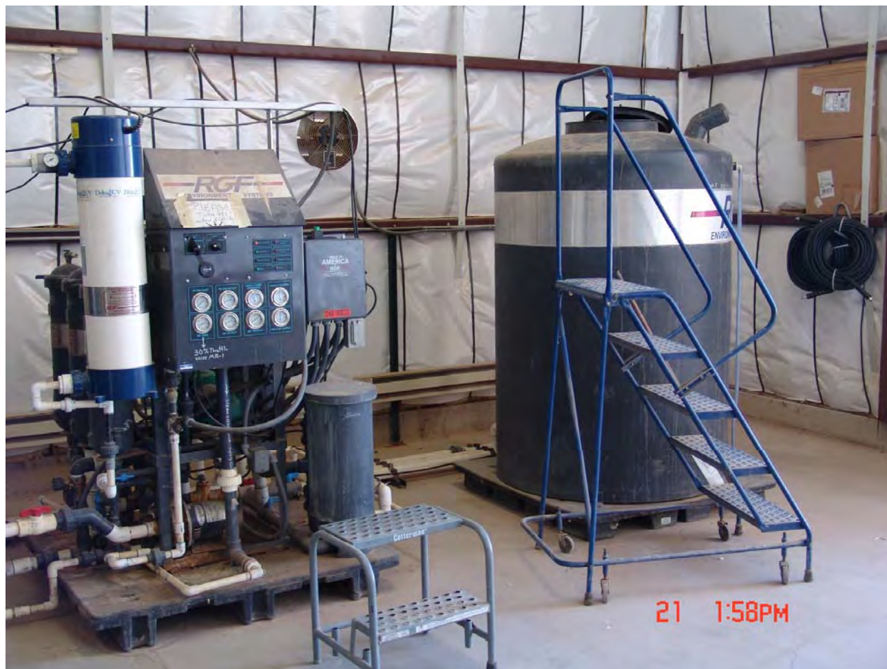
Wash rack at Material Test Directorate bldg. 2780 main filtering unit and tank #2.
