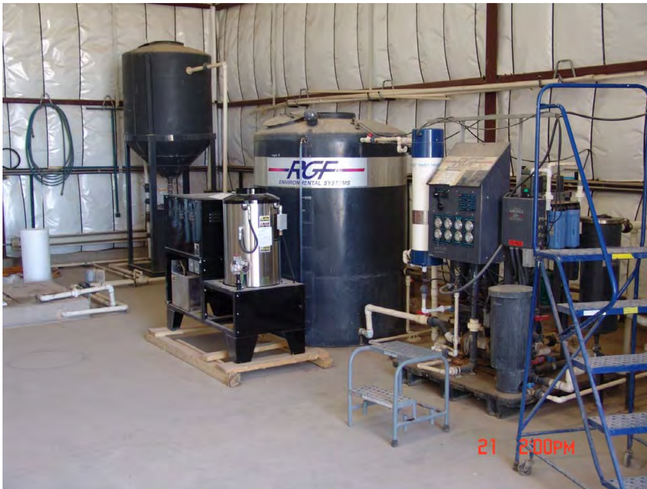
Wash rack at Material Test Directorate bldg. 2780 overall equipment view.
