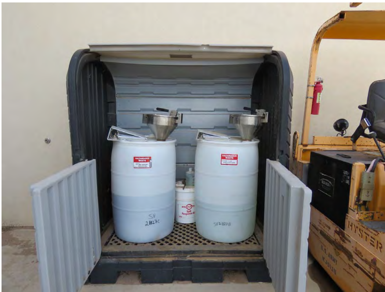
Satellite Accumulation Points at Building 21127 with containment open
