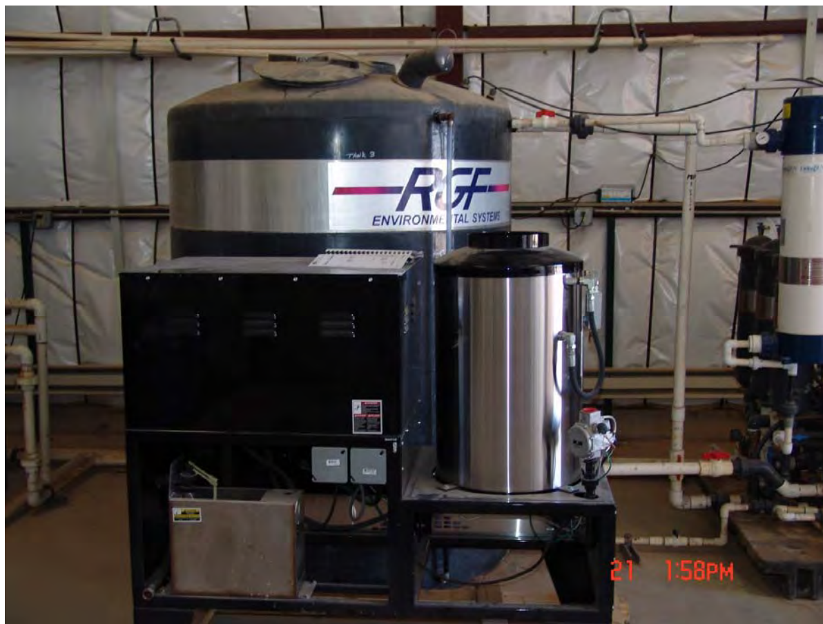
Wash rack at Material Test Directorate bldg. 2780 water heating unit and tank #3.
