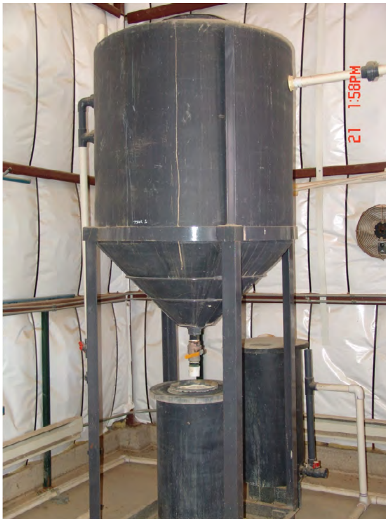
Wash rack at Material Test Directorate bldg. 2780 cyclone filter.
