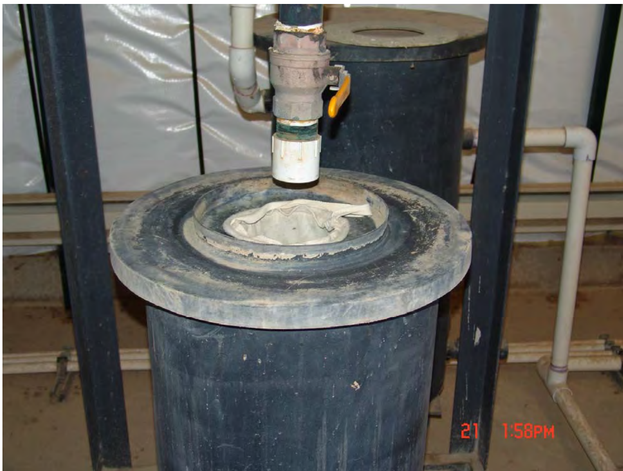
Wash rack at Material Test Directorate bldg. 2780 cyclone filter solids removal drain.
