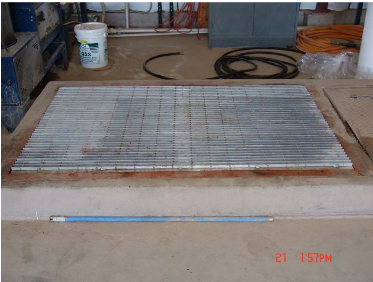
Wash rack at Material Test Directorate bldg. 2780 oily water sump.
