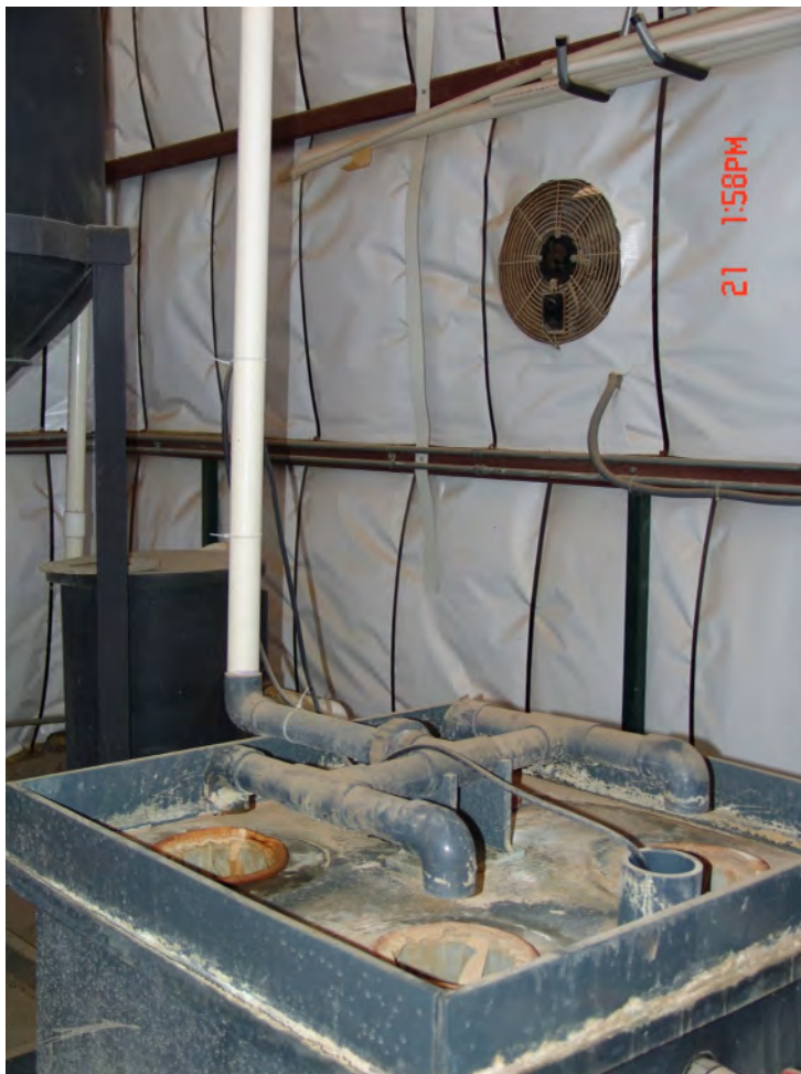
Wash rack at Material Test Directorate bldg. 2780 sock filter.
