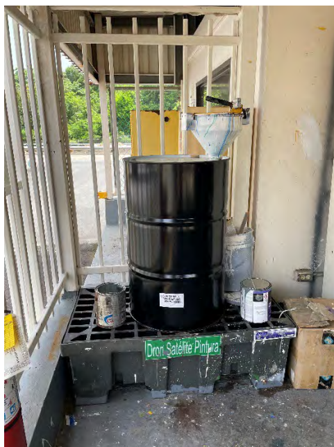
Photograph 2: Paint Shop SAA; 55-gallon drum of waste paint not marked and/or labeled with the words “hazardous waste” nor with an indication of the hazards of the contents.
