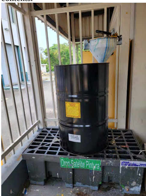
Photograph 6: Facility's corrective action – Paint Shop SAA with a 55-gallon drum of waste paint marked and/or labeled with the words “hazardous waste” and with an indication of the hazards of the contents.
