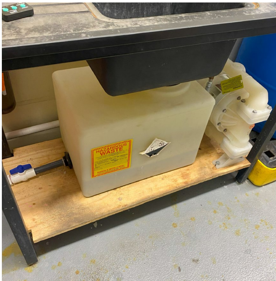
(Figure 1: Hazardous waste label put on tank located in the etching room)
