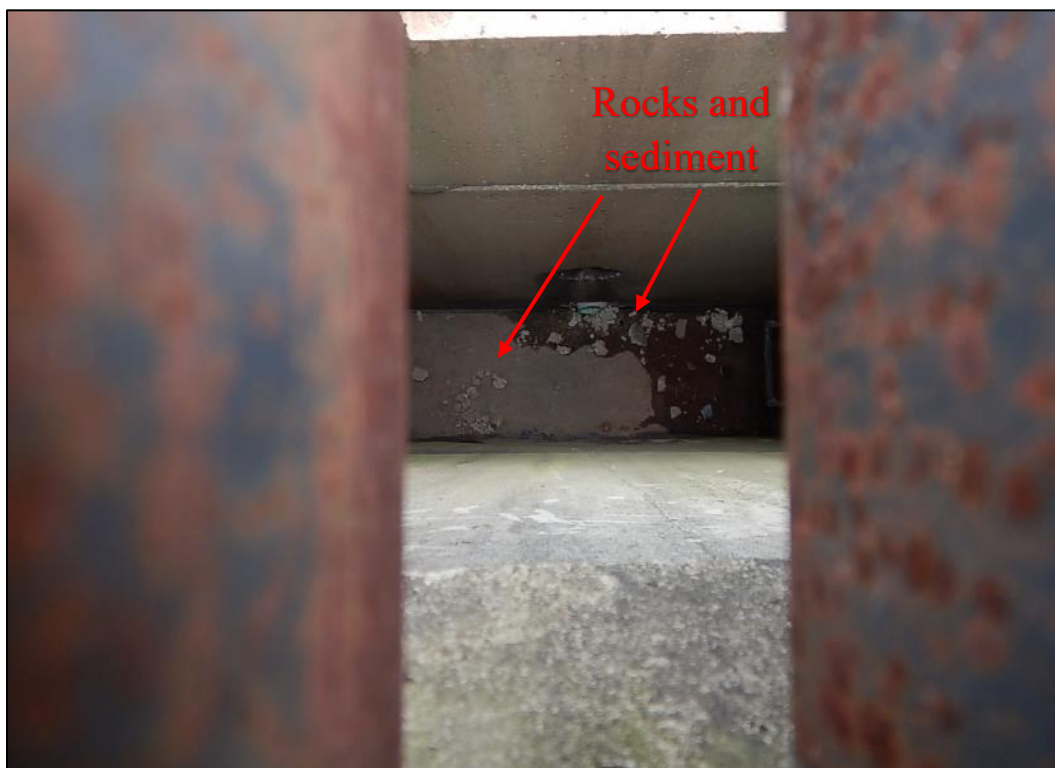
Photograph 40. View inside the concrete riser outlet structure. Note the rocks and sediment inside the structure.
