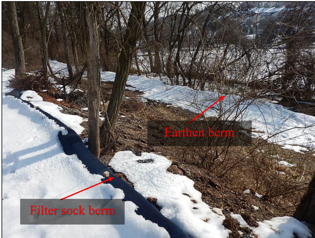
Photograph 20. View, facing southeast, of a filter sock berm located in the stockpile area as well as an earthen berm located down gradient along the perimeter of the property.
