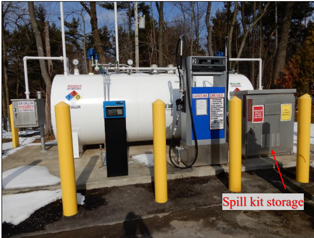
Photograph 16. View, facing north, of the fueling station. The station had a joint aboveground tank for gasoline (500 gallons) and diesel (2,000 gallons) on the northern border of the property.
