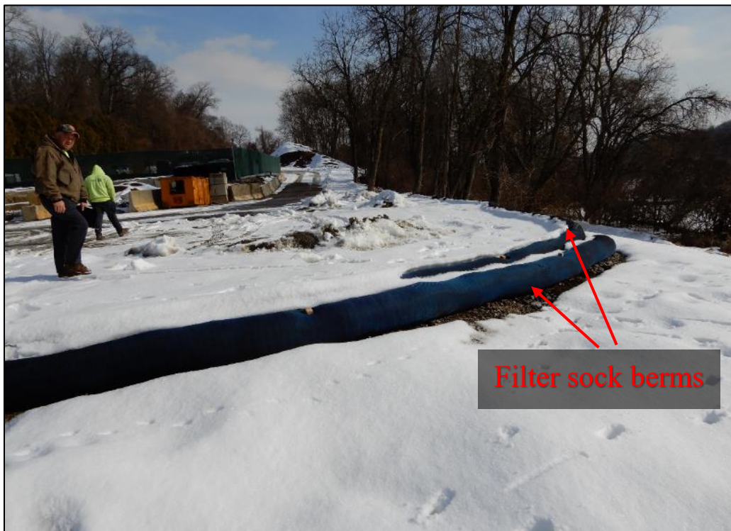
Photograph 19. View, facing northeast, of two filter sock berms used to control runoff in the the northeastern portion of the property.
