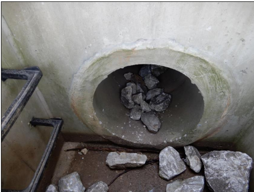
Photograph 46. View inside the concrete riser outlet structure. Note the rip rap inside the structure.
