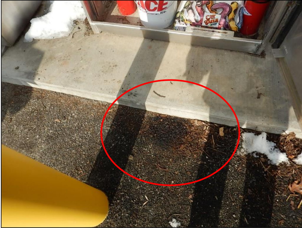
Photograph 18. Apparent petroleum stain in front of the spill kit storage at the fueling station.
