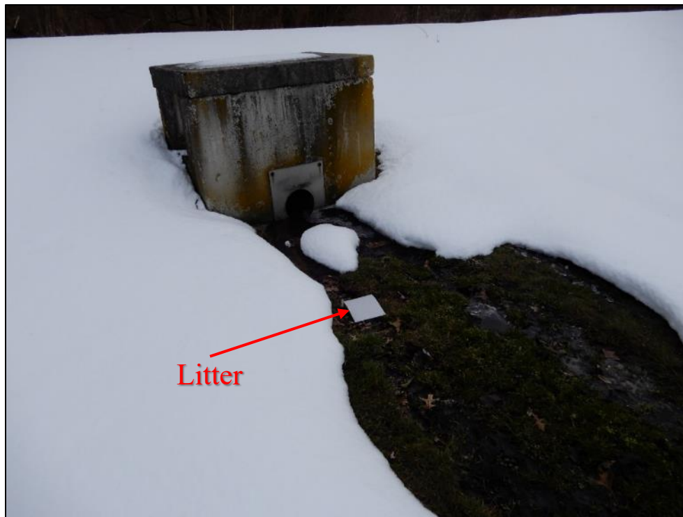
Photograph 27. View, facing west, of the outlet structure. Note that the concrete channel is not visible due to the vegetation growing in the accumulated mud and sediment in front of the structure. Litter was also present near the outlet.
