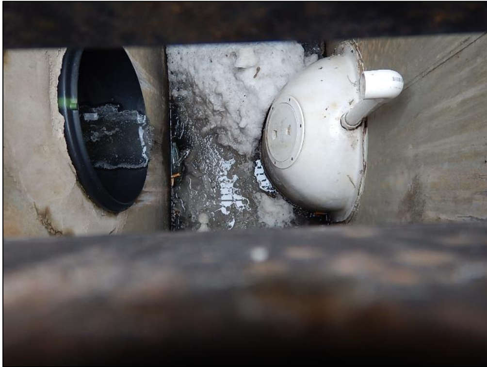
Photograph 22. View of the water quality snout device installed in the catch basin upstream of the stormwater basin.
