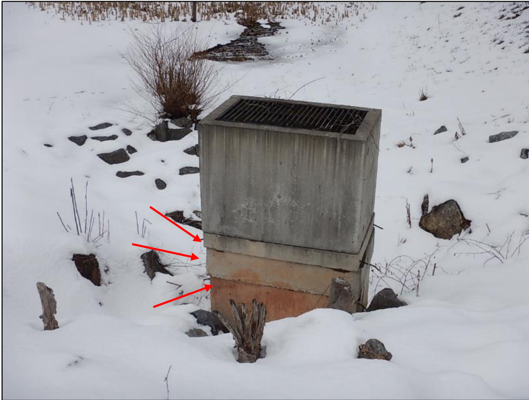
Photograph 24. View of the concrete riser outlet structure. The red arrows show where the riser sections were apparently not aligned.
