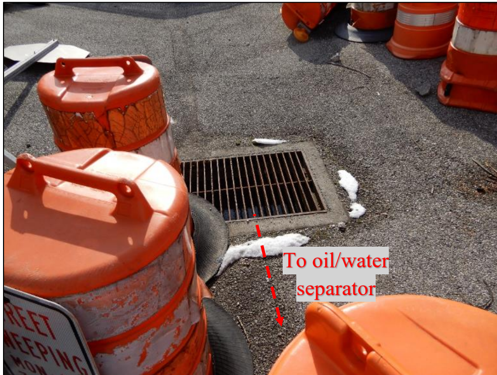
Photograph 10. View, facing south, of the catch basin that collects vehicle wash water and routes it to the oil/water separator.
