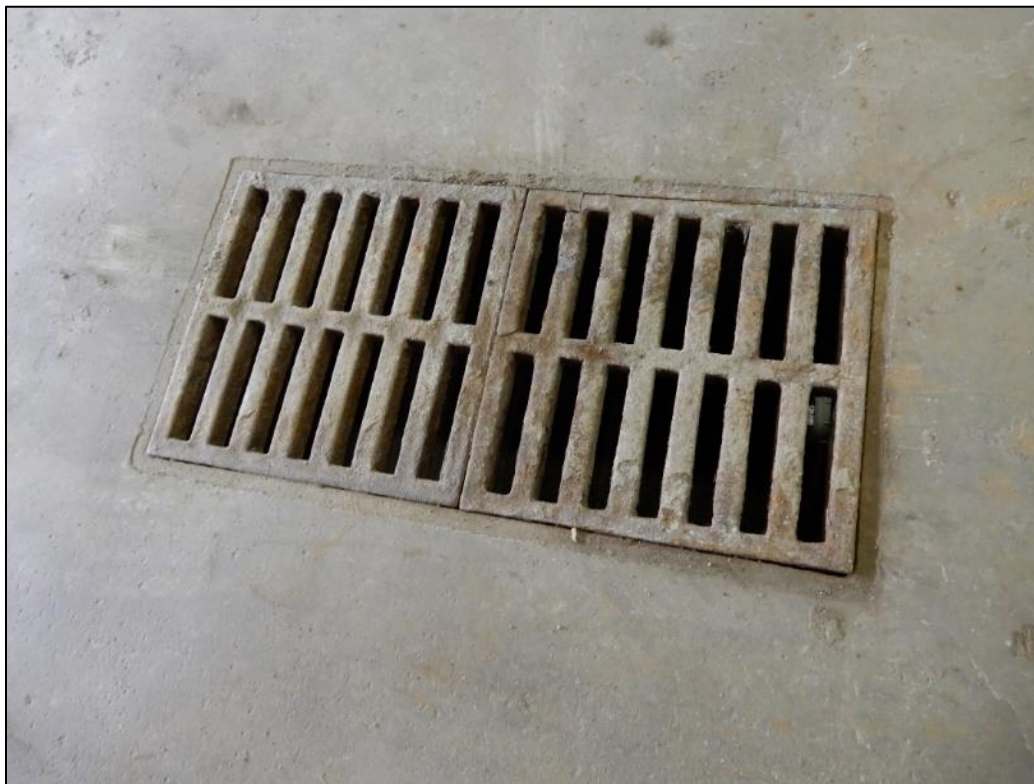
Photograph 7. View of another drain in the garage. Township staff stated the drains were plugged.
