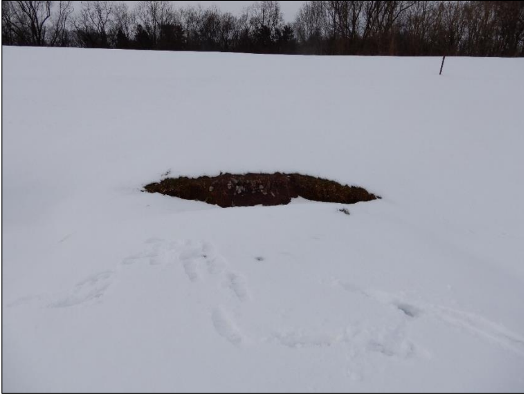
Photograph 41. View, facing northwest, of erosion in the center of the stormwater basin.
