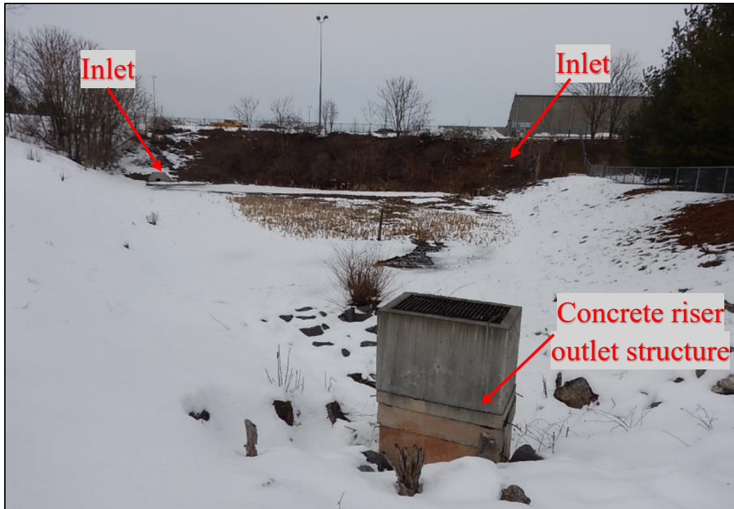
Photograph 23. View, facing northwest, of the stormwater basin and concrete riser outlet structure. The riser structure was not aligned.
