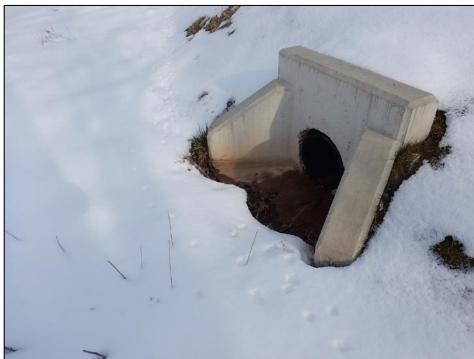
Photograph 4. View of the outlet for the new stormwater pond. Note that sediment was observed at the outlet.
