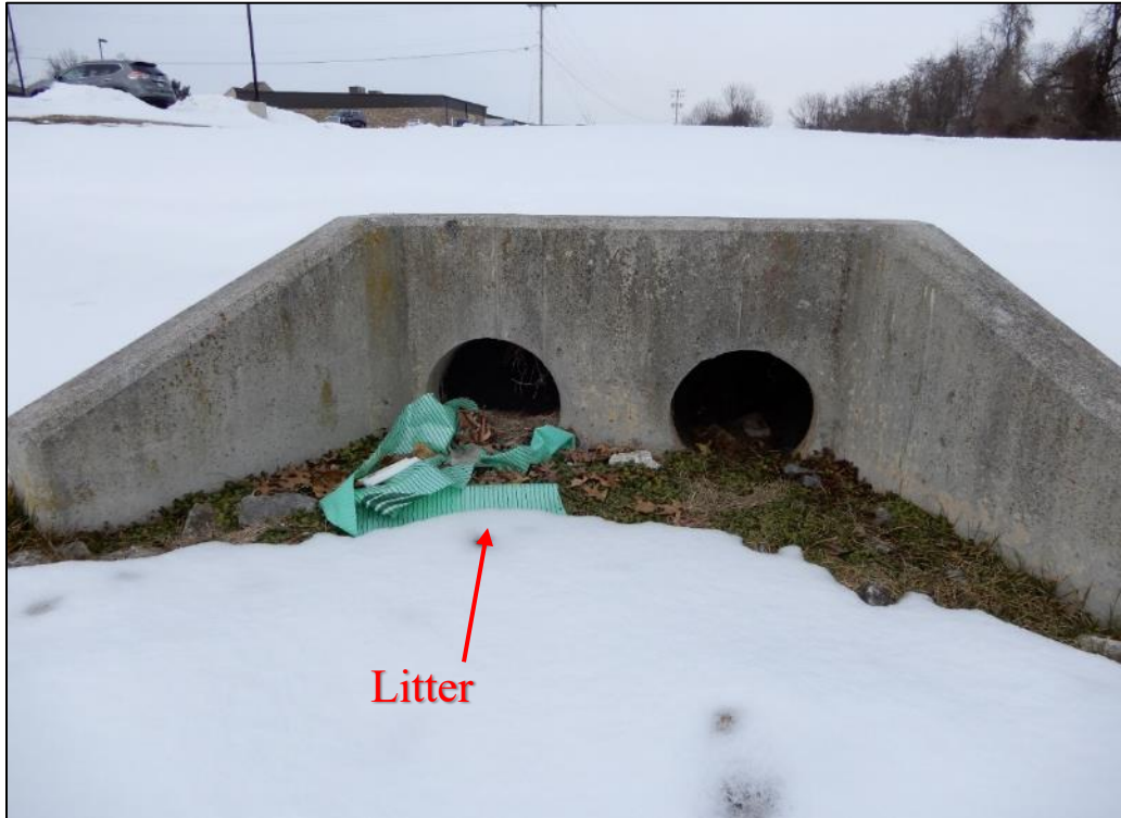
Photograph 28. View, facing north, of the stormwater basin inlets on the north side of the BMP which allow flow to enter the structure from the Advanced Auto stormwater basin. Note the trash observed at this location.
