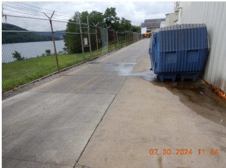
Figure 5: Photo from inspection, water was flowing from right to left across the pavement toward the Ohio River seen in the background
