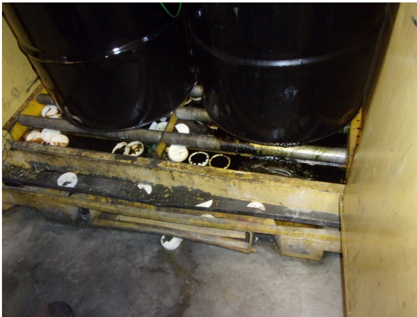
Photo 4 – Spills observed in secondary containment of flammable cabinet storing drums of hazardous waste.
