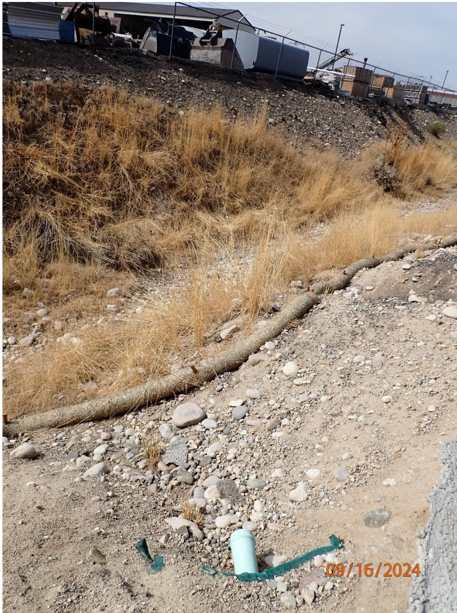
Photo 8 - Small area of erosion leading into Fivemile Creek (dry)
