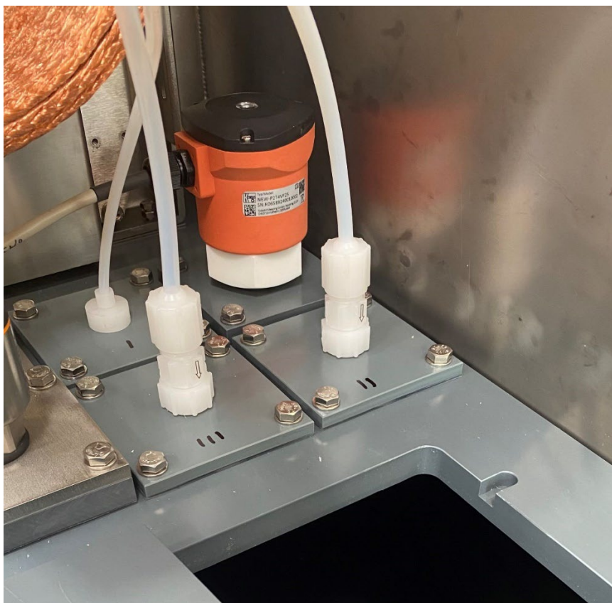
Figure 3: Reservoir of the plating unit where the chromium electrolyte and the wetting agent are contained
