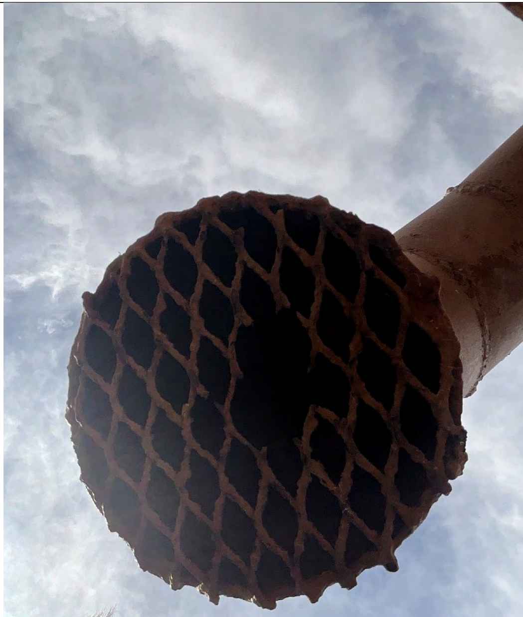
Station #2 - GST vent with large mesh screen and large hole in the screen
