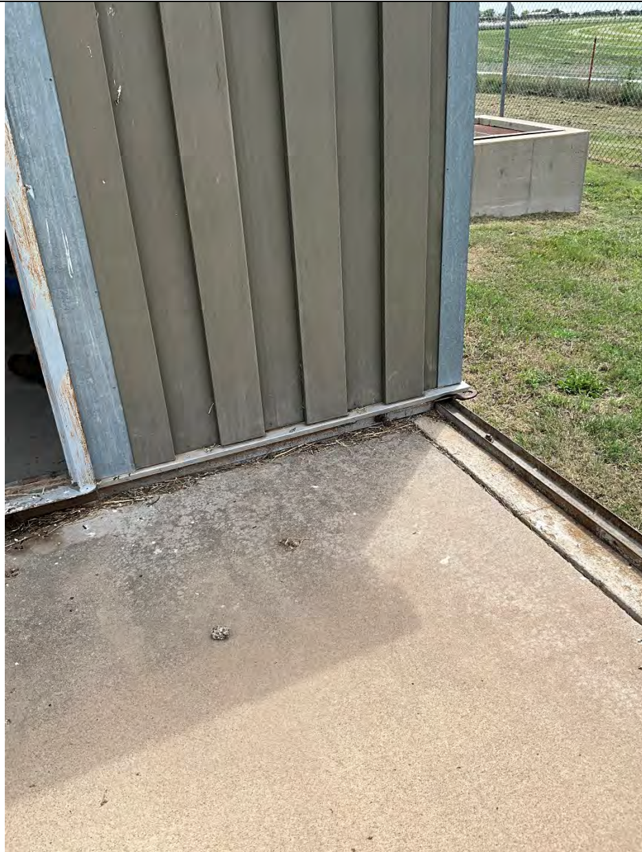
Well #35 – Well building on tracks to allow access to the pump components
