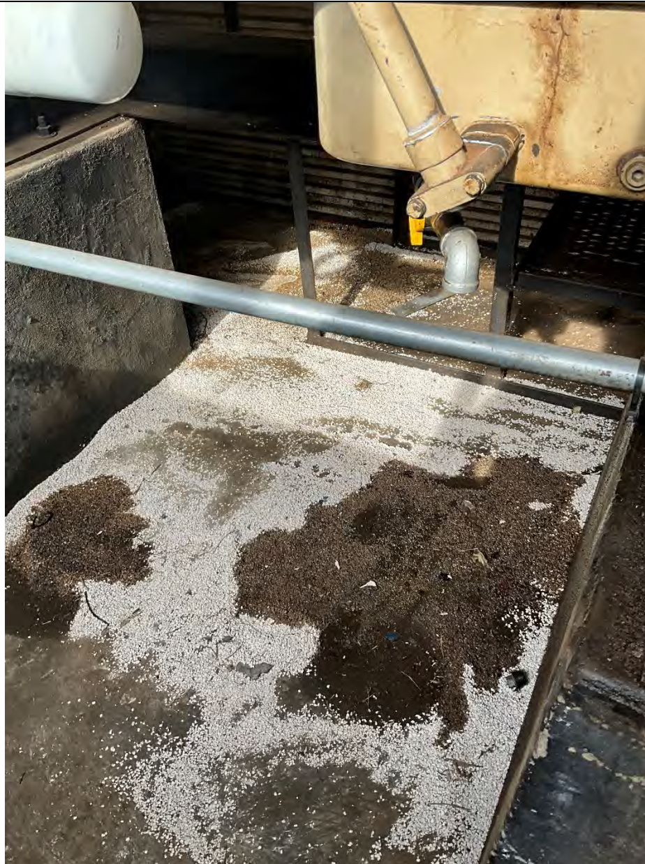
Well #1-7 – oil spilled on the floor of the well building below the natural gas-powered generator.
