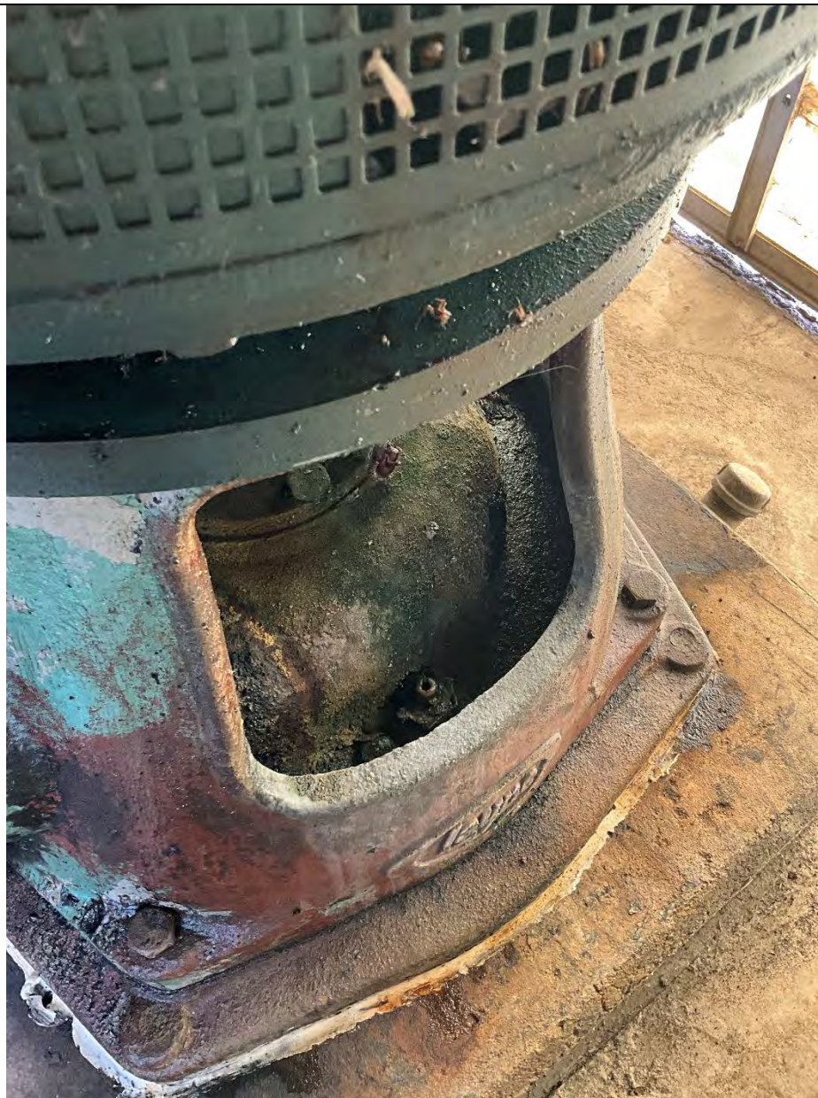
Well #3-3 without a casing vent
