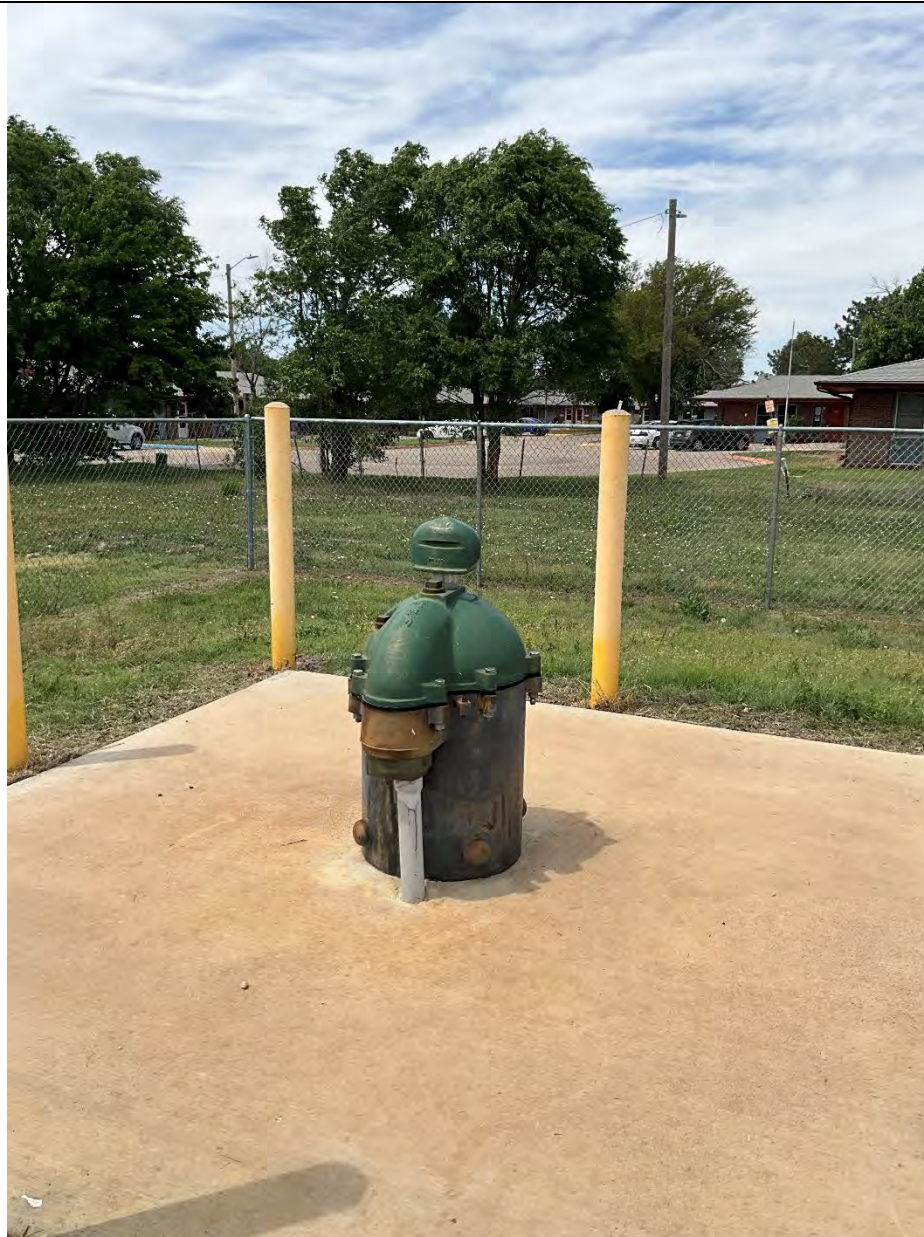
Well #35 – submersible pump with physical barriers
