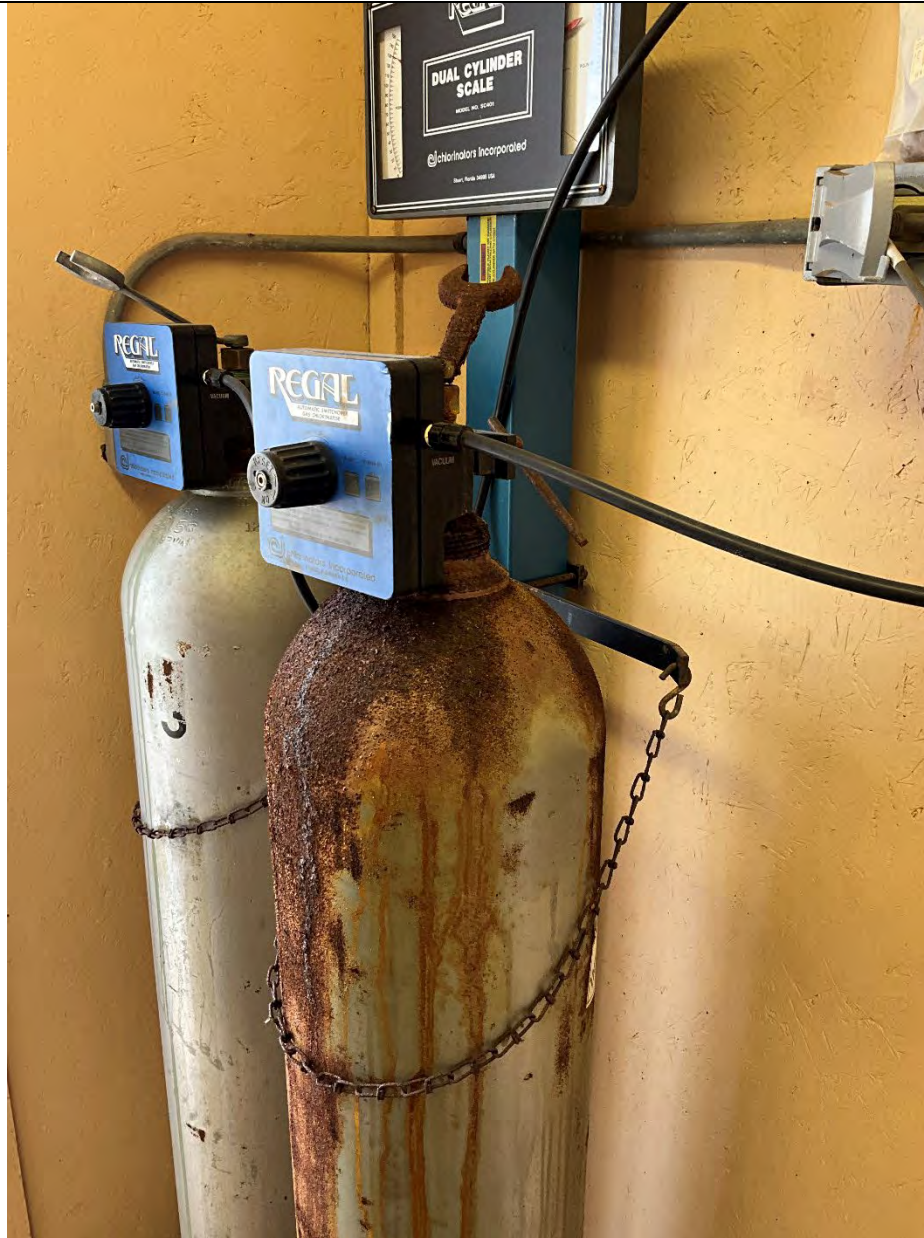
Well #63 – gas chlorine cylinders with heavy corrosion due to cylinder leak
