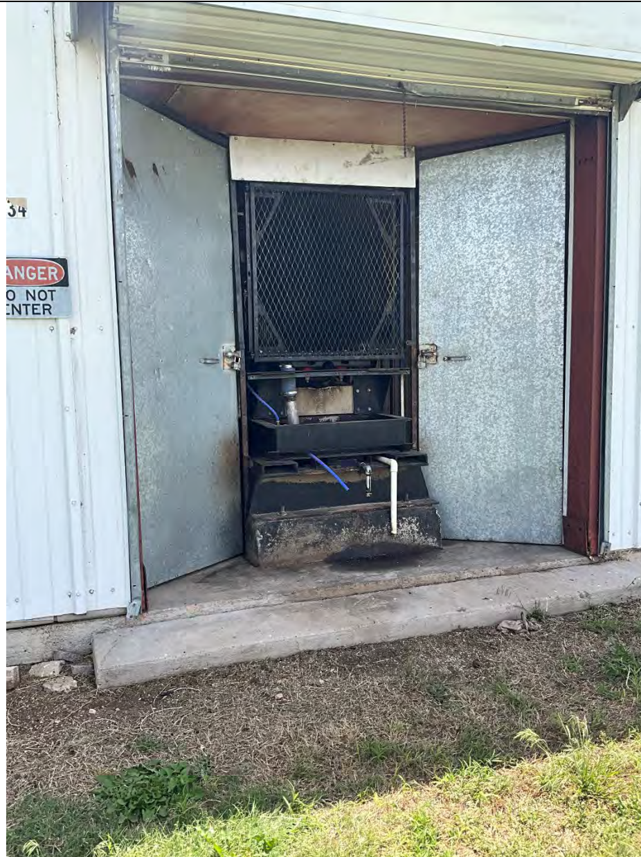
Well #34 – drains for lubricants and antifreeze for the natural gas powered pump
