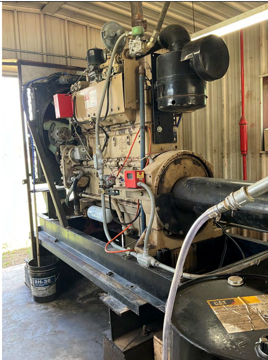
Well #34 – natural gas powered pump.
