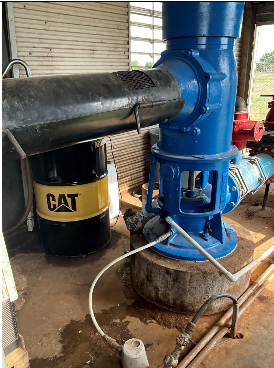
Well #1-7 – well pump connected to the natural gas generator; note the 55-gallon drum of oil near the well base.
