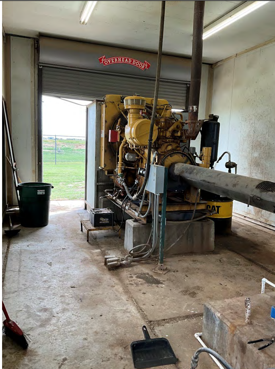
Well #2-9 view of second natural gas powered pump; note the 55-gallon barrel of oil near well pump base.
