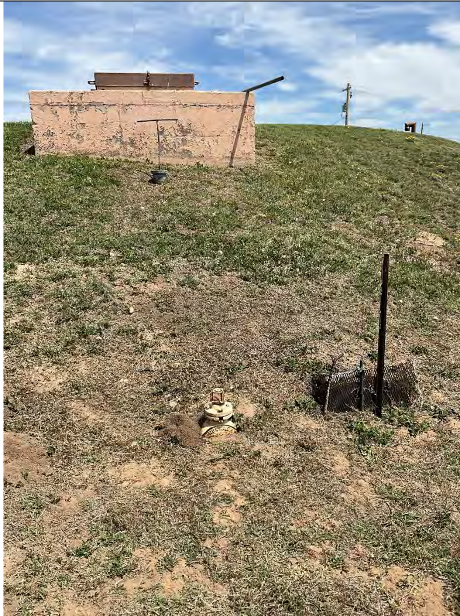
Station #3 – Ground storage tank concrete access hatch, drain valve, and drain location.
