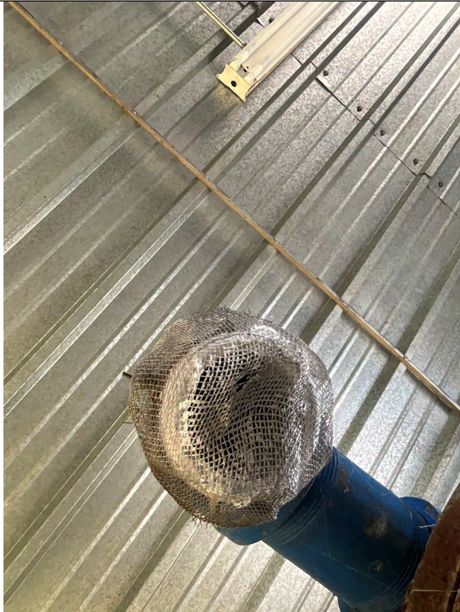
Well #3-3 – pressure relief valve discharge point with tears in the screen.
