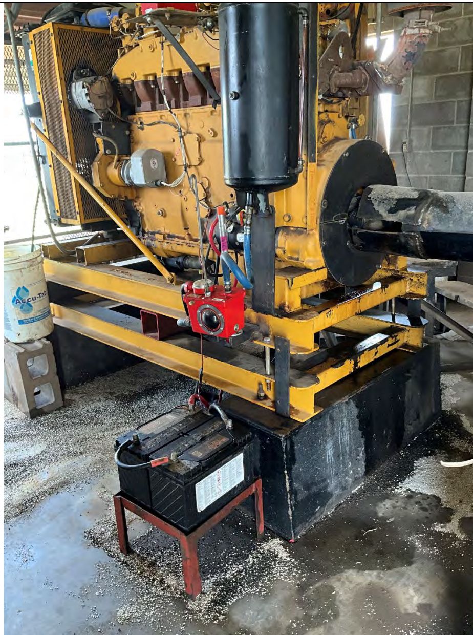
Well #2-7 – natural gas powered generate with oil spill on the floor adjacent to the pump base.
