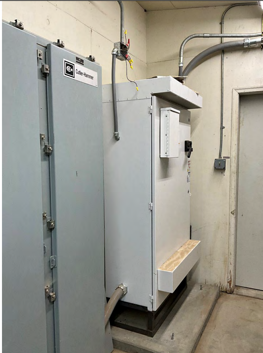
Well #53 – uncovered electrical junction box from the variable frequency drive (VFD) panel
