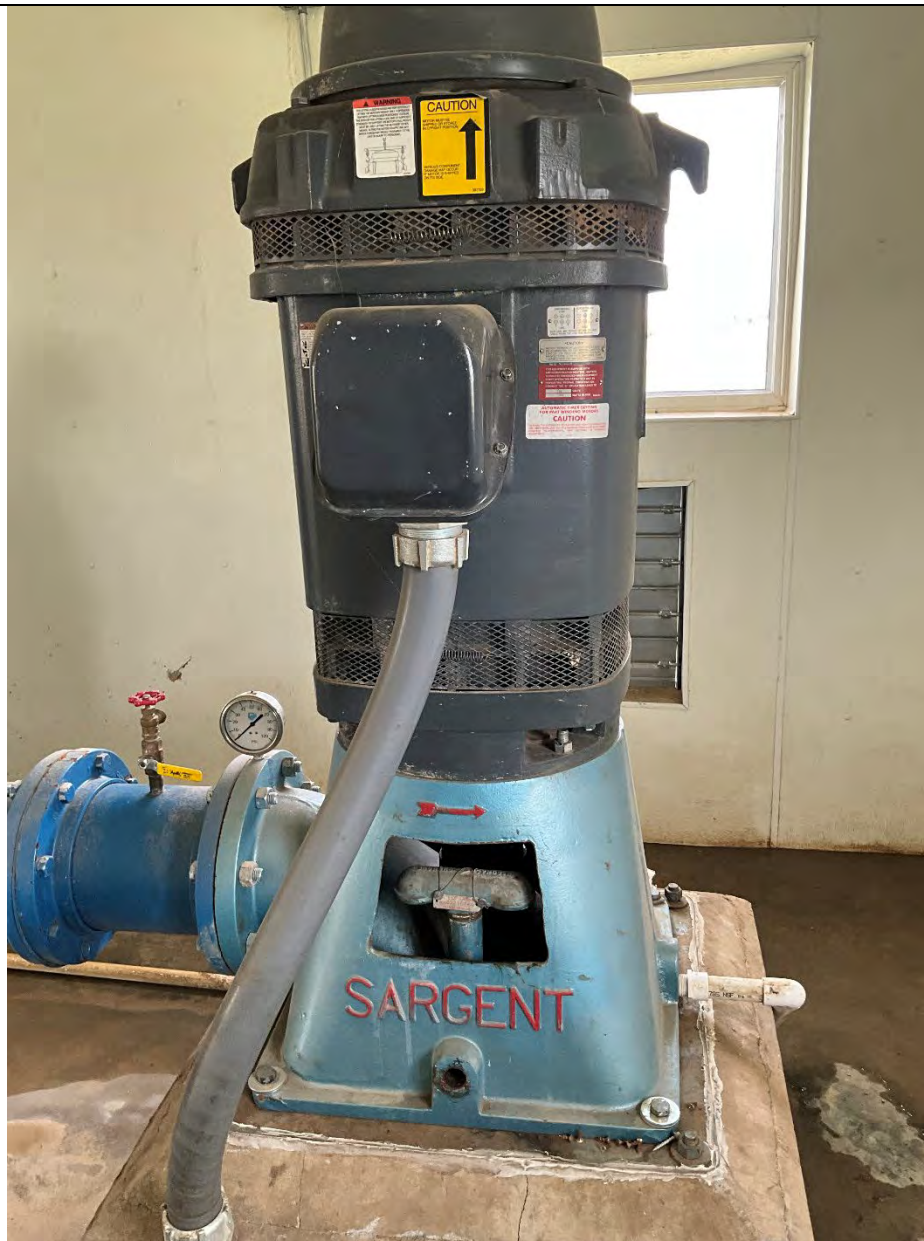
Well #45 – casing vent extended and downturned (large mesh screen not pictured), pressure gauge, packing drain tube, and well components.
