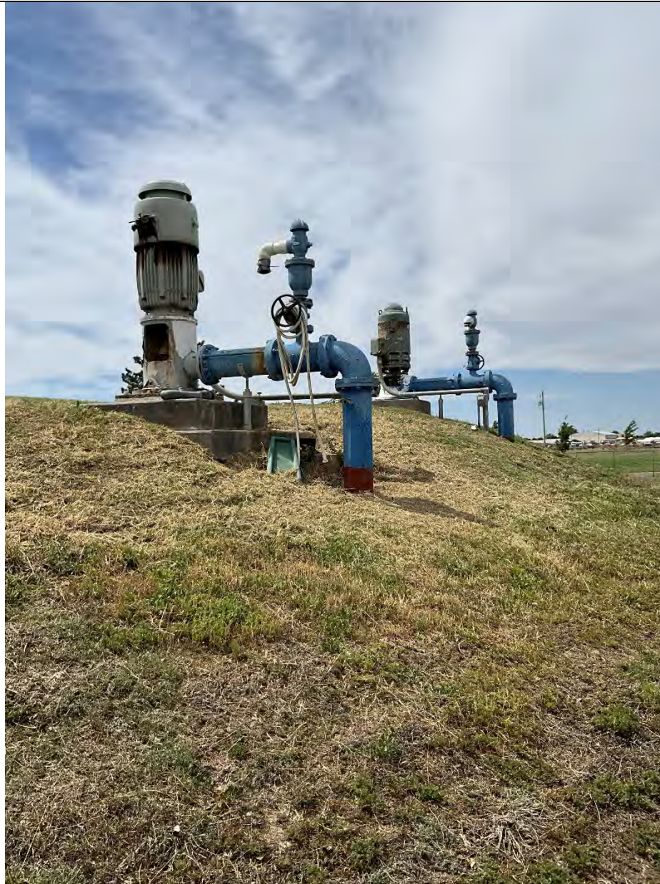
Station #2 – two electric high service pumps from the GST.
