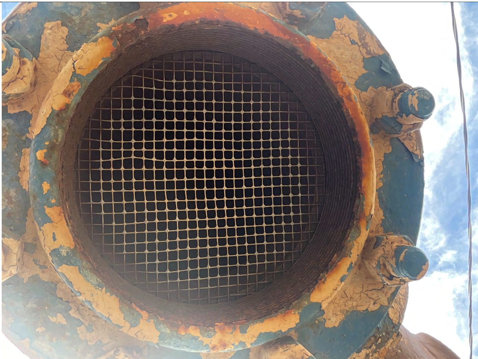
Station #4 – ground storage tank vent with large mesh screen (~4 mesh)
