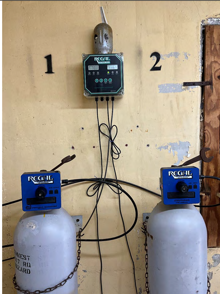
Station #4 – chlorine gas cylinders with automatic switch over valves, valve wrenches in place, and digital scale monitor measuring cylinder weight to record usage.
