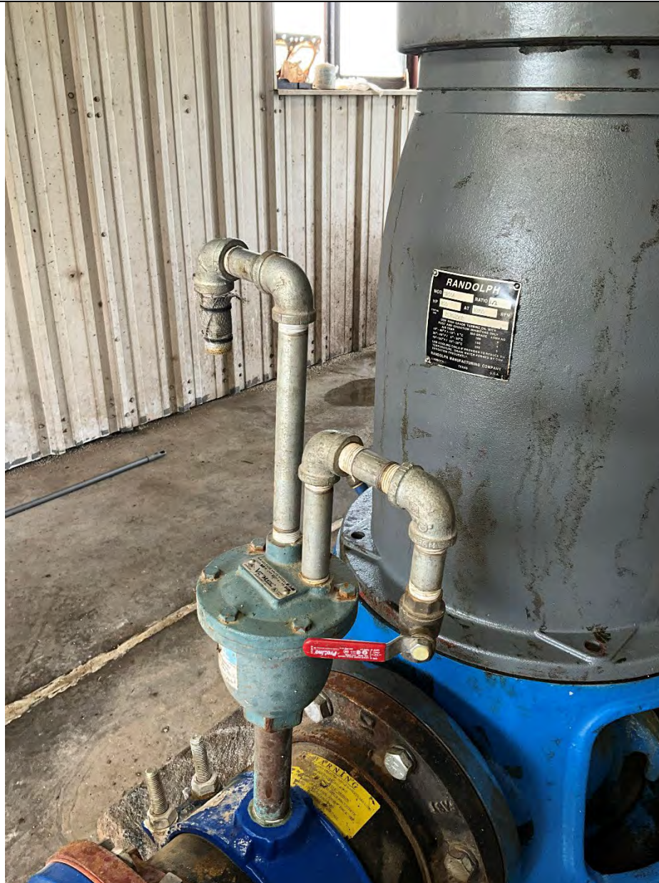
Well #34 – pressure relief valves with screened discharge point.
