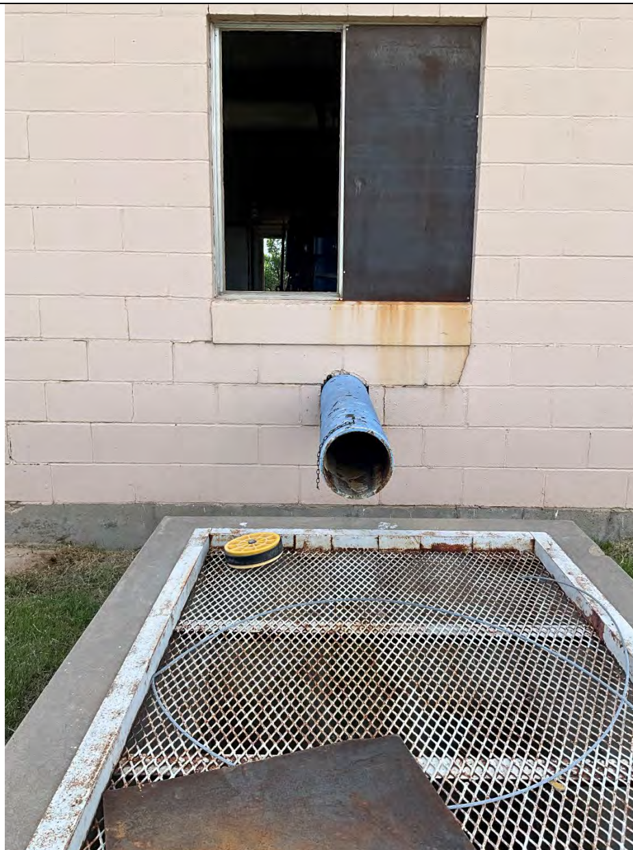
Well #2-7 – discharge pipe with cap for pump to waste if necessary
