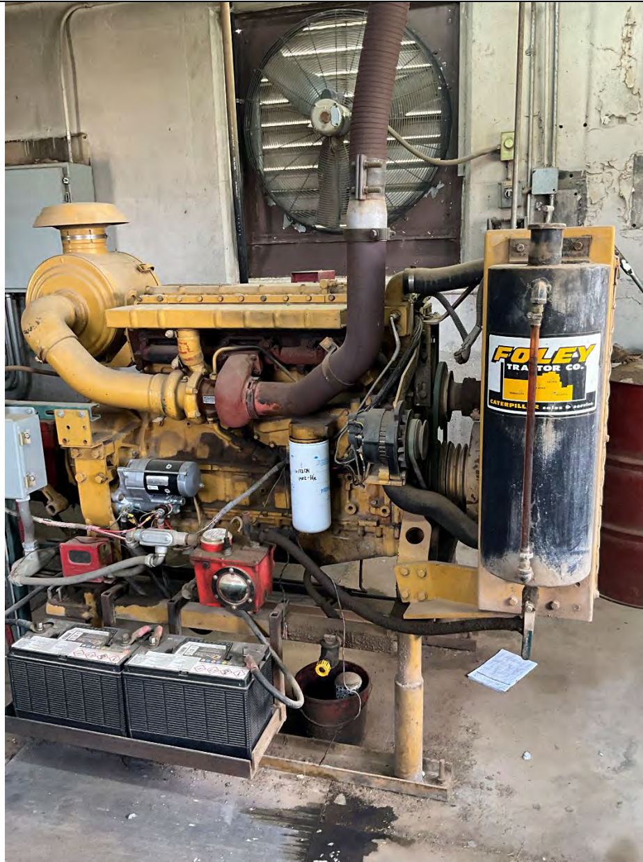
Station #3 – Diesel powered pump
