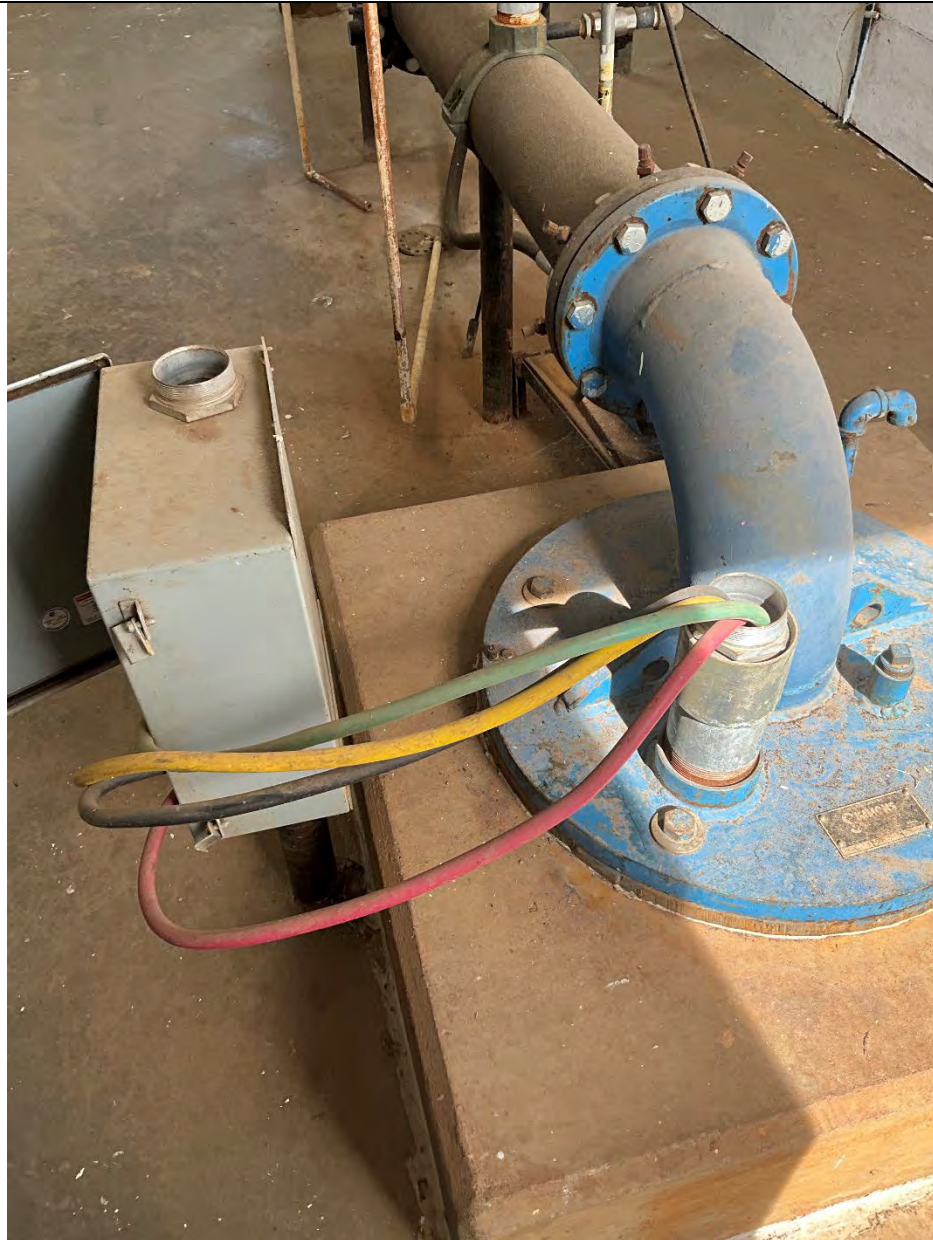
Well #62 – submersible pump electrical wiring without conduit from the junction box to the well casing.
