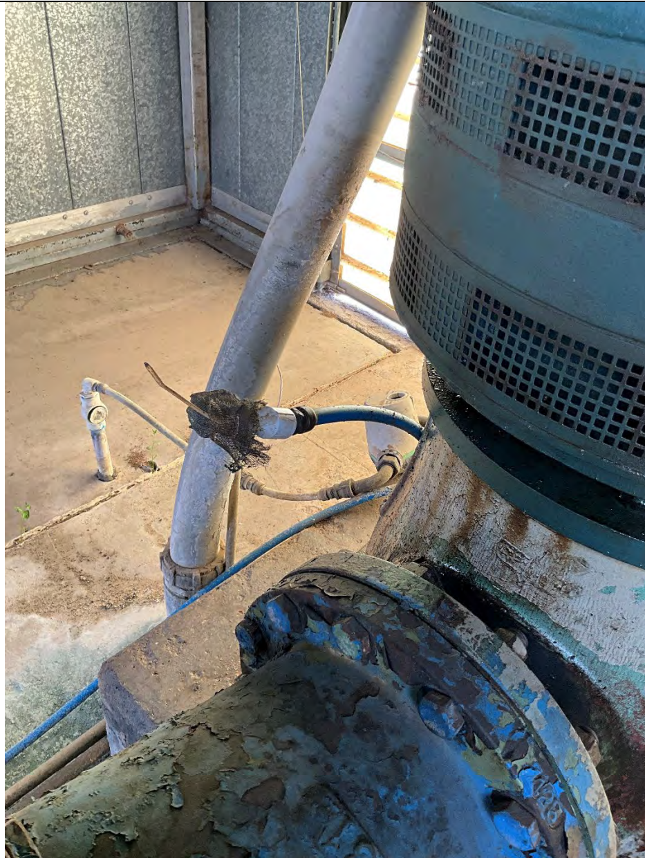
Well #3-3 drawdown tube extended and screened; however, facing outward and not downturned
