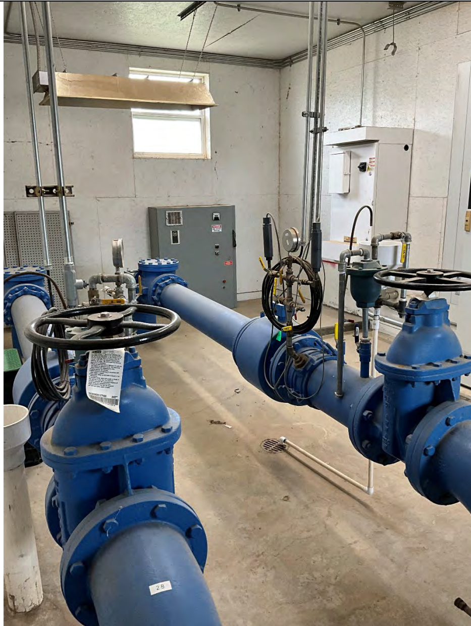
Station #2 – pump building interior
