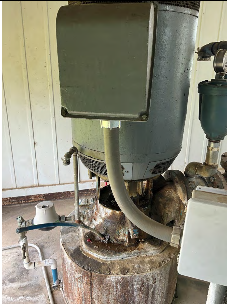
Well #43 – view of well pump on concrete base with casing vent screened, extended, and downturned; Draw down tube screened; also pressure relief valve and discharge point screened.
