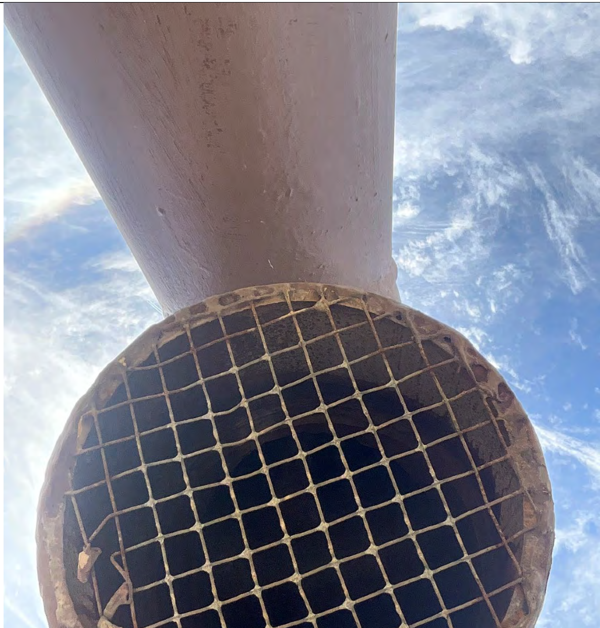
Station #3 – Ground storage tank vent screen with large mesh (4 mesh)
