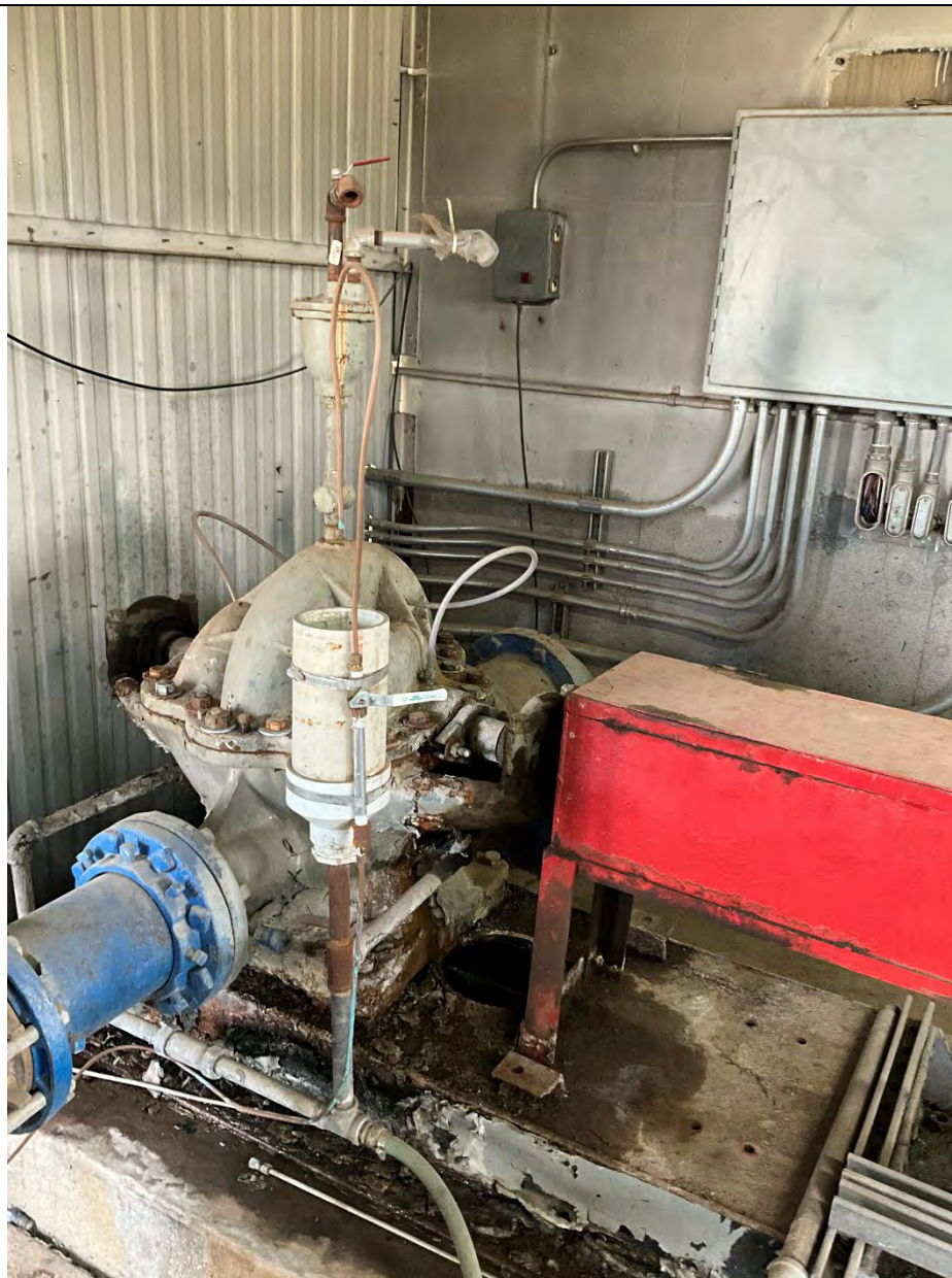
Station #3 – split casing pump and components
