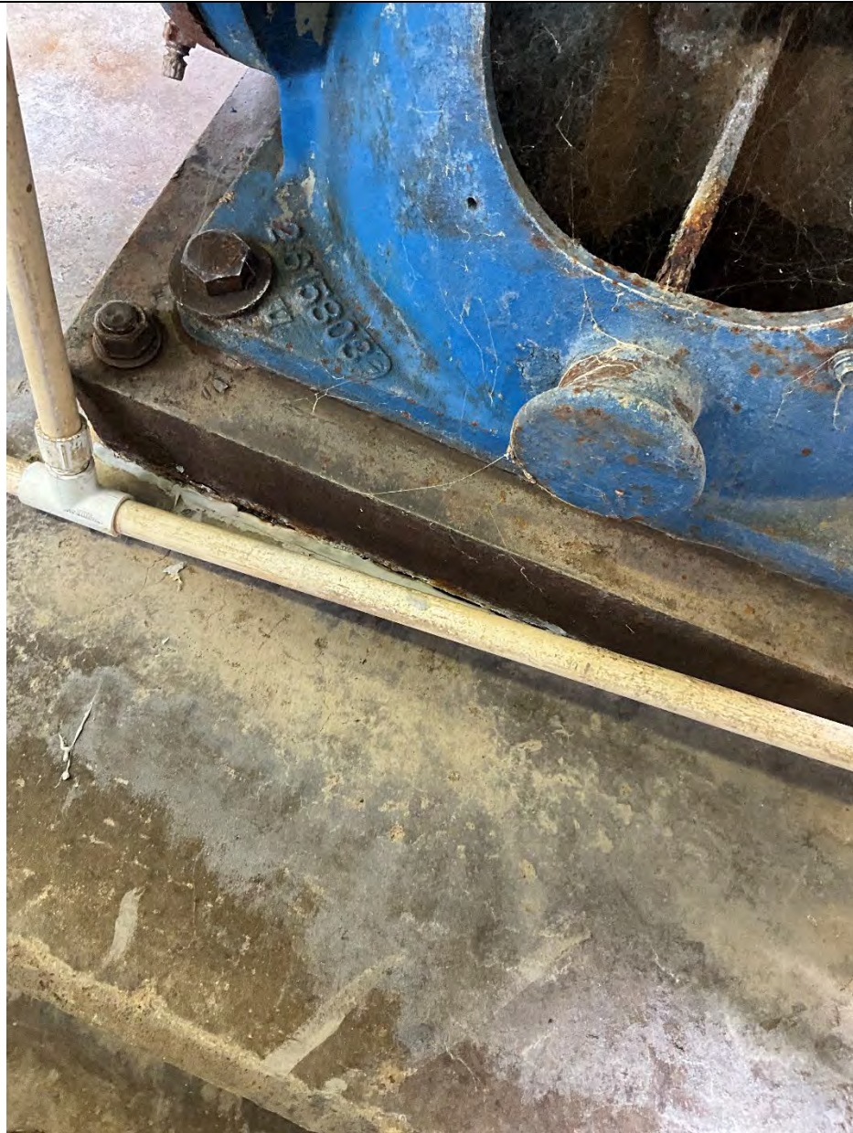
Well #1-1 - gap in sanitary seal between well pump and well base
