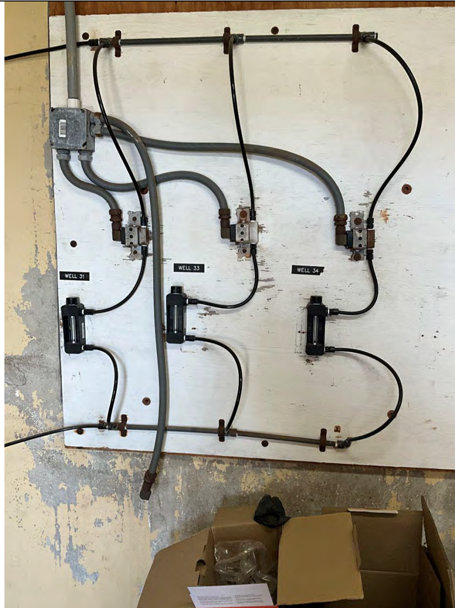
Station #3 – chlorine gas feed adjustment mechanism for each source water line
