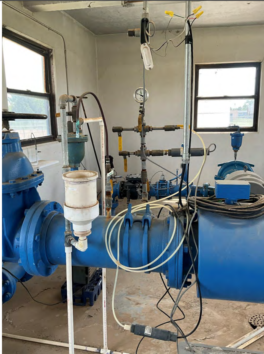
Station #3 – electrical pumps, plumbing components, and sample location
