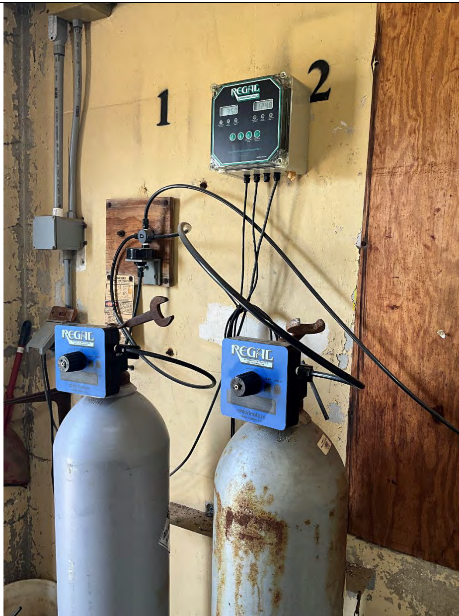
Station #3 – gas chlorine cylinders with auto switch valves, valve wrenches, and digital scale monitor
