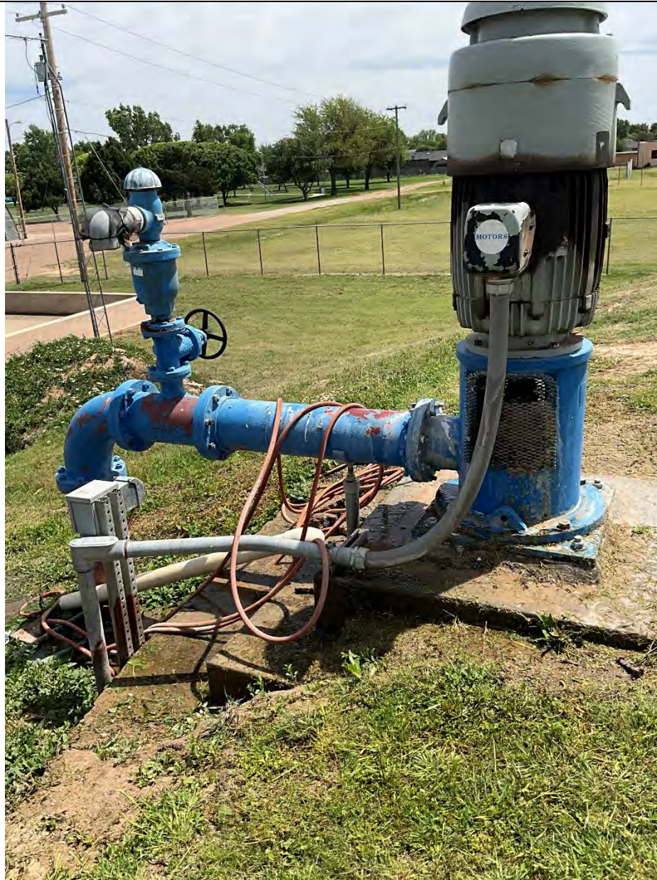
Station #3 – High Service Pump – packing leak
