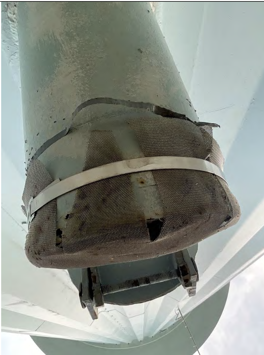
Water tower overflow screen with tears in the bottom of the screen
