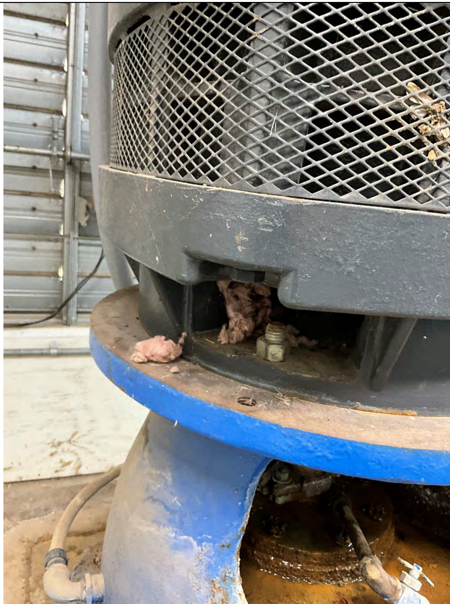
Well #53 – mouse nest in the electrical pump
