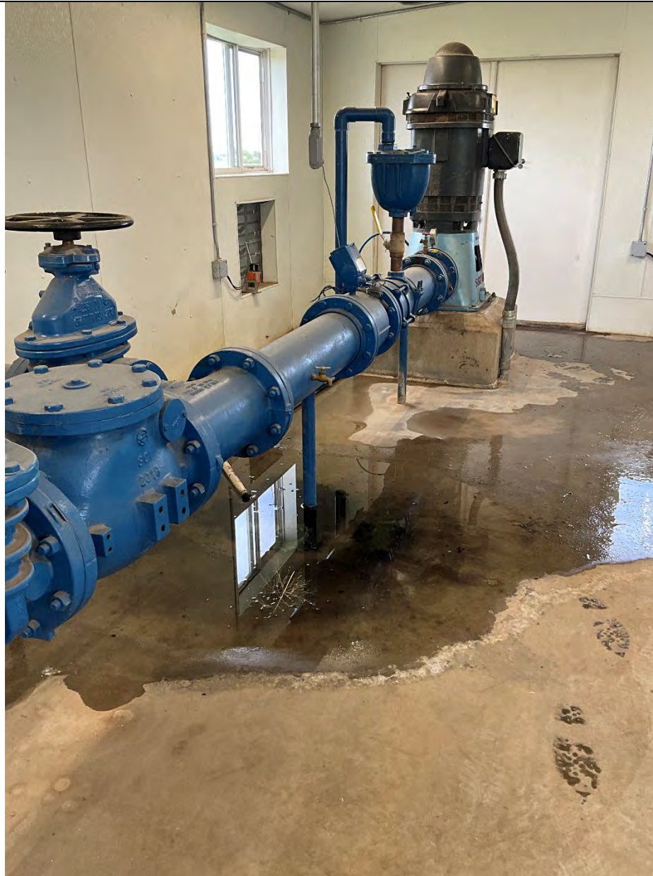
Well #45 – view of discharge line with pressure relief valve and isolation valve; Note the floor drain is clogged and water accumulation on the floor.
