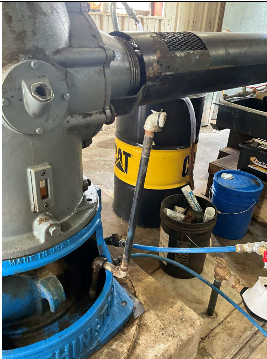
Well #34 – well casing vent extended but pointing outward; Also note the 55-gallon drum of lubricating oil near the pump base.
