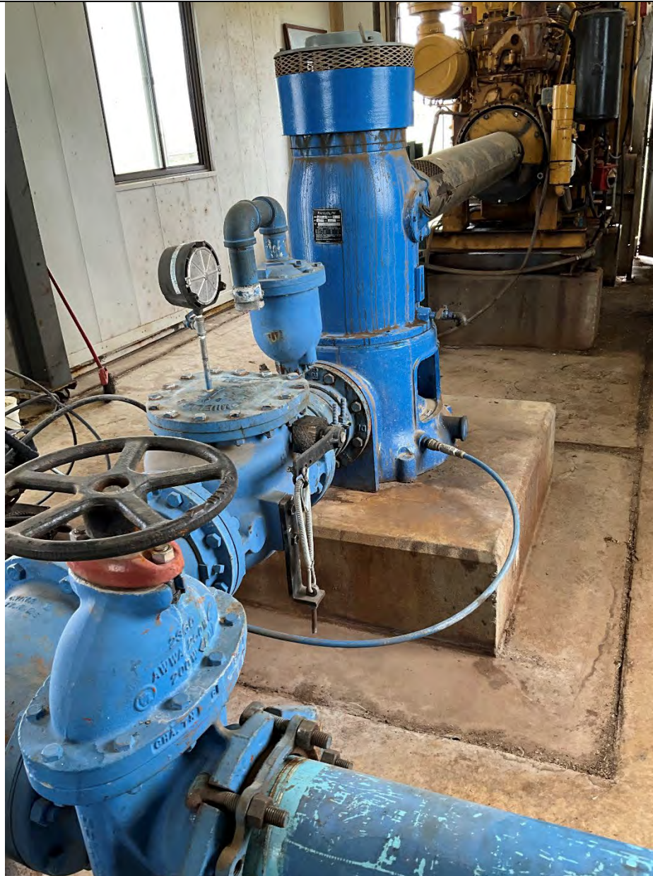
View of Well #2-9 casing lubrication line, pressure relief valve screened discharge point, check valve, isolation valve, and natural gas powered generator in the background.
