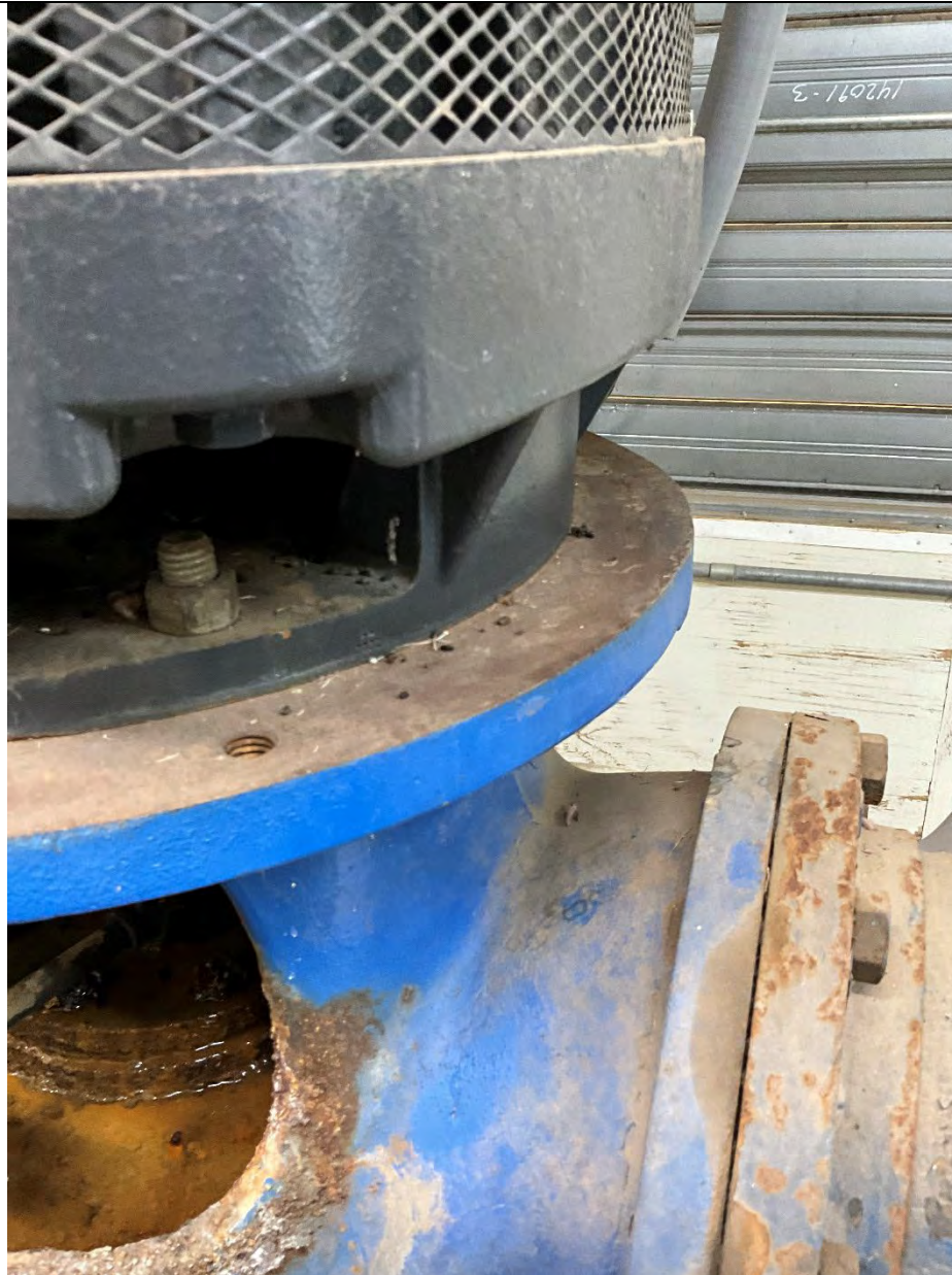
Well #53 – mouse droppings on the well pump
