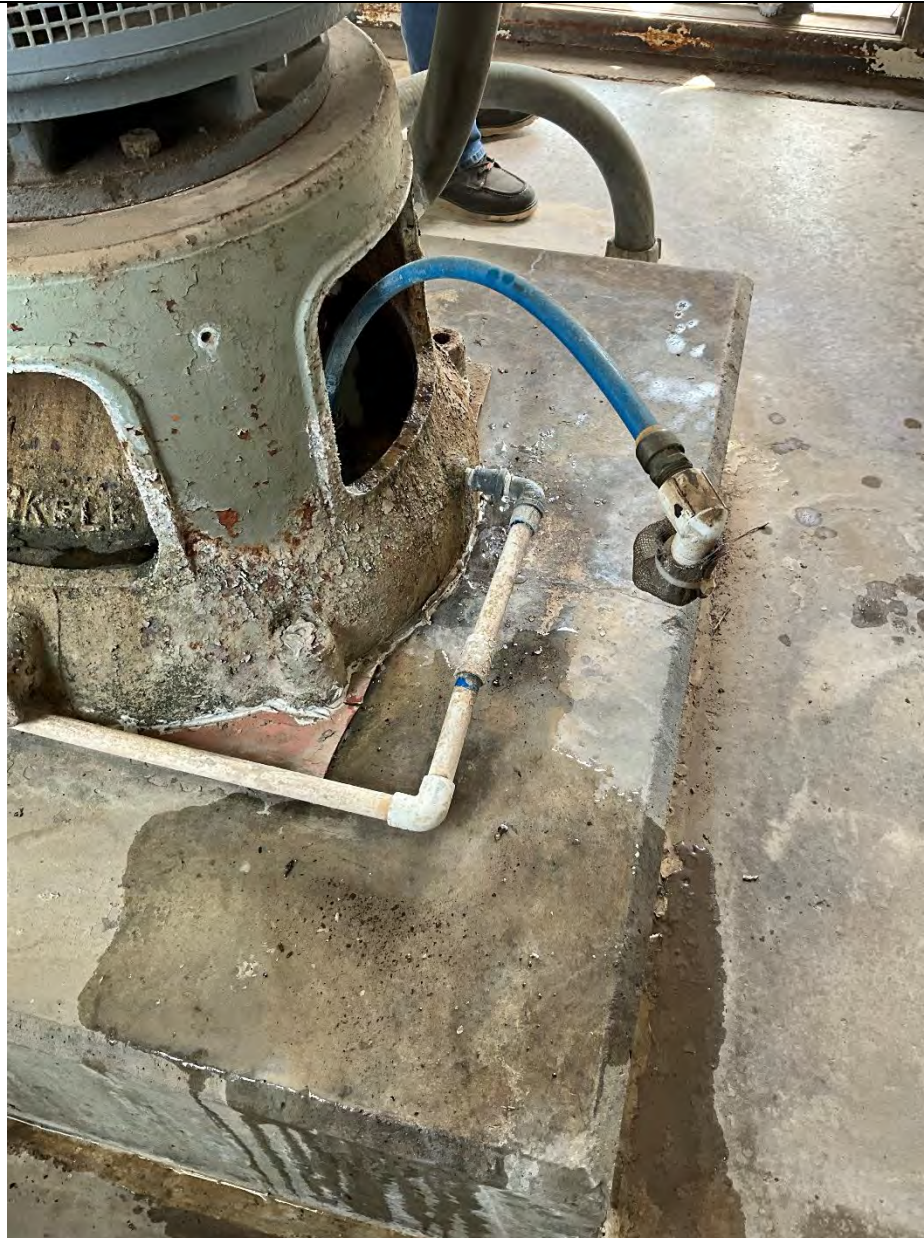
Well # 2-7 – well pump base with drawdown tube / casing vent assembly screened.
