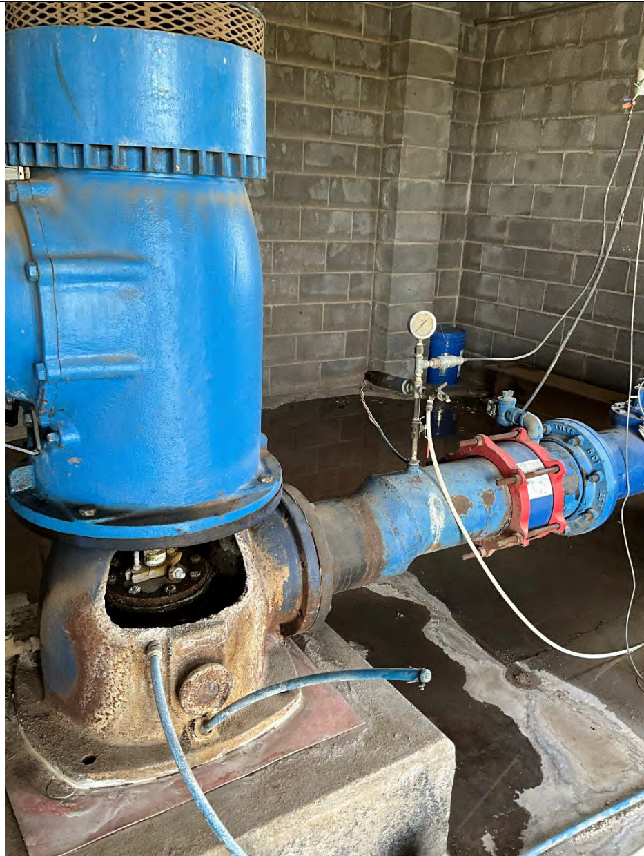
Well #2-7 – floor drain clogged and water accumulating on the floor of the building
