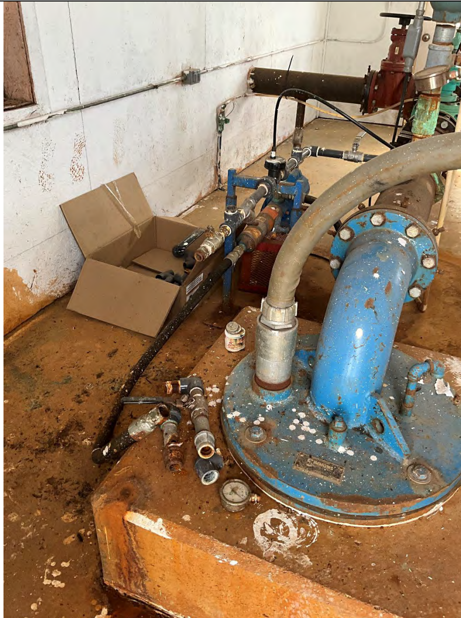
Well #63 – well out of service due to chlorine injection pump repair
