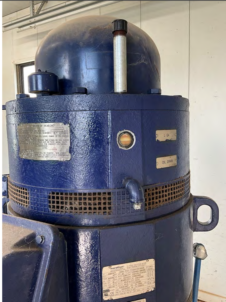
Well #44 – well head with lubrication level indicator
