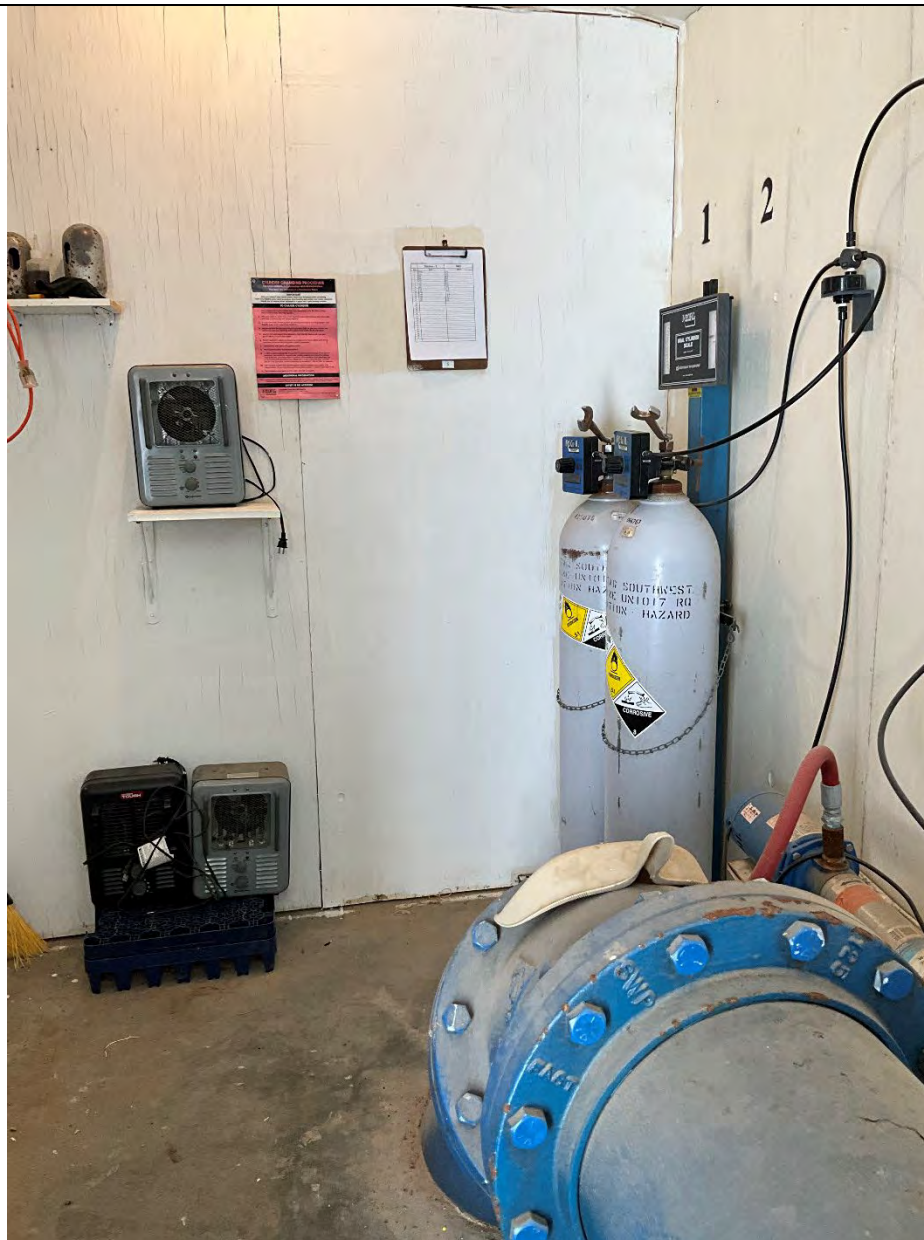
Station #5 gas chlorine tanks and interior of the pump building
