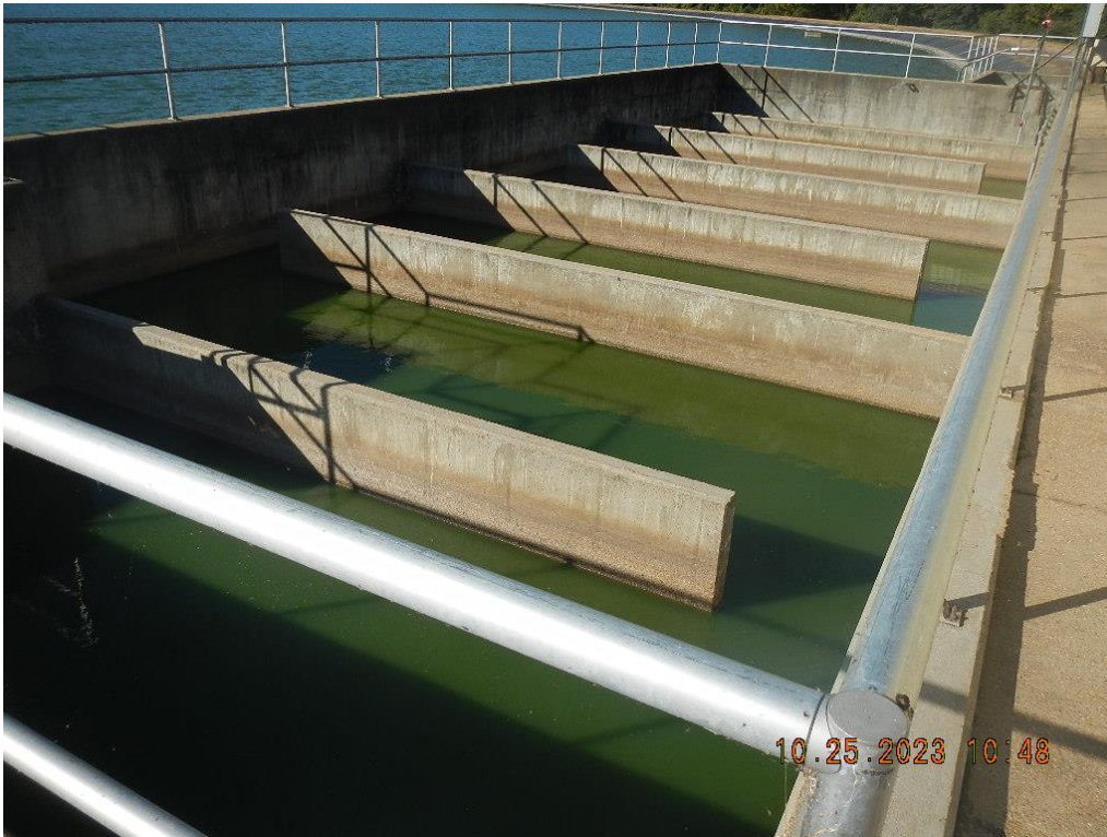
Photo 2. Green algae observed in the chlorine contact chamber.
