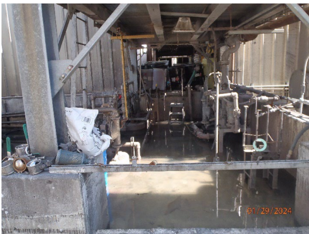
Picture 26 – Tank System 1 Pumphouse secondary containment flooded with rainwater
