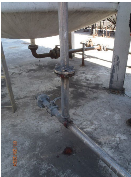
Picture 20 – Tank System 1 Tank B7 flange leak
