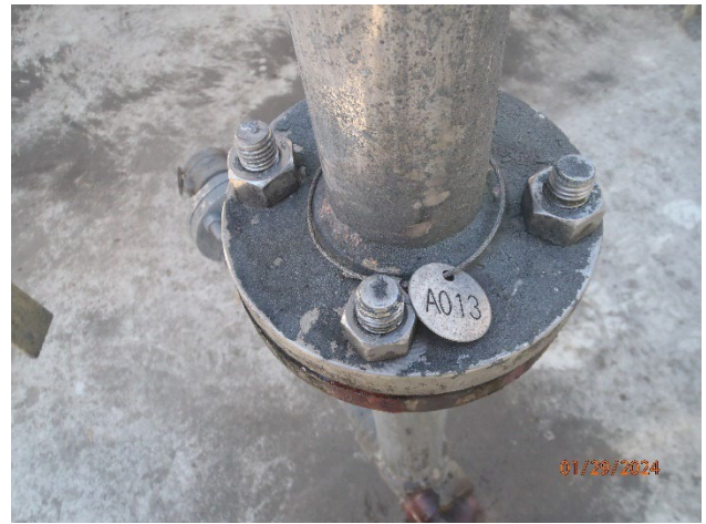
Picture 22 – Tank System 1 Tank B7 flange A013 leaking
