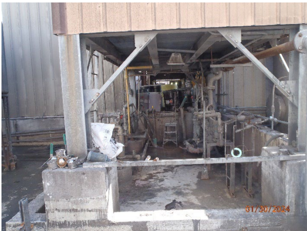
Picture 27 – Tank System 1 Pumphouse secondary containment pumped out
