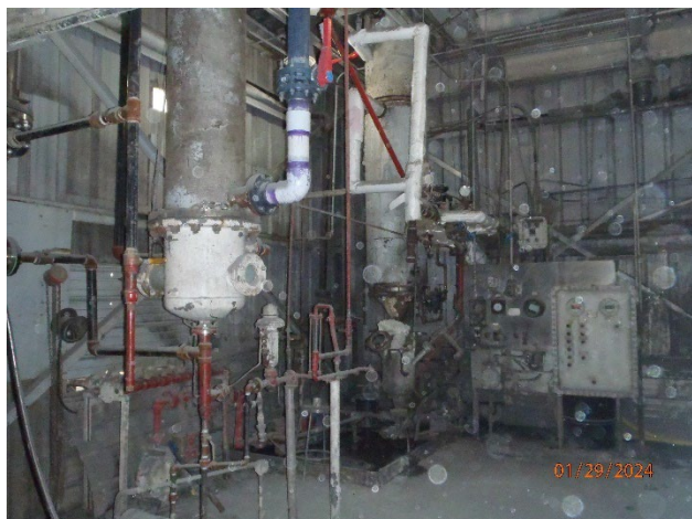
Picture 48 – LUWA thin film solvent recovery system
