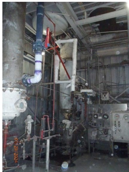
Picture 49 – LUWA thin film solvent recovery system
