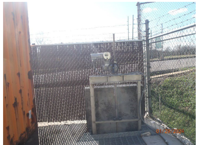
Picture 5 – Inbound Staging Area gate valve to outfall
