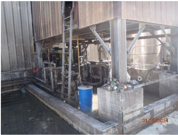
Picture 25 – Tank System 1 Pumphouse
