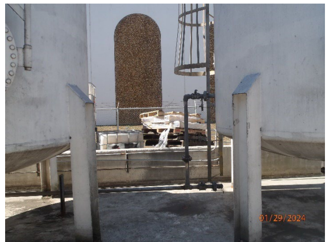
Picture 23 – Tank System 1 Tank B7 flange leak
