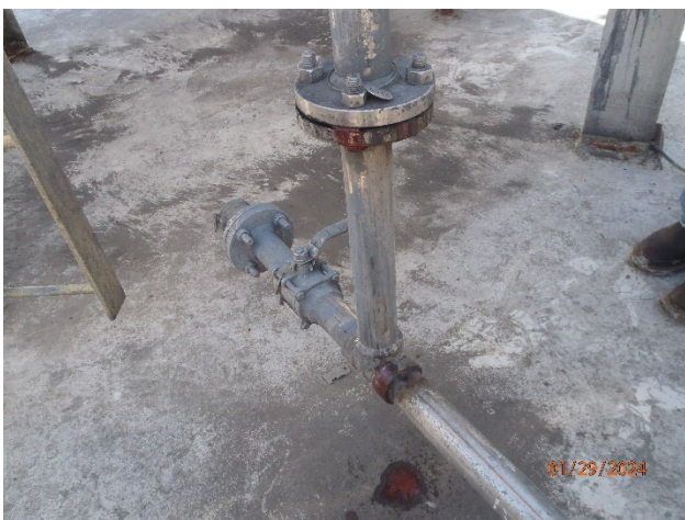
Picture 21 – Tank System 1 Tank B7 flange leak
