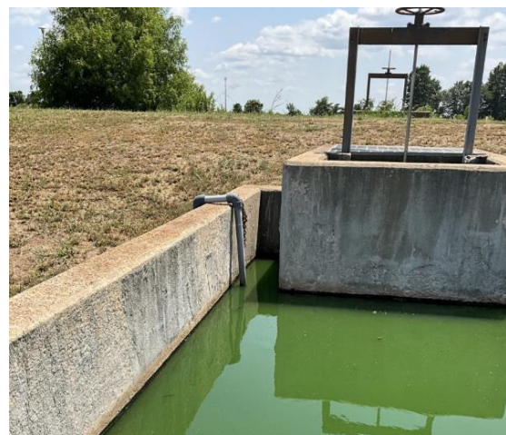
Photo 4: Chlorine Gas injection location
