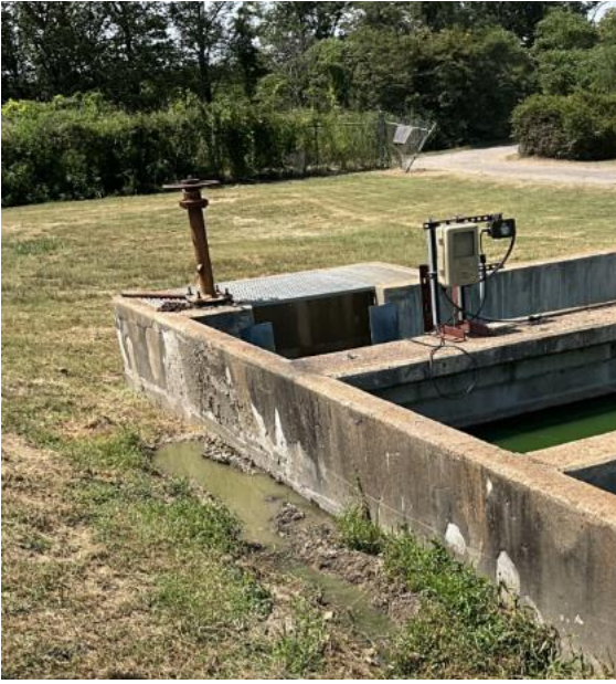
Photo 5: Leak in the Chlorine contact chamber wall
