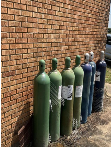
Photo 1: Gas chlorine cylinders
