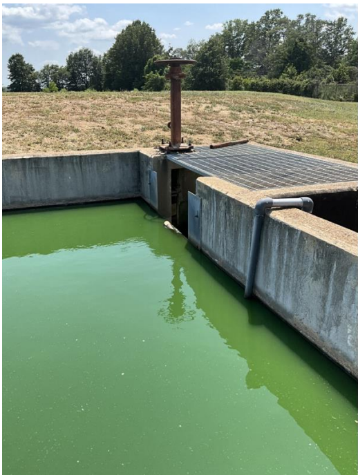
Photo 3: Sulfur Dioxide injection location and Weir
