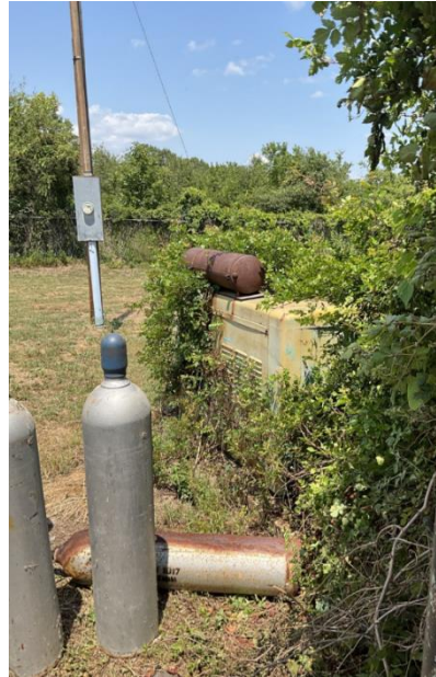
Photo 2: Gas chlorine cylinders exposed to the environment.
