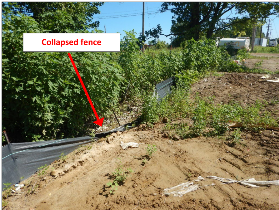
Photograph 24. View, facing southeast, of a collapsed silt fence along the Site's eastern boundary.
