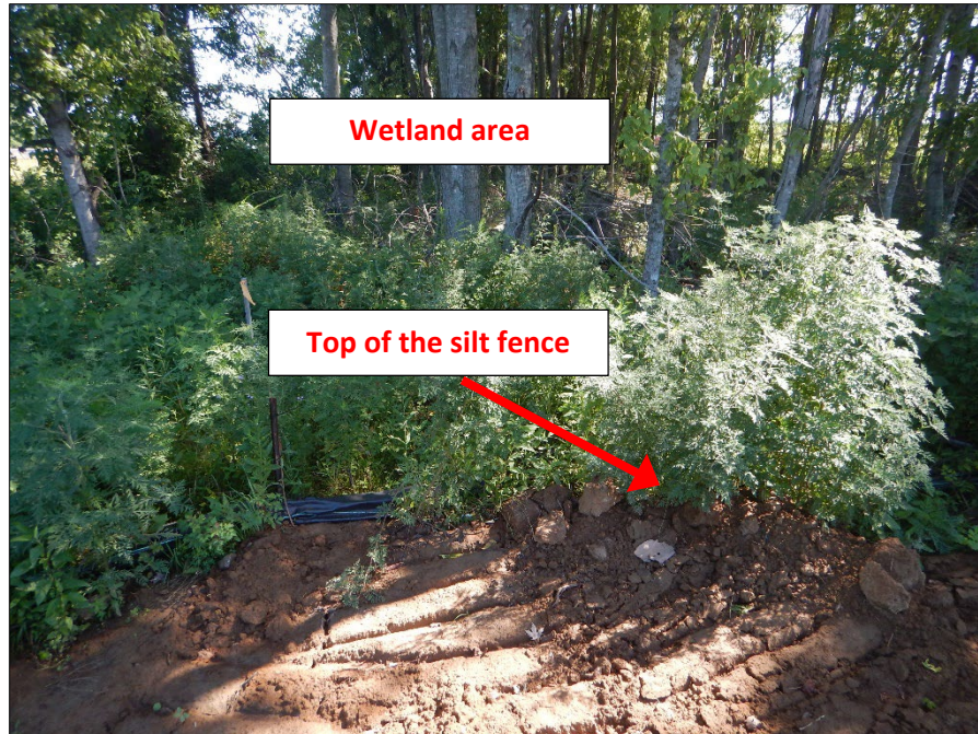
Photograph 21. View, facing northeast, of sediment accumulation to the height of the silt fence in the western portion of the Site.
