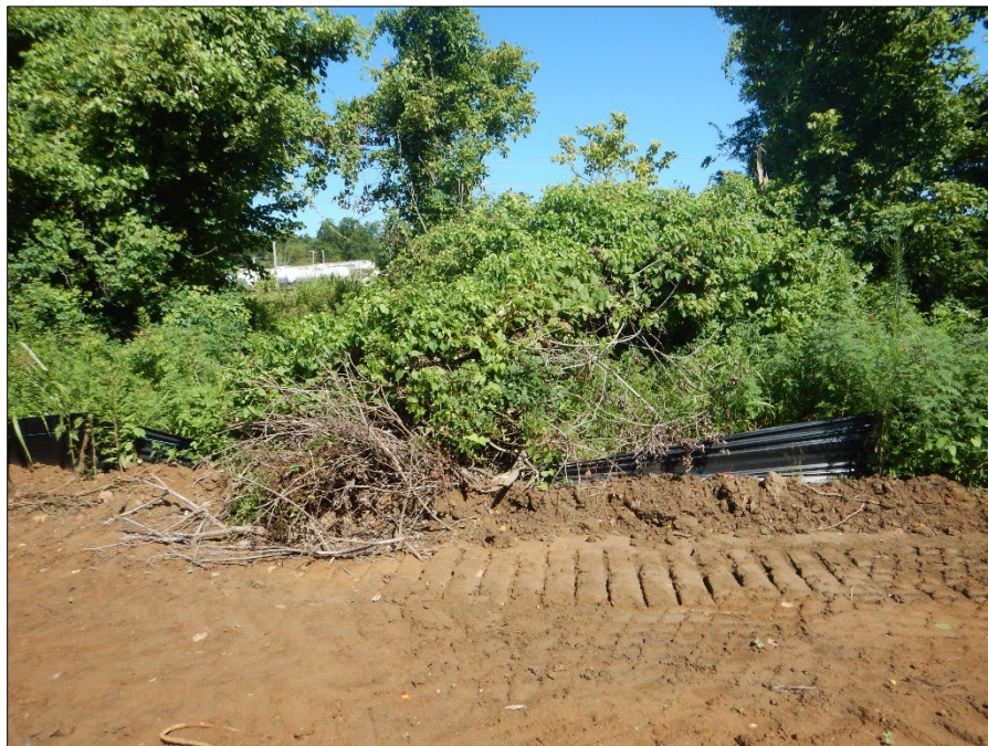
Photograph 20. View, facing east, of vegetation that had fallen and partially collapsed the silt fence on the eastern boundary of the Site.
