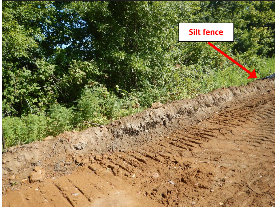
Photograph 19. View, facing north, of sediment accumulation overtopping the silt fence in the western portion of the Site.
