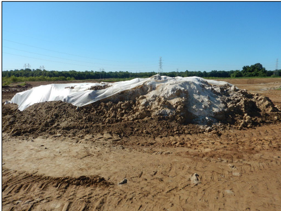
Photograph 2. View, facing south, of a partially covered pile of lime and dirt in the center of the Site without erosion or sediment controls.
