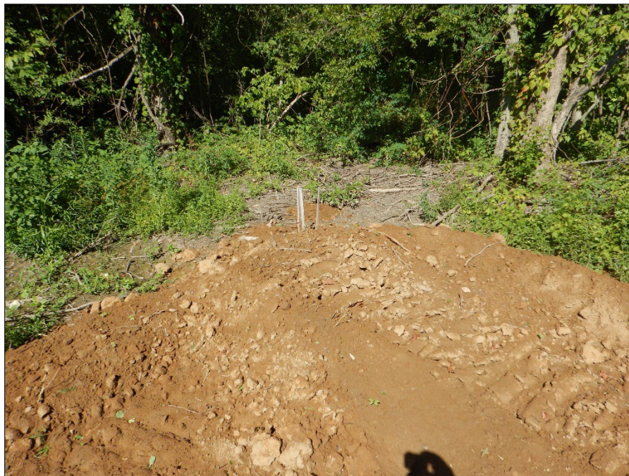
Photograph 18. View, facing west, of a lack of perimeter controls (e.g., silt fence) in the southwestern portion of the Site.
