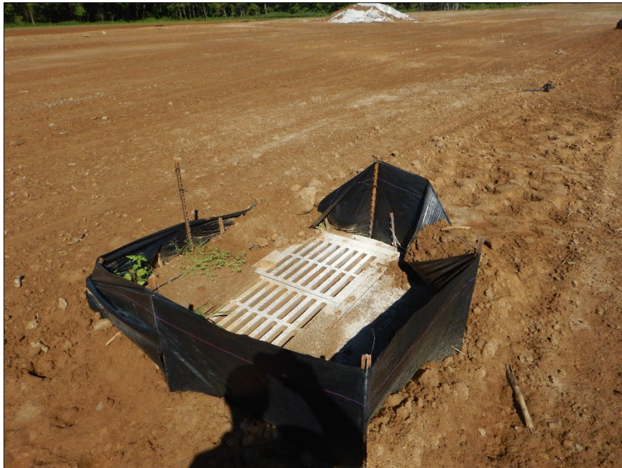
Photograph 8. View of an inlet in the center of the Site where sediment had been deposited over the silt fence inlet protection and into the inlet.
