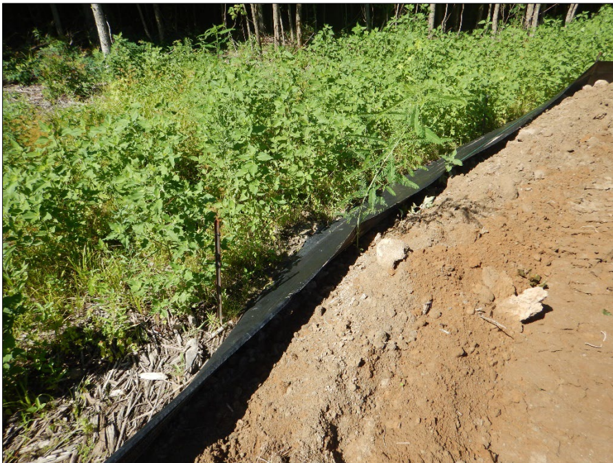
Photograph 16. View, facing south, of sediment accumulation against the silt fence in the southwestern portion of the Site. Silt fence in the area had separated from posts and required maintenance or reinstallation.
