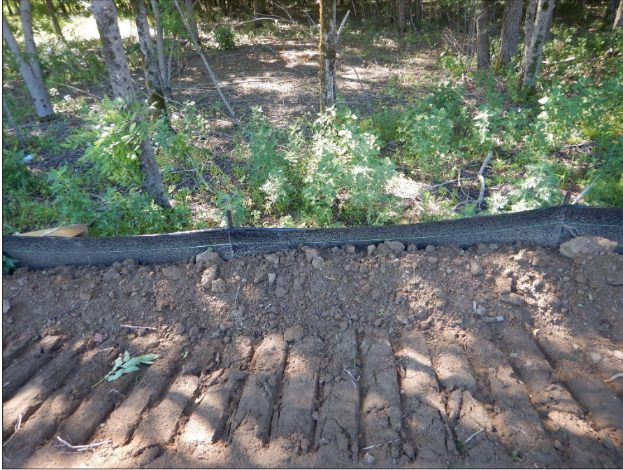
Photograph 15. View, facing southwest, of sediment accumulation against the silt fence along the Site's southern boundary. Sediment had accumulated to at least half the height of the silt fence.
