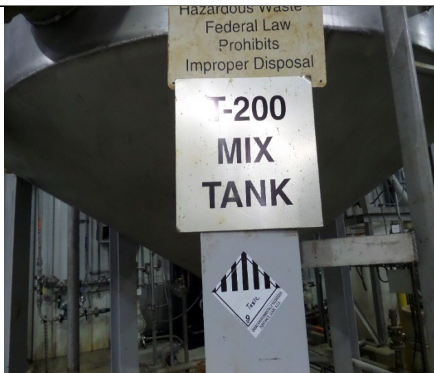
Leachate Treatment System. The inspector observed PSCT mark the T-200 Mix Tank with the word “toxic”. Photograph 14 taken at 10:59 a.m.
