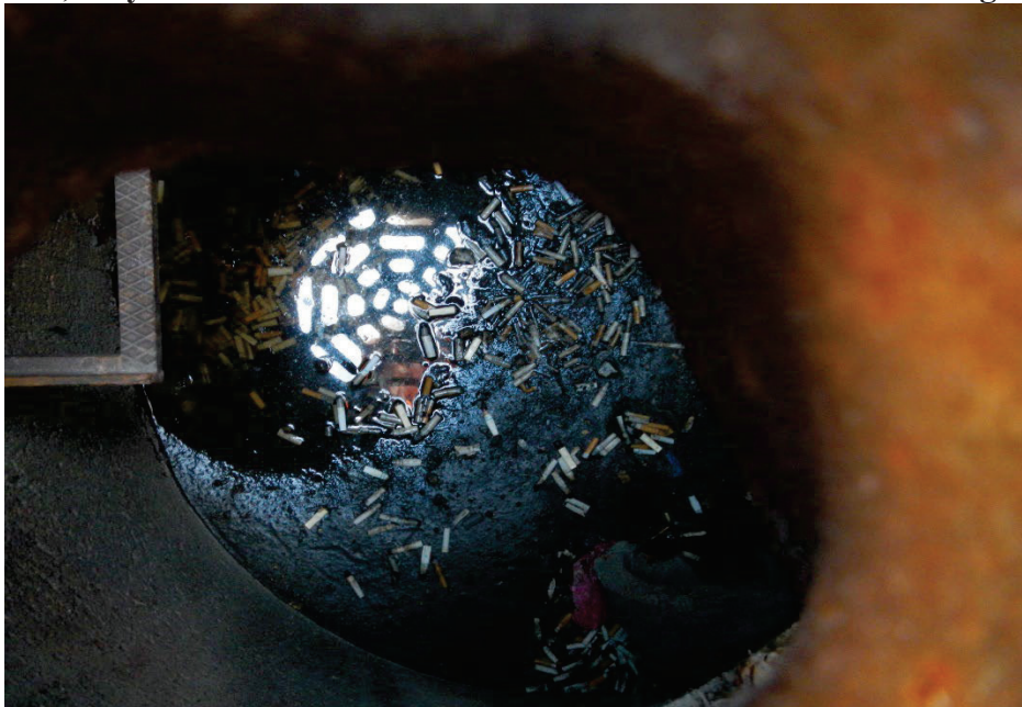
Photo 3, Oily Substance in the stormwater inlet at the Material Storage area
