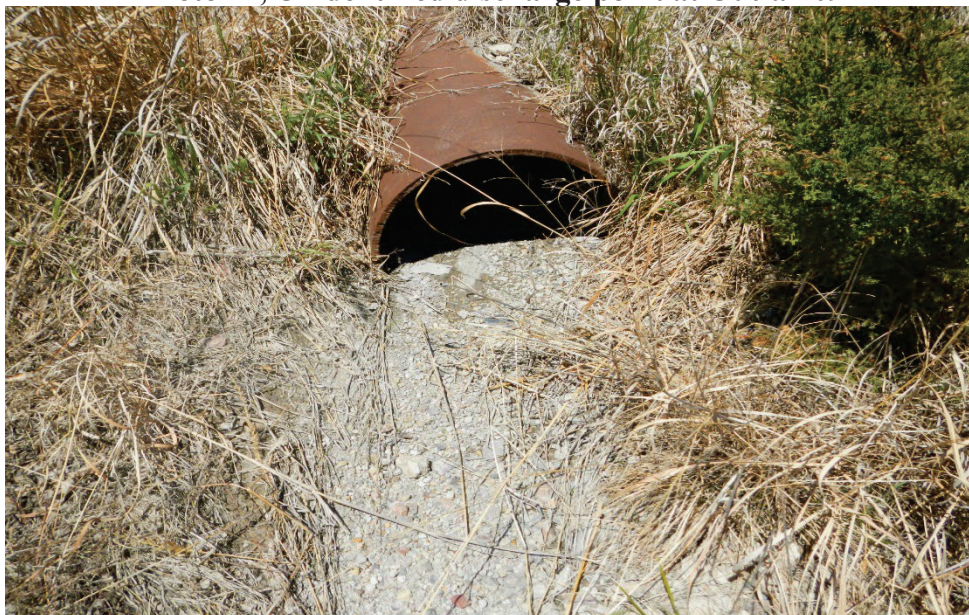
Photo 22, Unidentified discharge point at Outfall 09
