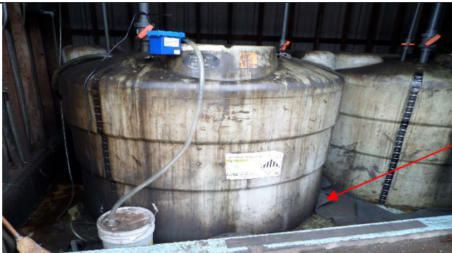
Photo-3 1,100-gallon tanks containing coolant water sludge in Secondary Containment System with leaks and spills
