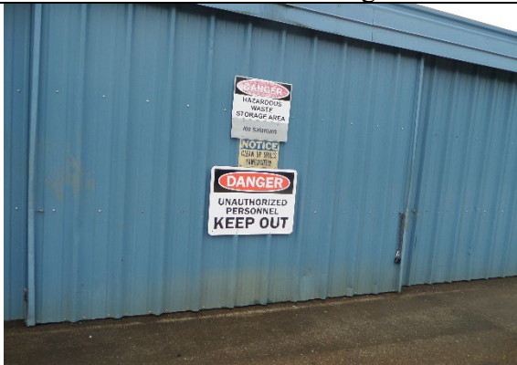
Photo-2 Hazardous Waste Storage Area
