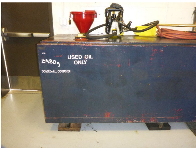
Photo 12: 480-gallon tank of used oil in the Building 4430 Vehicle Maintenance Area.
