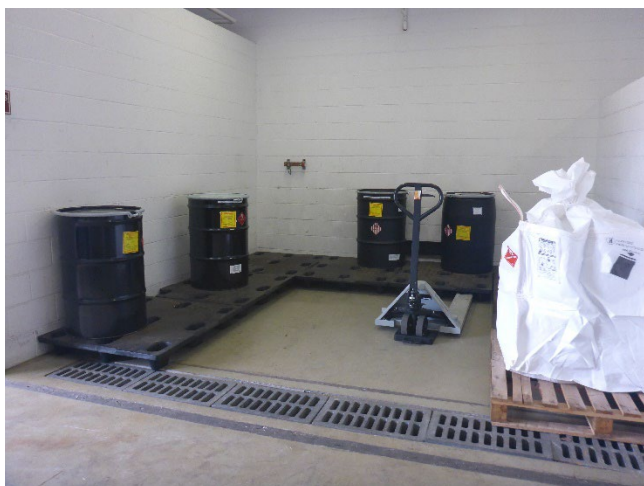
Photo 2: Four 55-gallon containers and one supersack of hazardous waste in the first bay within the CAA.
