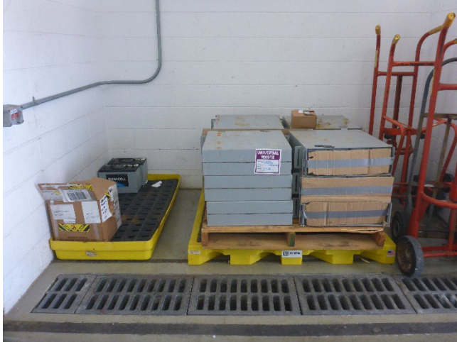
Photo 4: Two individual lead-acid batteries, one box of non-spillable batteries, and twelve battery slabs in the fourth bay within the CAA.
