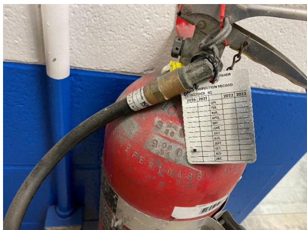
Photo 21: Fire Extinguisher recharged 10/2020.
