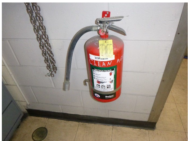
Photo 20: Fire Extinguisher recharged 11/2018.
