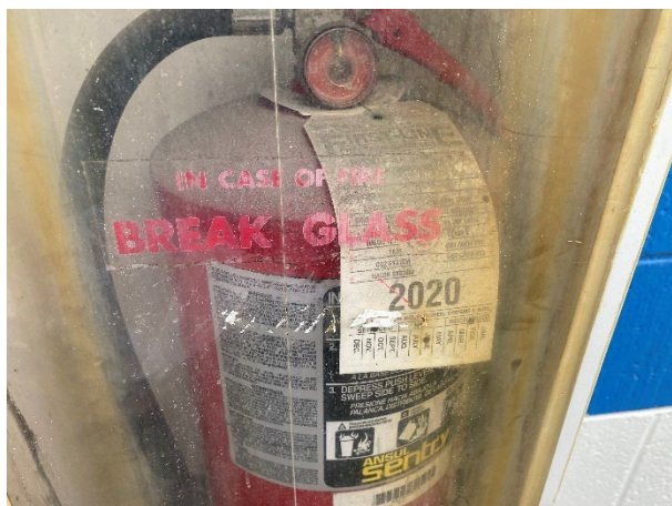
Photo 19: Fire Extinguisher recharged 6/2020.
