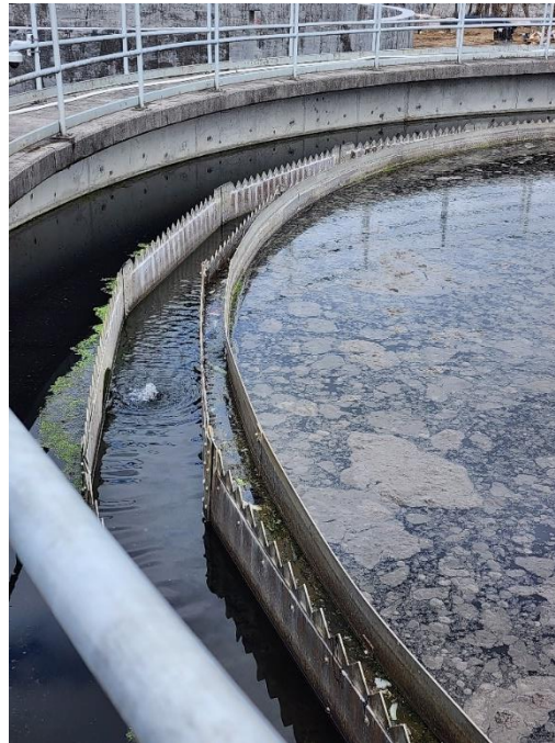
Photo 6: Unlevel floating weir in clarifier #1.
