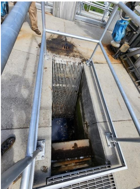
Photo 2: Secondary manual bar screen after cleaning.
