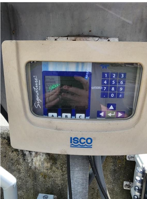
Photo 11: Effluent flow meter reading 7.5MGD.
