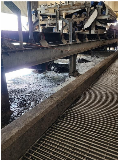
Photo 16: Sludge under belt press.
