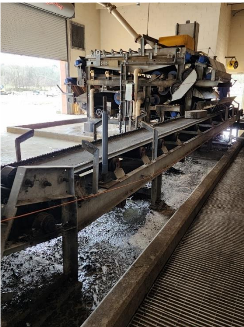
Photo 15: Belt press out of service.
