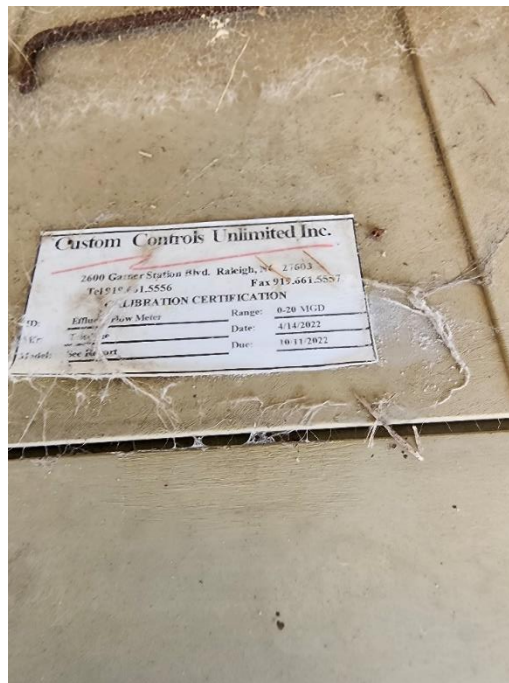
Photo 12: Effluent flow meter calibration sticker.
