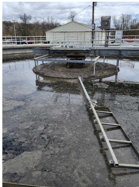
Photo 8: Center well of clarifier #1 full of solids.
