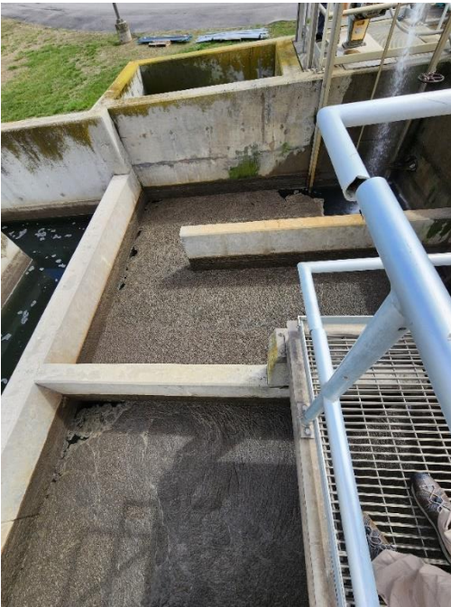
Photo 9: Floating sludge/foam in chlorine contact chamber front section.
