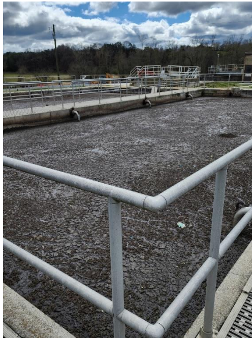
Photo 14: Sludge thickening in old aeration basin.
