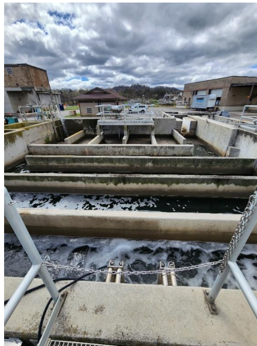
Photo 10: chlorine contact chamber full view.
