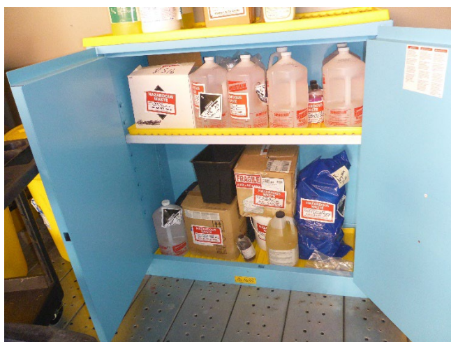
Photo 29: Two shelves holding containers of waste corrosive liquids. Each container appeared to be labeled with the words "Hazardous Waste", identified with an indication that its contents are corrosive, and marked with an accumulation start date.
