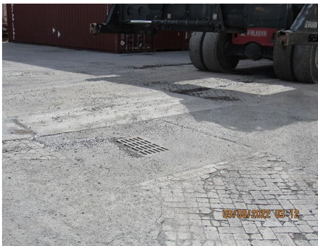
IMG 518 -Stormwater catch basin that drains entire area of Tropical's MT Yard. Inlet of catch basin not protected.
