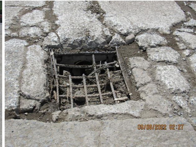
IMG 480 -Close-up of the stormwater catch basin partially clogged with sediment from upstream. The inlet of the catch basin is not protected.
