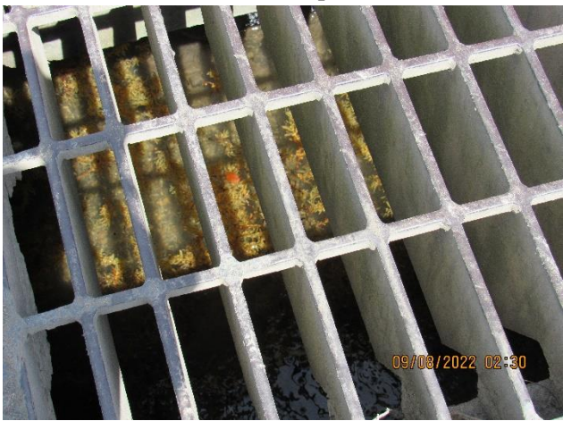
IMG 484 -Close-up view of stormwater catch basin with raised inlet. Observed sea water intrusion with large amount of marine vegetation inside catch basin.
