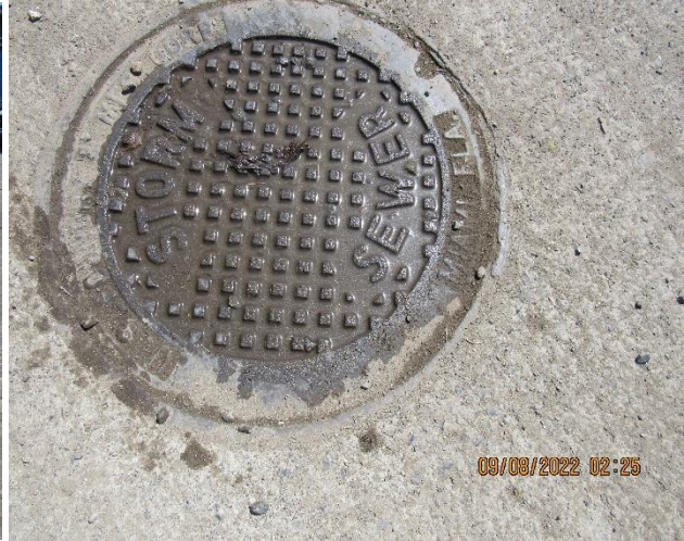
IMG 478 -Picture of cover to storm sewer that conveys stormwater from upstream area.
