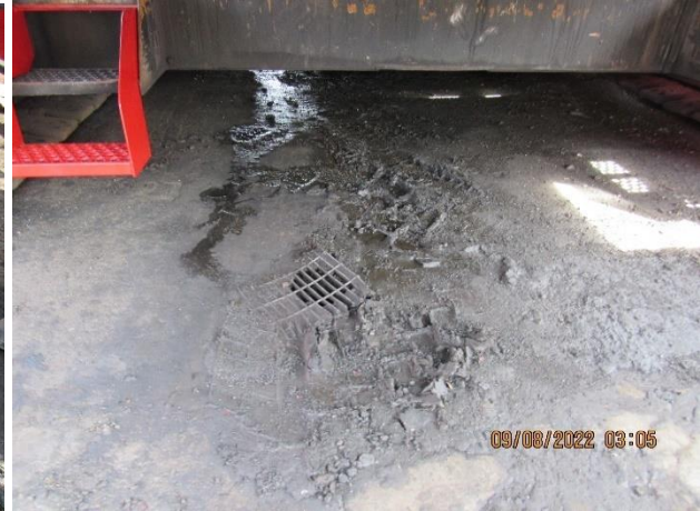
IMG 514 -View of the inlet submerged in oily-mud. Oily-water runoff and sediment entering the Oil/Separator unit. Did not identify discharge port.
