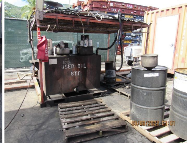
IMG 510 -Use Oil management tank not within containment to capture used oil spills and prevent releases that are exposed to stormwater runoff flow.
