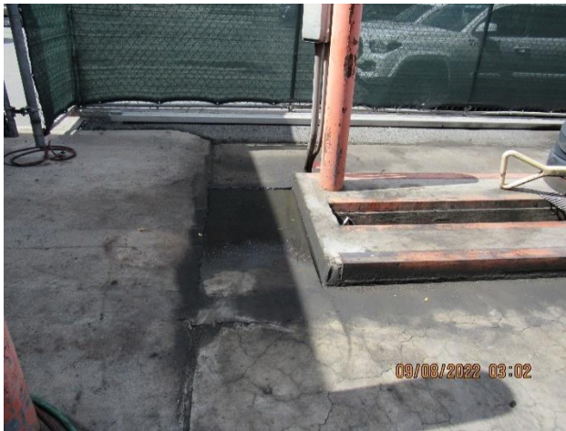
IMG 511 -Evidence of spilled used oil on platform washed-off by stormwater runoff flow away from the used oil storage system.
