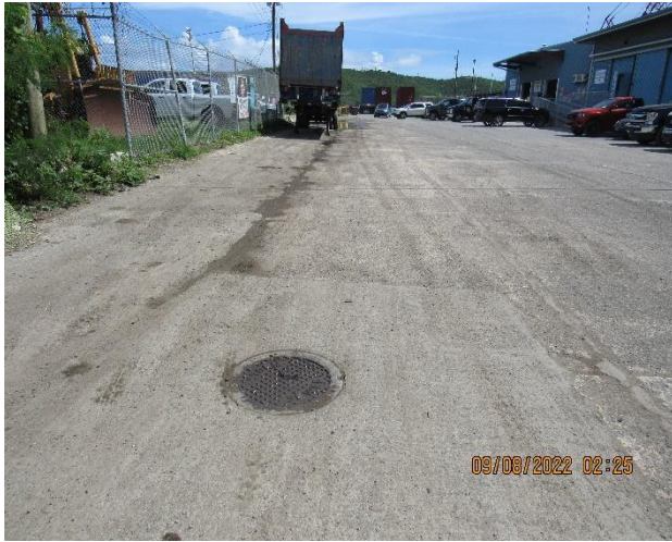
IMG 477 -Road going into the dock area. Sediment transported by storm water runoff from Field seen in the stormwater flow path along the road.
