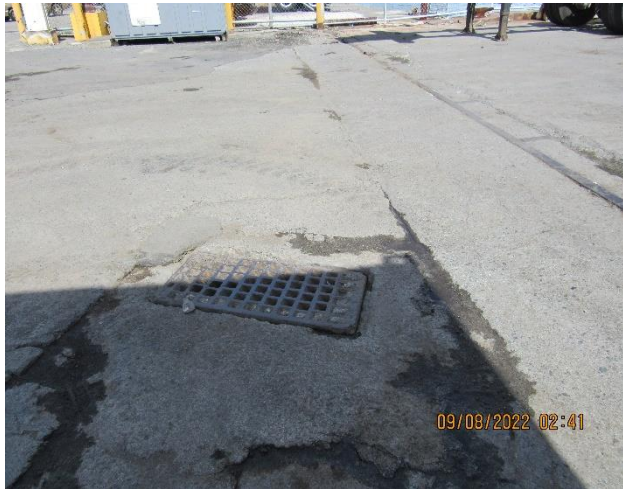
IMG 486- A storm water catch basin within the fence line. The inlet of the catch basin is not protected.
