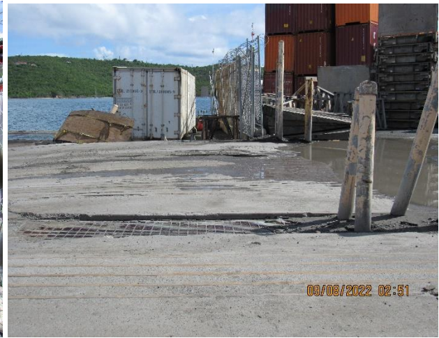
IMG 500 -Large catch basin in which mid-section of the Facility through which stormwater enters the large drainage canal, and into the Bay.
