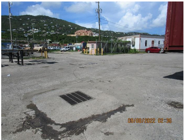
IMG 485 -Stormwater catch basin with raised inlet just in front of Tropical's fenced dock area. The inlet of the catch basin is not protected.
