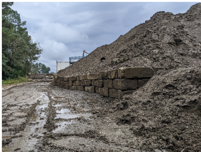
Figure 98: PXL_20211006_181114686.jpg – Rear side of solid waste pile near Outfall 3
