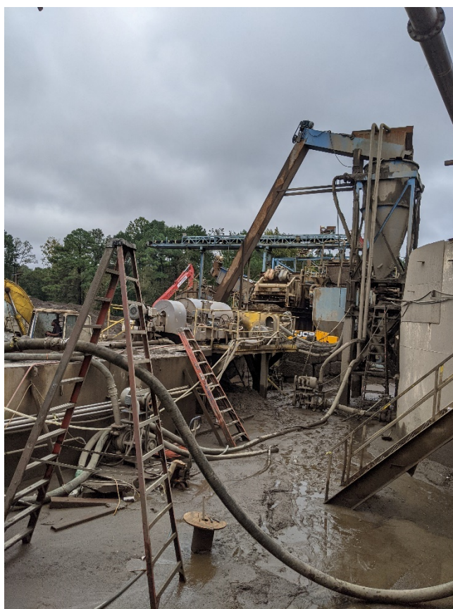
Figure 72: PXL_20211006_151016463.jpg - Wastewater Treatment Area
