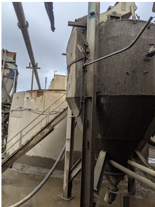
Figure 75: PXL_20211006_151034451.MP.jpg – Wastewater Treatment Area Tanks
