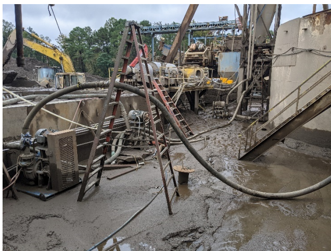
Figure 74: PXL_20211006_151028251.jpg – Wastewater Treatment Area
