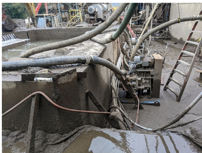
Figure 67: PXL_20211006_150035330.jpg – Wastewater treatment area
