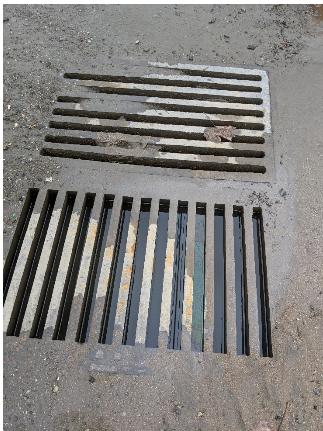
Figure 83: PXL_20211006_151632795.jpg – Plugged up Stormwater drain
