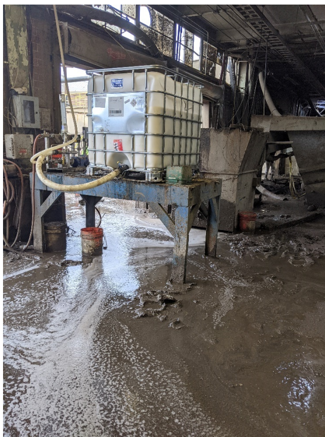
Figure 64: PXL_20211006_145902126.jpg – Sludge flowing across the floor.
