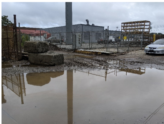
Figure 81: PXL_20211006_151548117.jpg – Plugged up Stormwater drain
