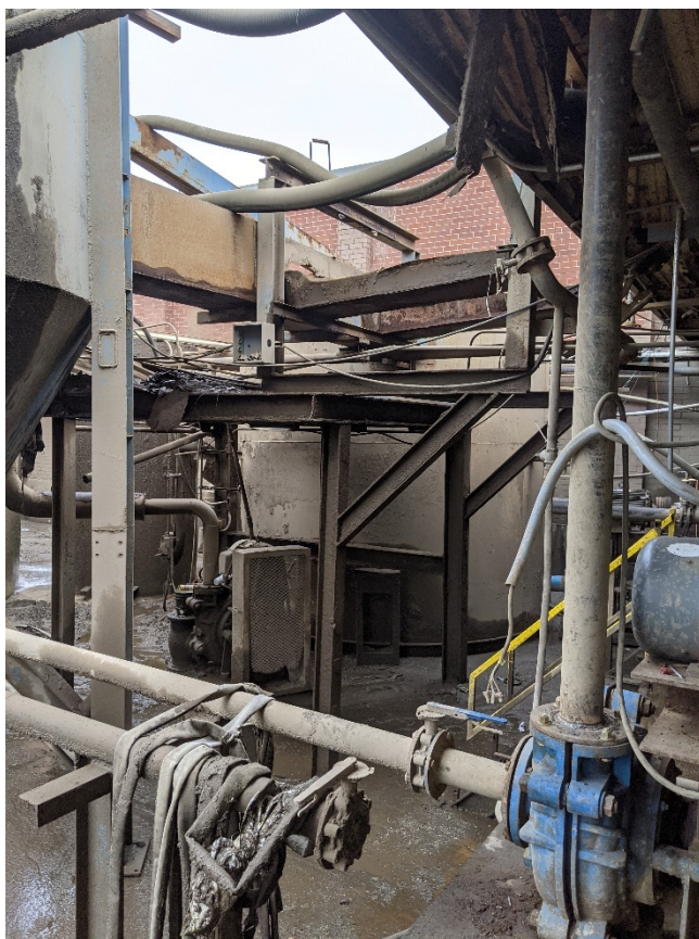
Figure 76: PXL_20211006_151038425.jpg – Wastewater Treatment Area
