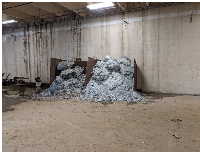
Figure 94: PXL_20211006_180547574.jpg – Partially melted aluminum in the Basement
