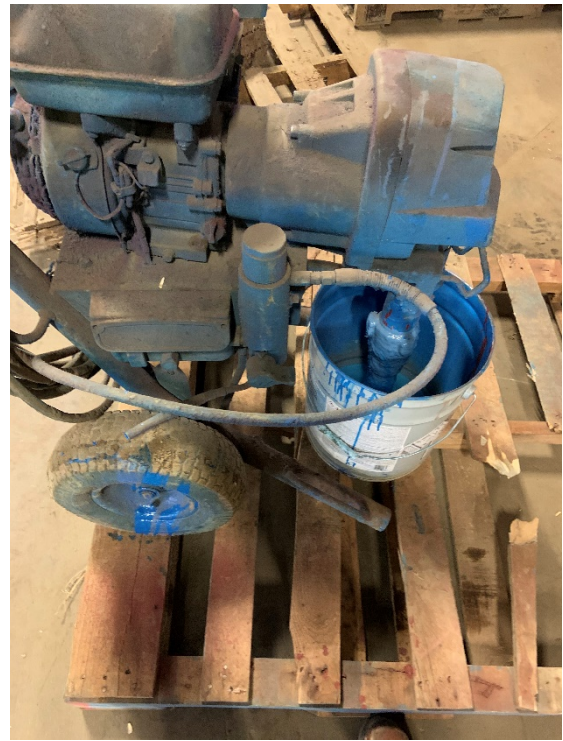
Figure 6: IMG_3075.jpg – Paint sprayer in the Fabrication Building
