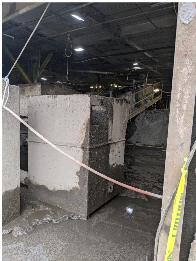
Figure 65: PXL_20211006_145919867.jpg – Tank receiving process wastewater and sludge/wastewater overflow on the floor
