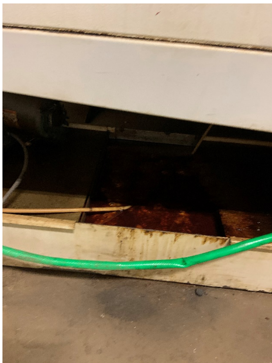
Figure 3: IMG_3072.jpg – oil under the CNC machine in the Shipping Building
