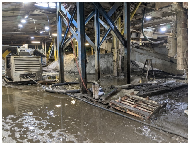
Figure 80: PXL_20211006_151153926.jpg – Wastewater Treatment Area
