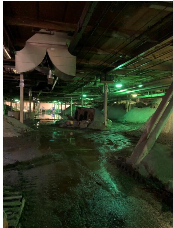
Figure 34: IMG_3103.jpg – Piles of solid waste stored in the Keebler Building
