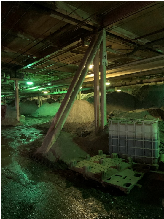
Figure 33: IMG_3102.jpg – Containers of unknown waste and pile of solid waste in the Keebler Building
