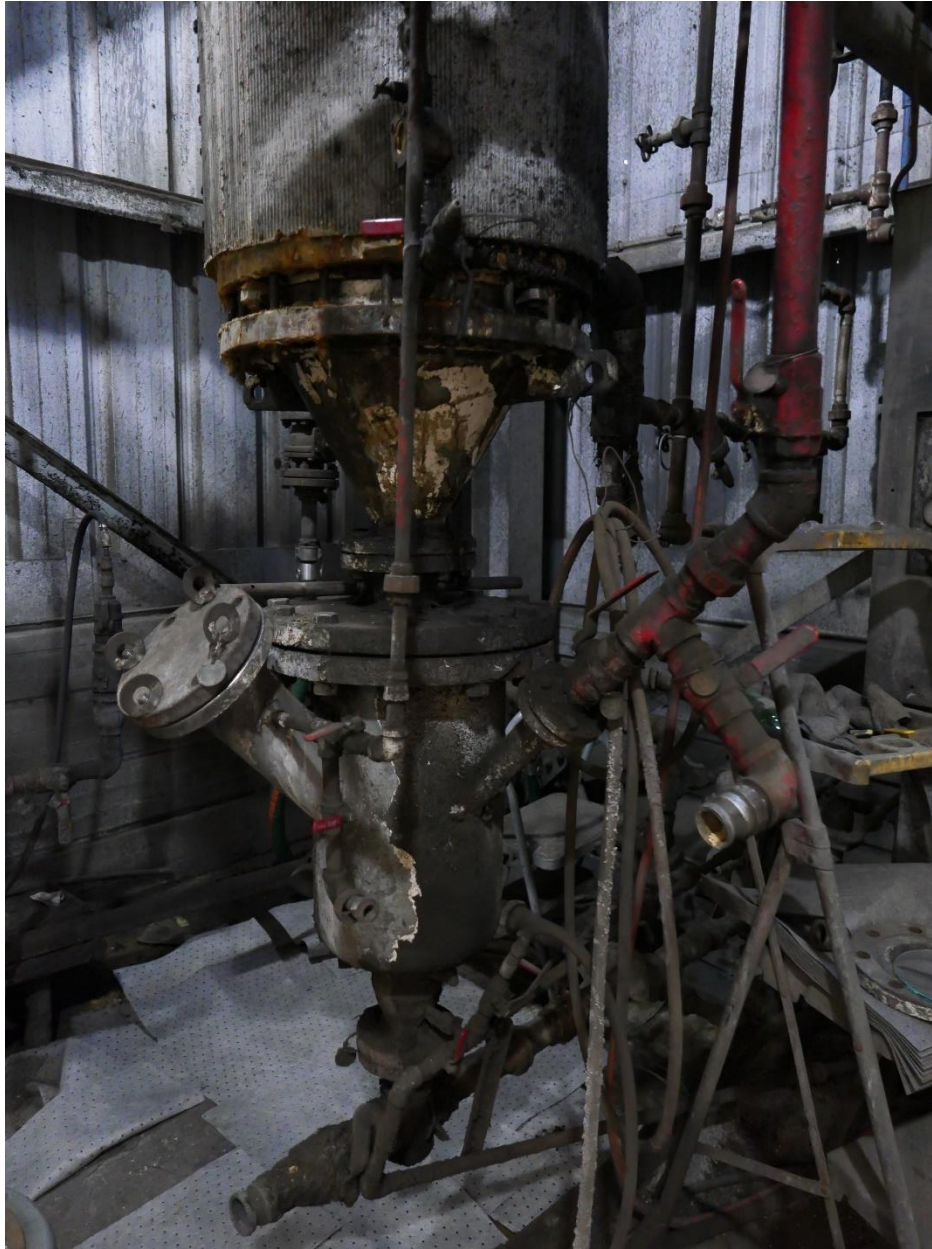
Photo 8: Luwa® Solvent Recovery Unit illegible tags for equipment.
