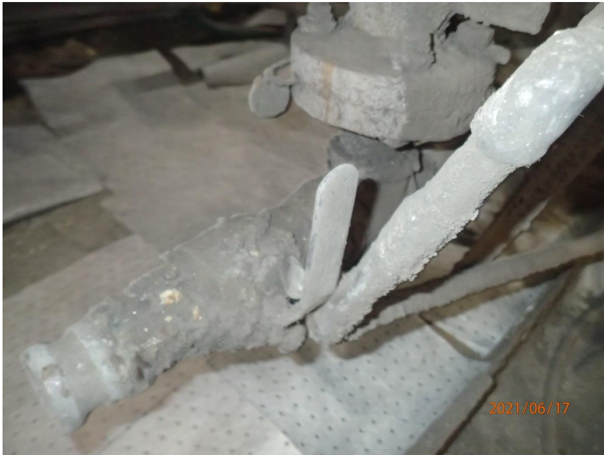
Photo 7: Luwa® Solvent Recovery Unit illegible tags for equipment.
