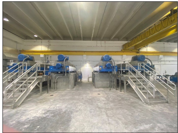
Photo 12: New sludge dewatering centrifuges.
