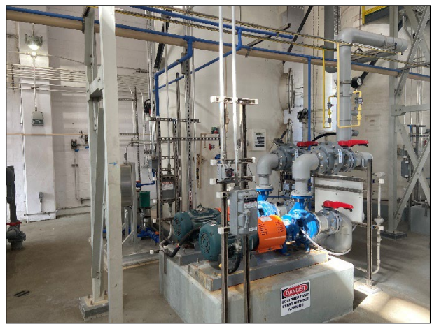
Photo 8: Plant 2 odor control scrubbers.
