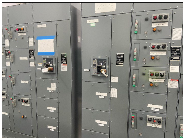
Photo 2: New electrical building equipment.
