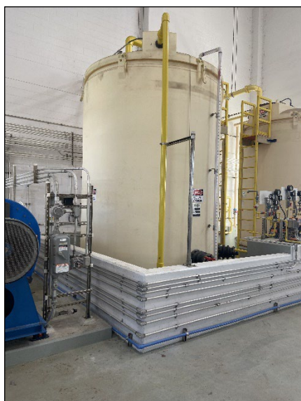
Photo 3: Plant 1 odor control scrubbers.
