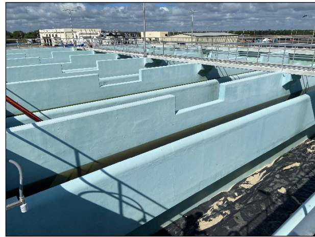
Photo 10: New deep-bed sand filters.
