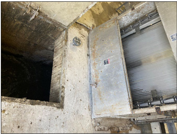
Photo 7: Plant 2 influent bar screens.
