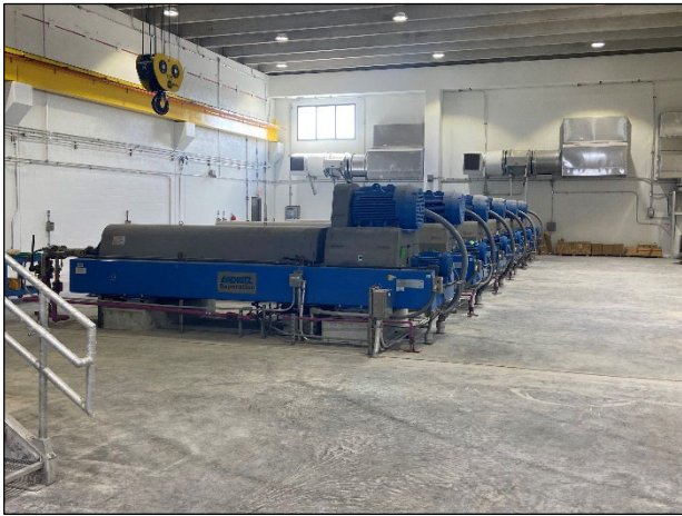
Photo 11: New sludge thickening centrifuges.
