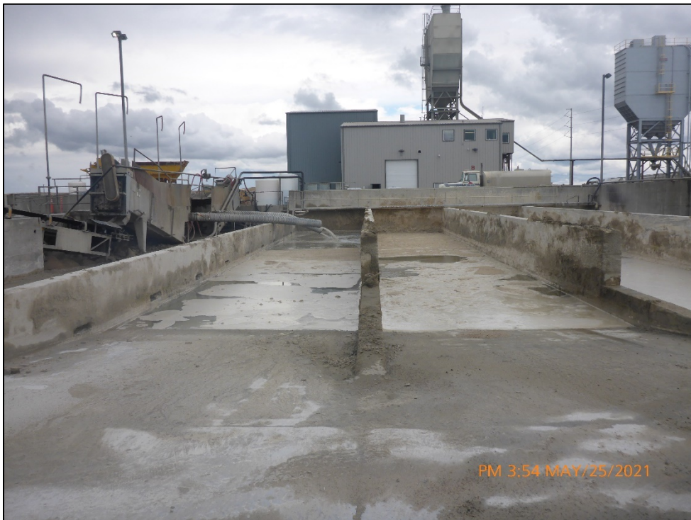
Photograph 18. View of the wash water recycling system, which was operational at the time of the inspection.
