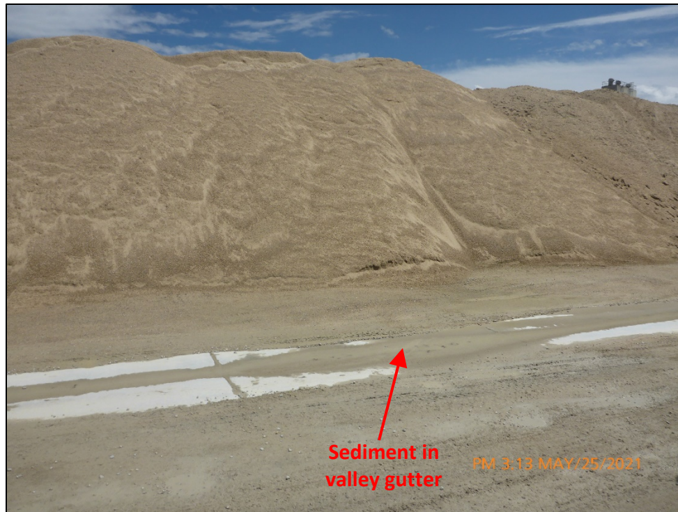
Photograph 13. View, facing east, of sediment in the valley gutter adjacent to the aggregate stockpiles shown in Photograph 12. Control measures were not in place to prevent sediment from the aggregate stockpiles from entering this valley gutter.
