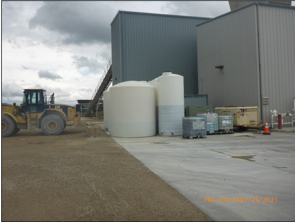
Photograph 17. View, facing north, of the bulk chemical storage area at the batch plant. This chemical storage area is not identified on the SWPPP site map.
