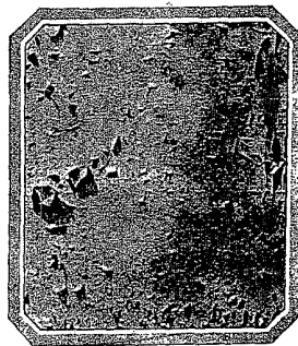
This paint film lost its contact with the metal. It scaled off in patches... left the metal unprotected against corrosion. The paint did not retain its adherence.
