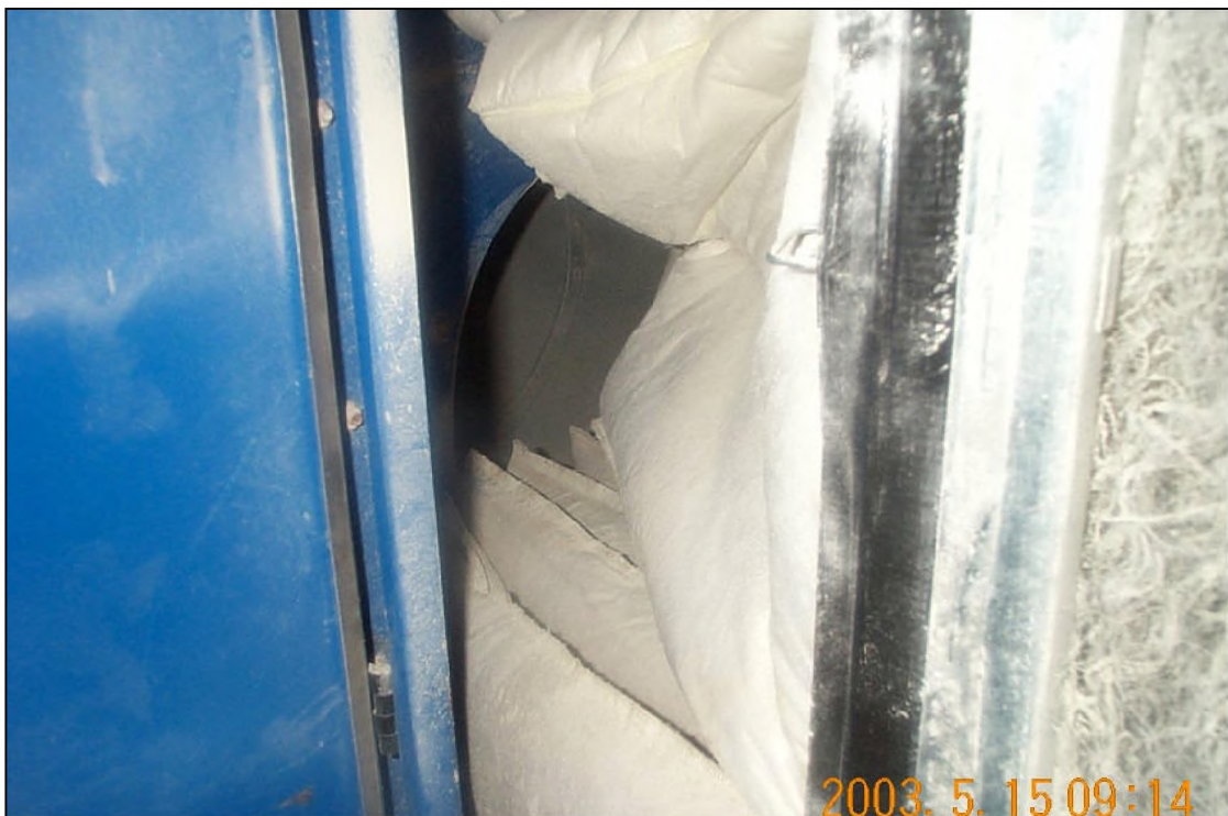
AirCure Secondary Filter – 9 days after installation Filter collapsing due to inadequate chamber space available
