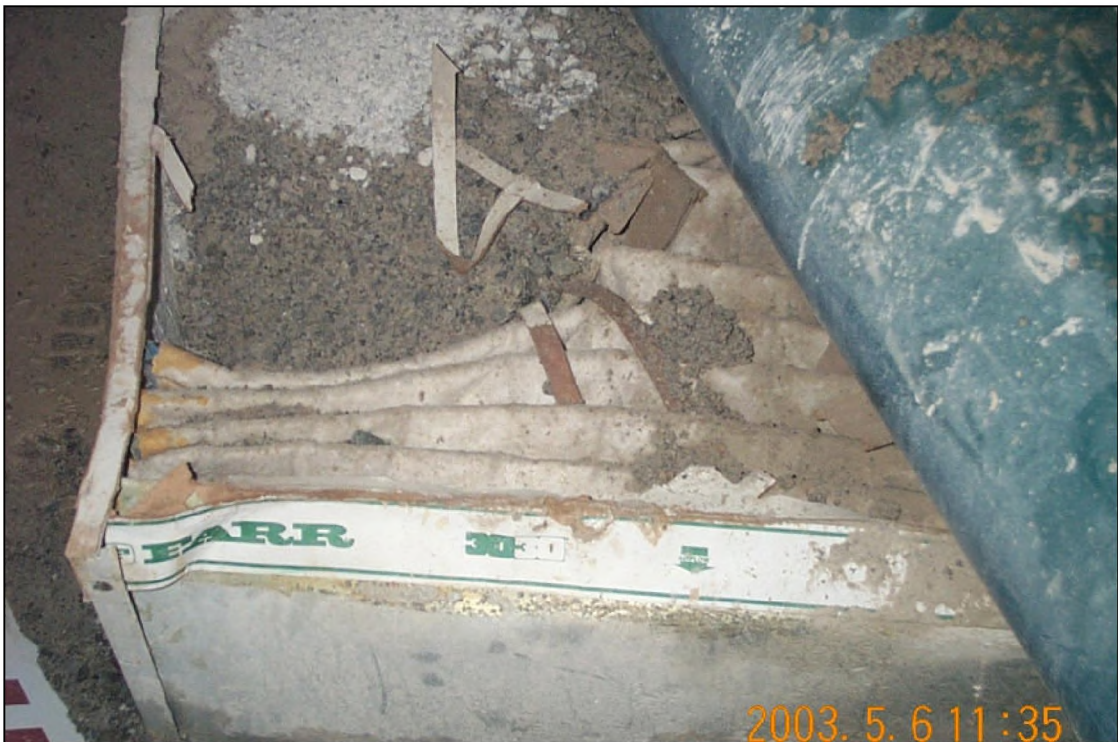
Condition of Dynavane Secondary Filter – X days after installation
