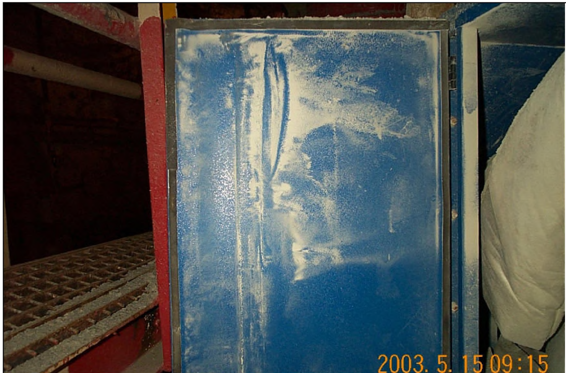
Blow marks (leakage) on access door due to incorrect door design
