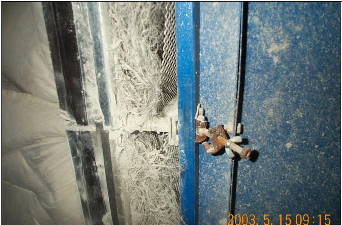
AirCure Primary Filter –9 Days after installation. Improved holding frame required
